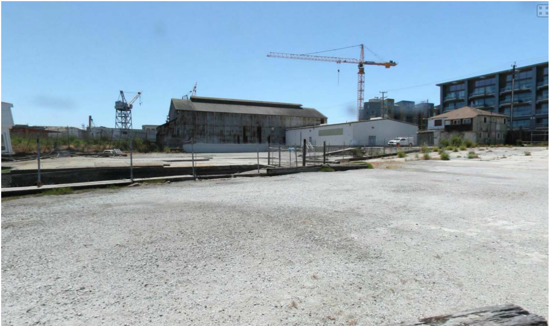
view of un-engineered fill looking south
