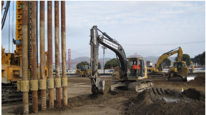
A landside buttress to stabilize the shoreline would be accomplished by deep mixing of in situ soils with cement as shown here - San Francisco, CA © Fugro
