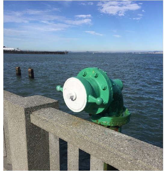
Suction connection for emergency firefighting, Rincon Park
