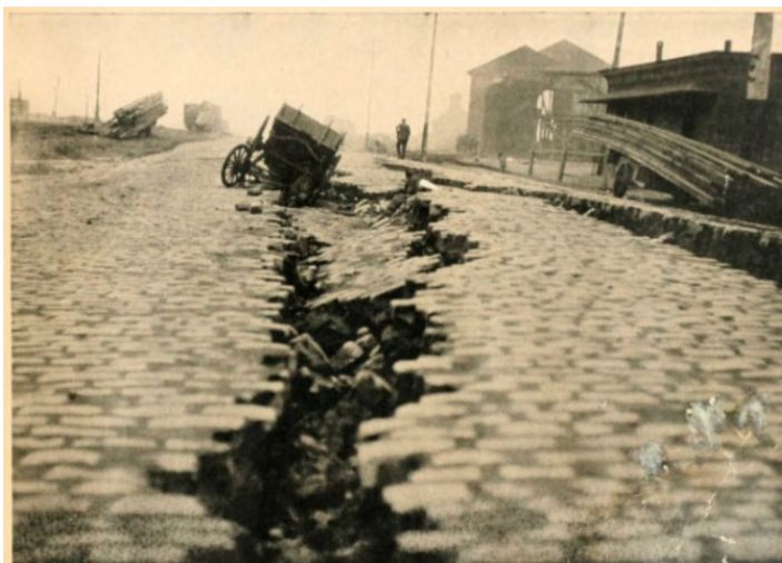
Figure 3-5. Damage from Lateral Spreading at the Foot of Lombard Street after the 1906 Earthquake
