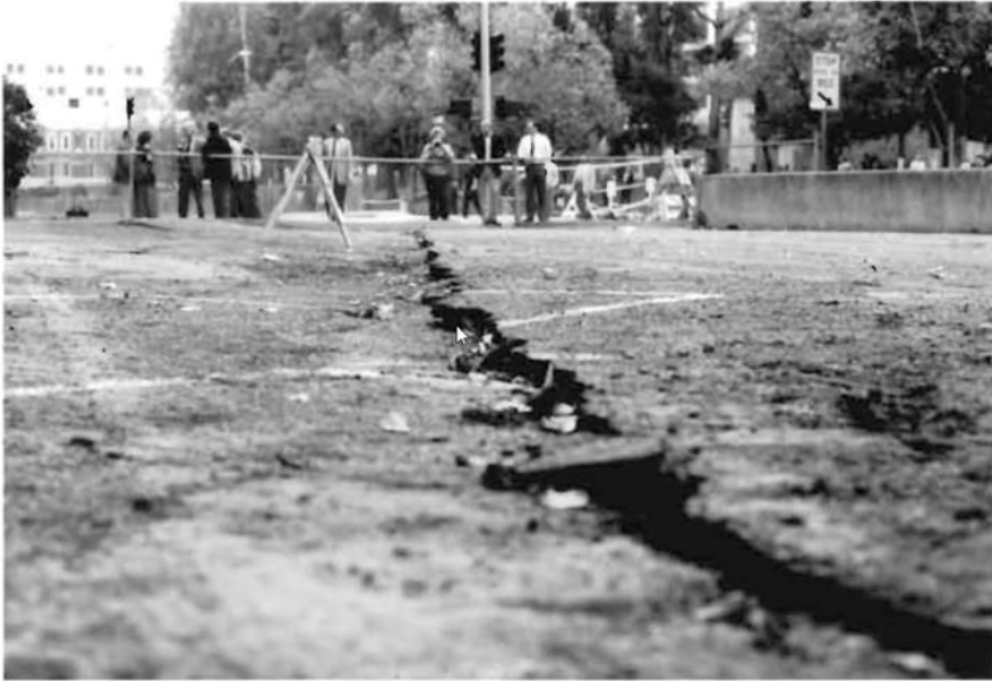
Figure 3-6. Differential Settlement on the Embarcadero Near the Intersection of Market Street in 1989
