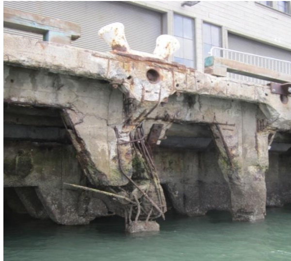
Figure 4: Pier 35 apron—scheduled for repair by the Port's new cement pile repair crew
