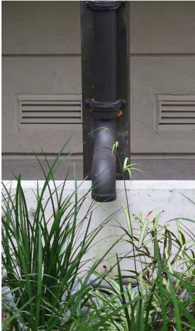
A disconnected roof downspout spills into a bioretention planter. Photo: Krystal Zamora
