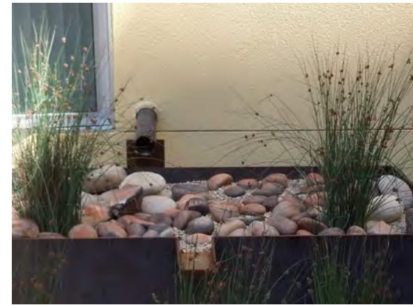
An interior roof drain discharges to a courtyard bioretention planter in San Francisco, CA. This properly designed and permitted stormwater facility is an example of an “approved alternate location” for stormwater discharge. Photo: Polly Perkins
