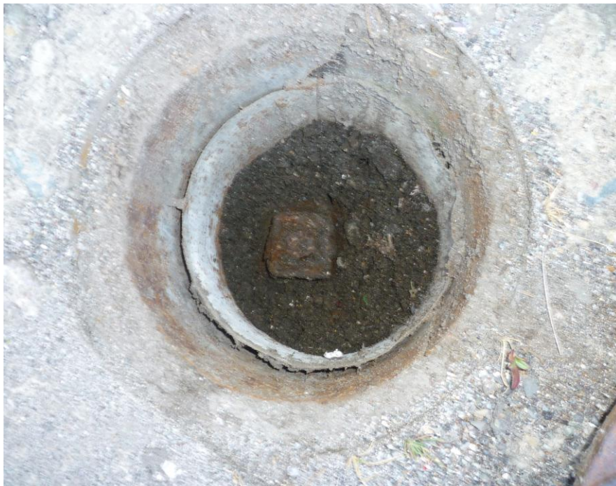
Photograph 2 – Circular metal vault with lid and square cap- located in driveway east of Building 14
