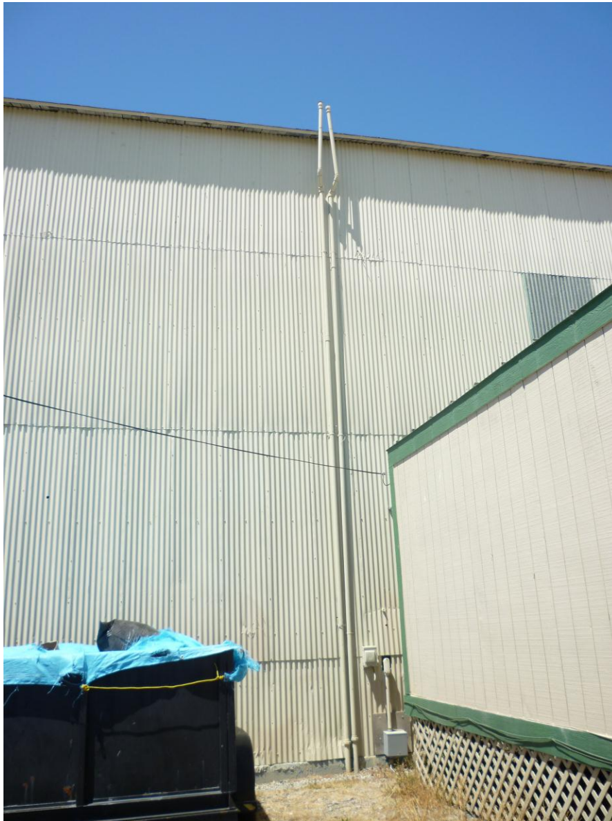
Photograph 3 - Two vertical vent pipes on south wall of Building 49
