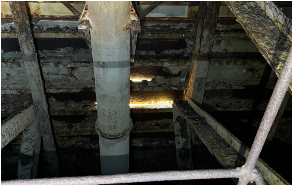
Photograph 12 - Internal view of Tank 12 side shell tear
