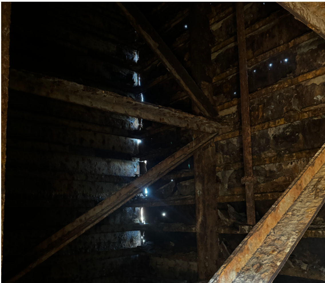
Photograph 34 - Internal view of vertical wing shell tear at Tank 29
