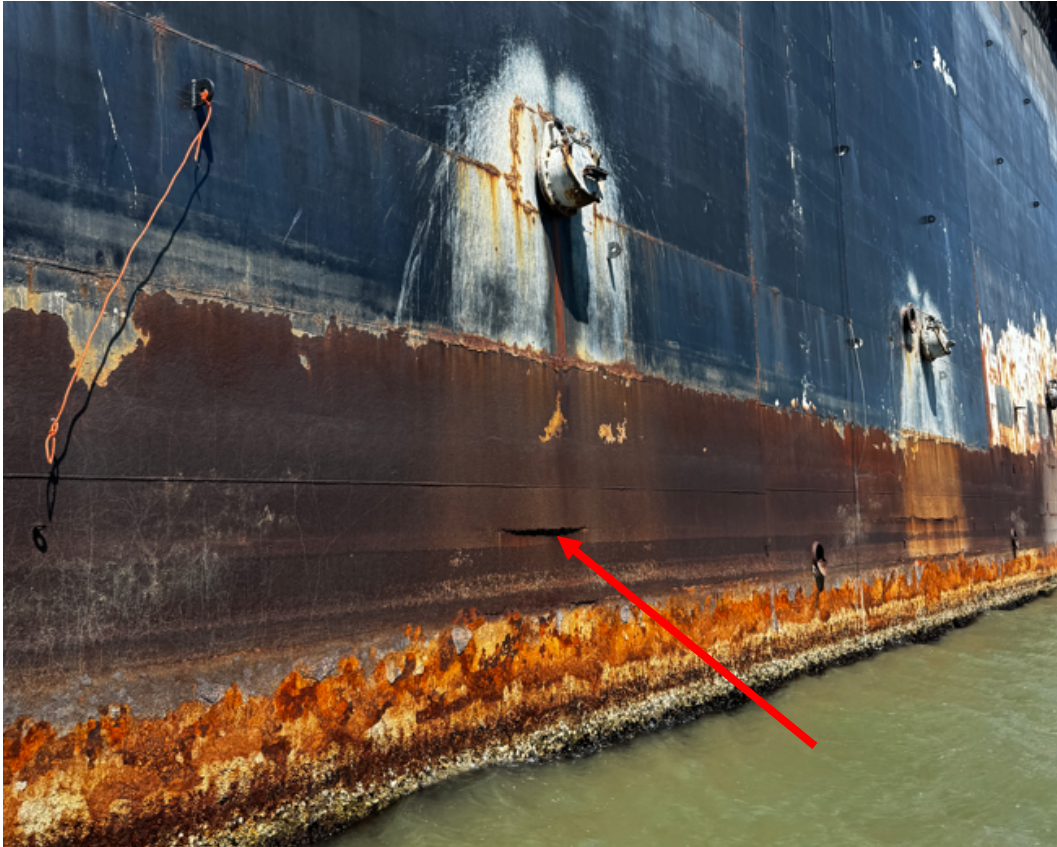
Photograph 11 - External view of Tank 12 side shell tear below discharge
