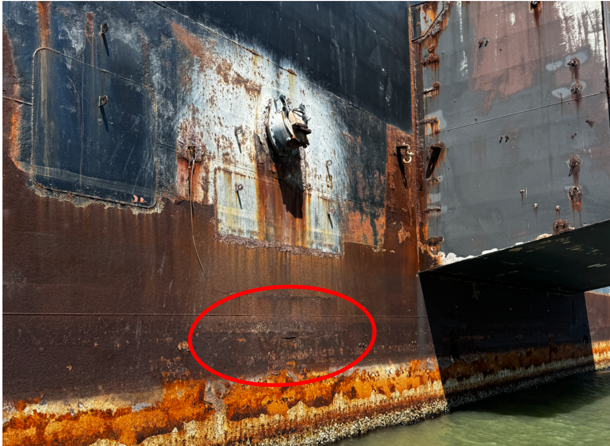
Photograph 5 - Corrosion around Tank 4 discharge penetration with side shell tear below
