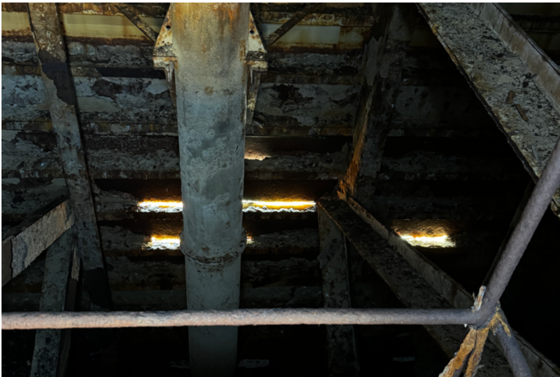
Photograph 23 - Internal View of side shell tears at Tank 30
