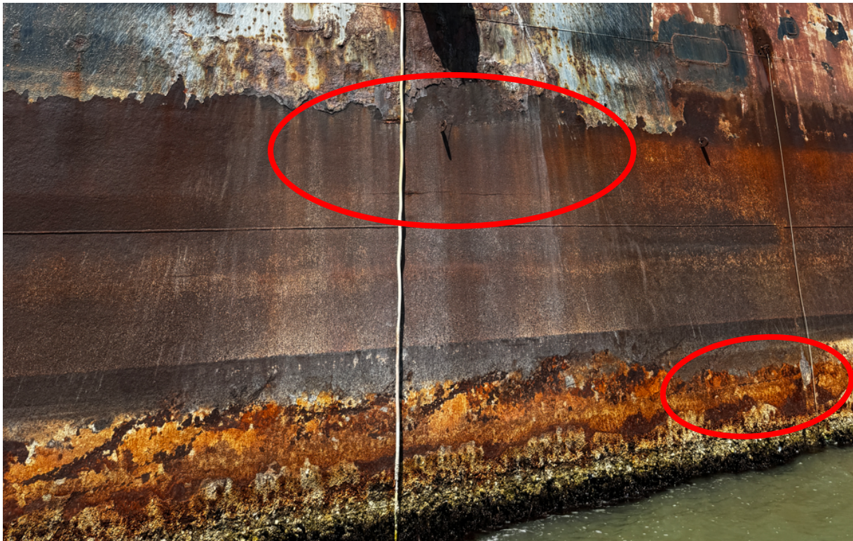
Photograph 19 - External view of Tank 22 side shell tears
