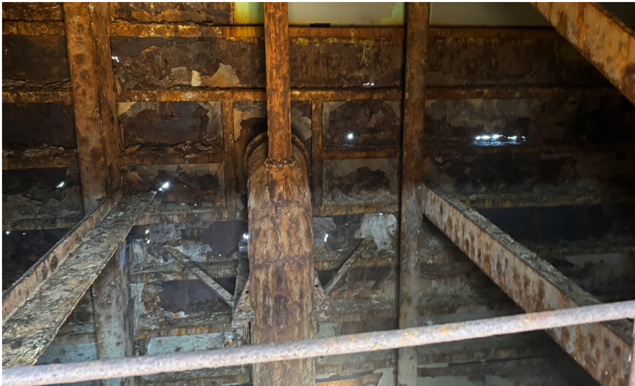
Photograph 32 - Internal view of side shell tears at Tank 29
