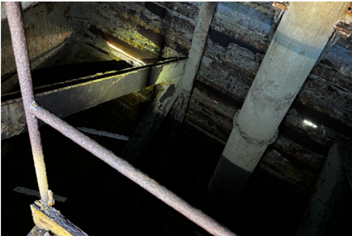
Photograph 20 - Internal view of Tank 20 side shell tears
