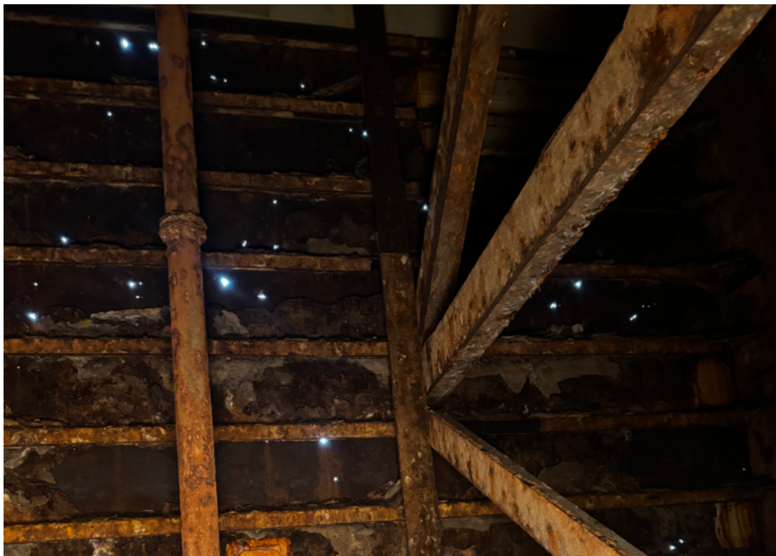
Photograph 30 - Holed through wing shell at Tank 25
