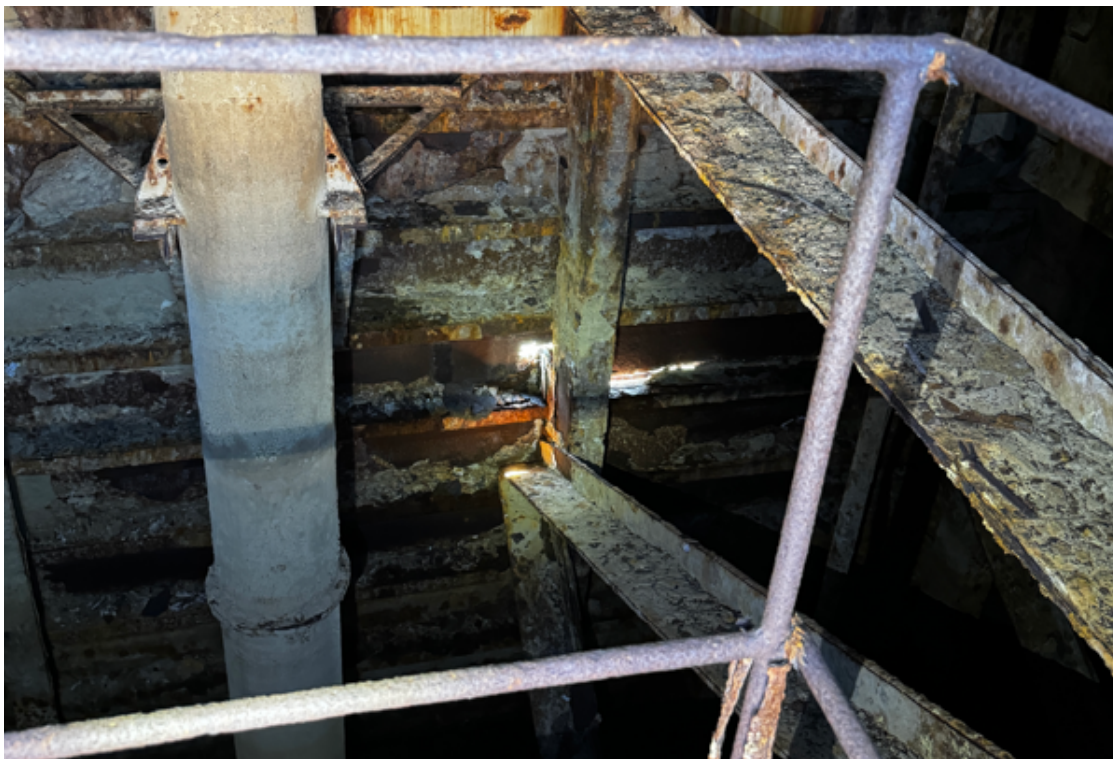
Photograph 16 - Internal View of Tank 16 side shell tear
