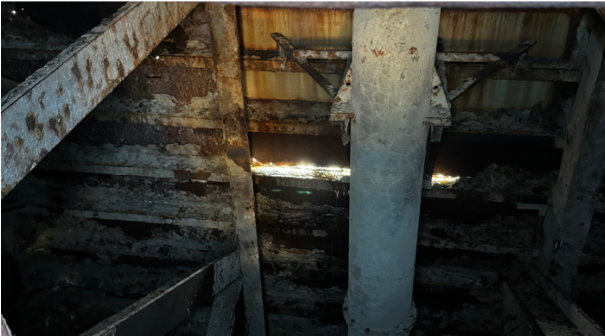
Photograph 6 - Internal view of Tank 4 side shell tear
