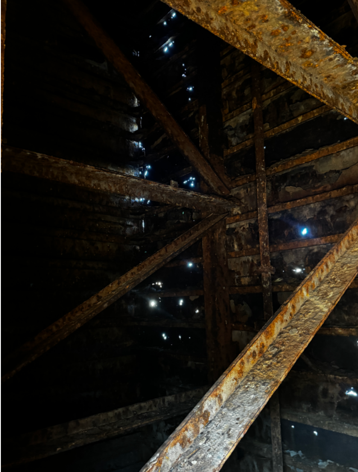
Photograph 26 - Vertical tear of wing shell at FR 26 (Tank 13)
