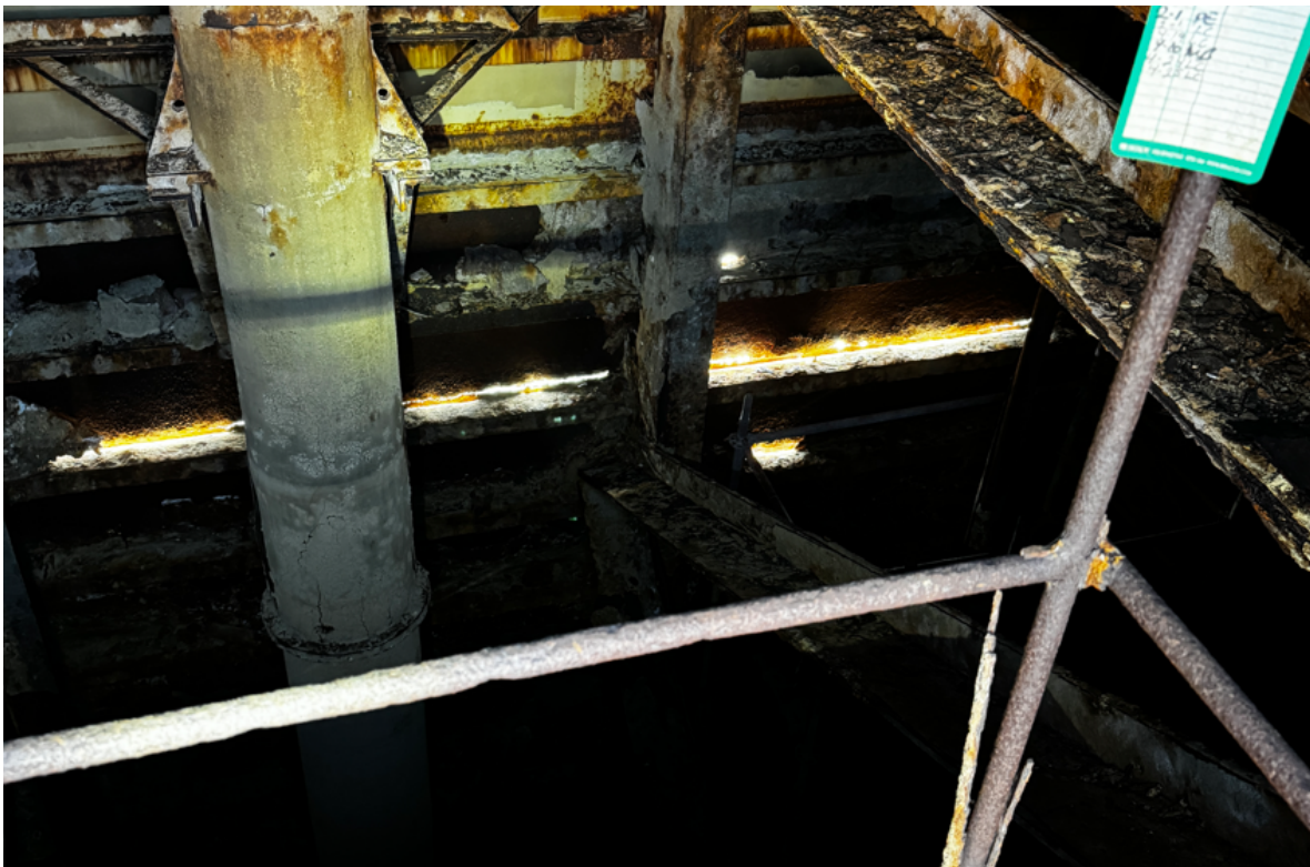
Photograph 14 - Internal view of Tank 14 side shell tear
