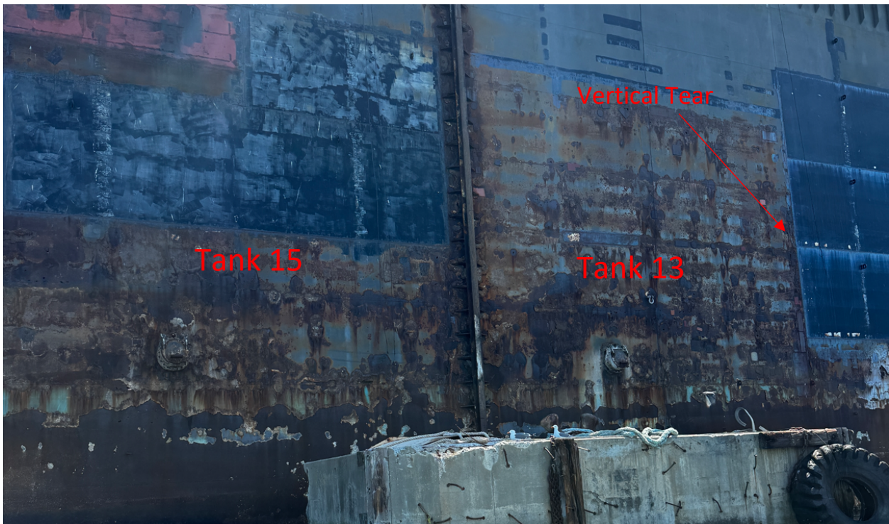
Photograph 25 - External view of corroded wing shell plating in way of Tank 13 and 15
