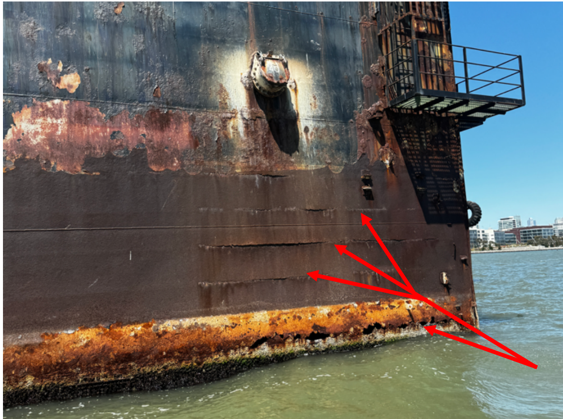
Photograph 1 - Outboard Shell tears just above waterline in NE corner of dock (Tank 40)
