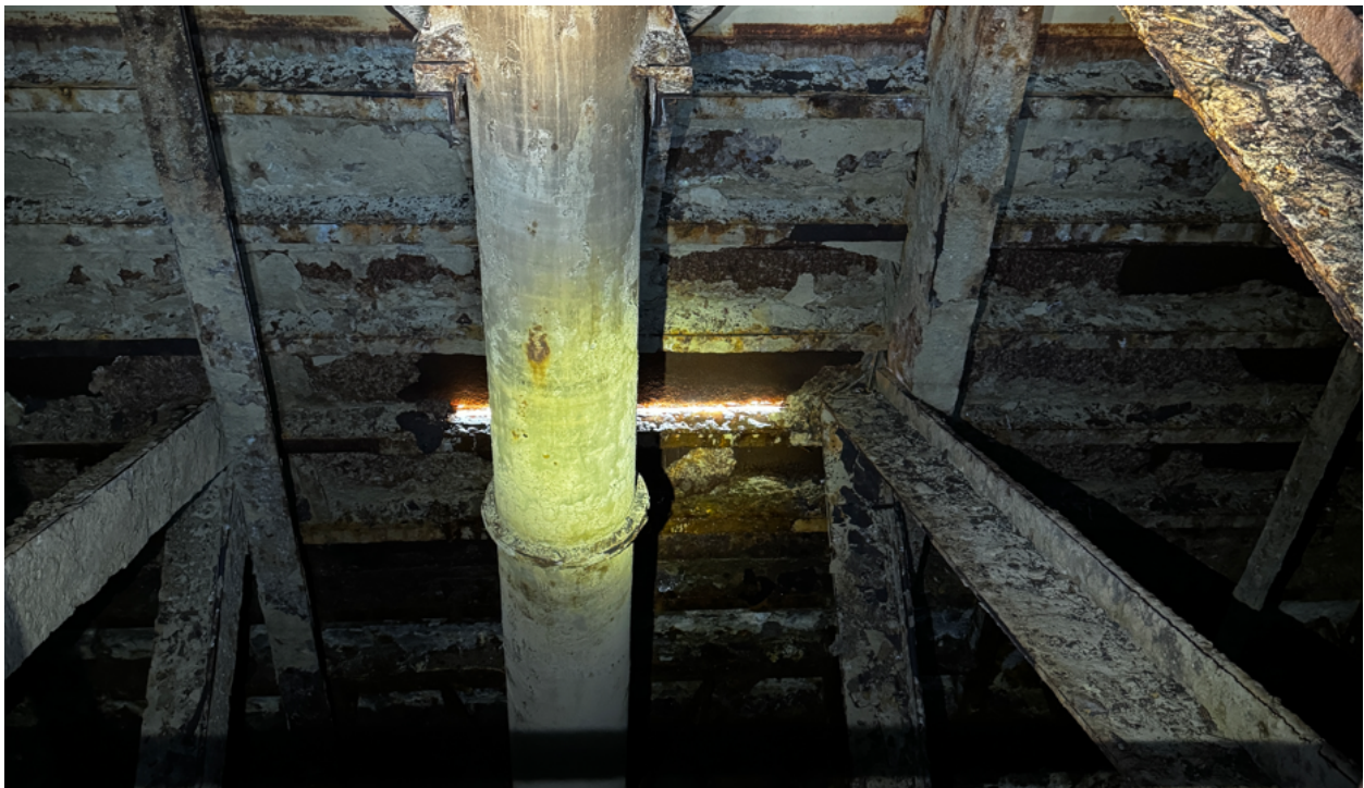
Photograph 10 - internal view of Tank 10 side shell tear
