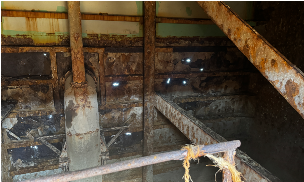
Photograph 28 - Internal view of through side shell plating in way of Tank 17 discharge
