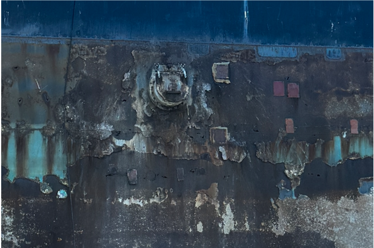
Photograph 27 - External view of through side shell plating in way of Tank 17 discharge
