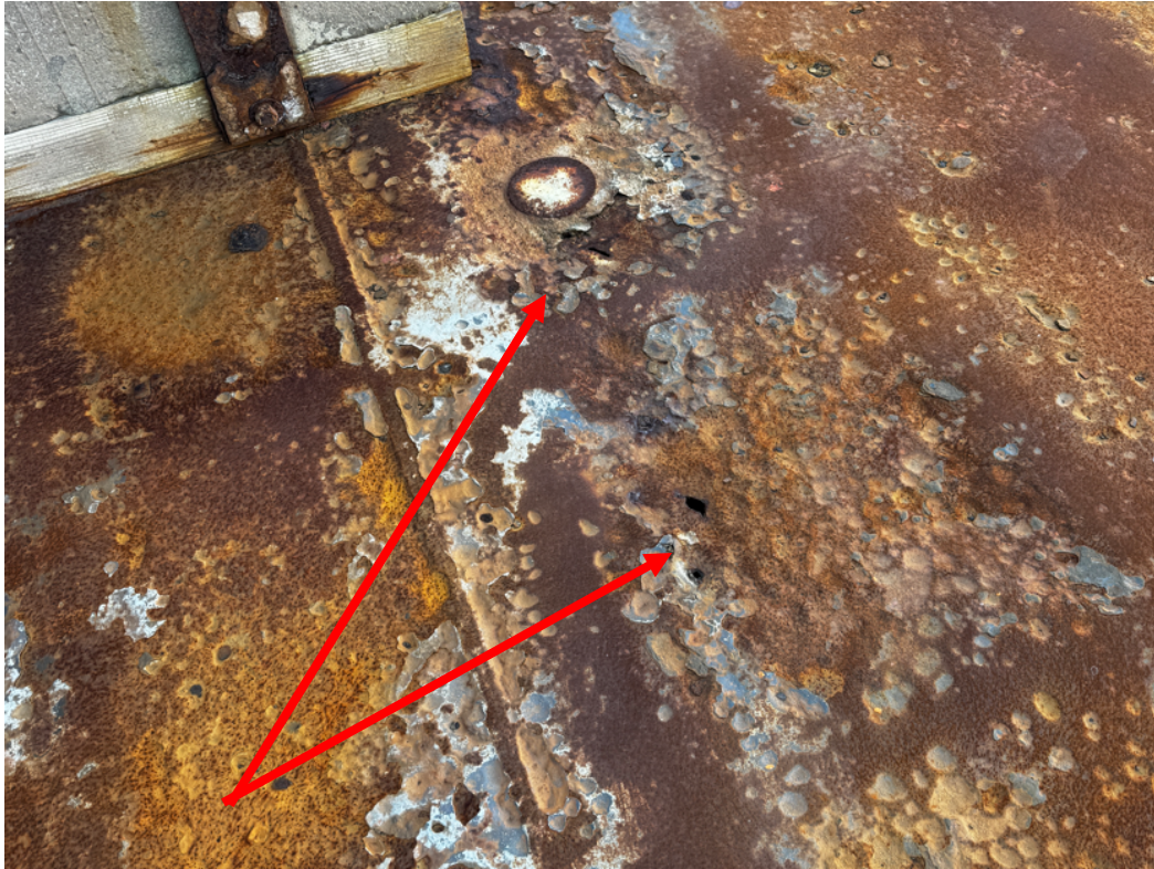
Photograph 37 - Typical condition of pontoon deck in way of holed through areas
