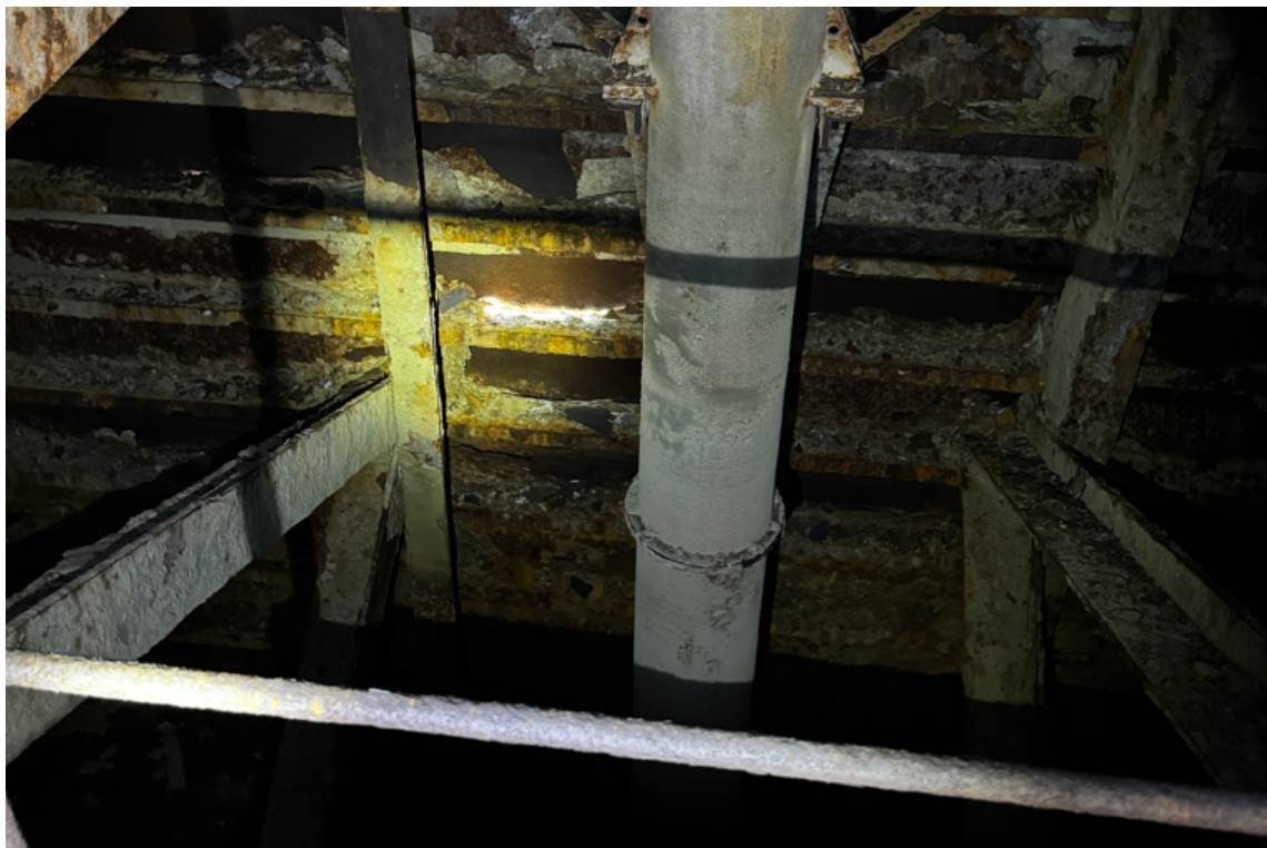
Photograph 18 - Internal view of Tank 18 side shell tear
