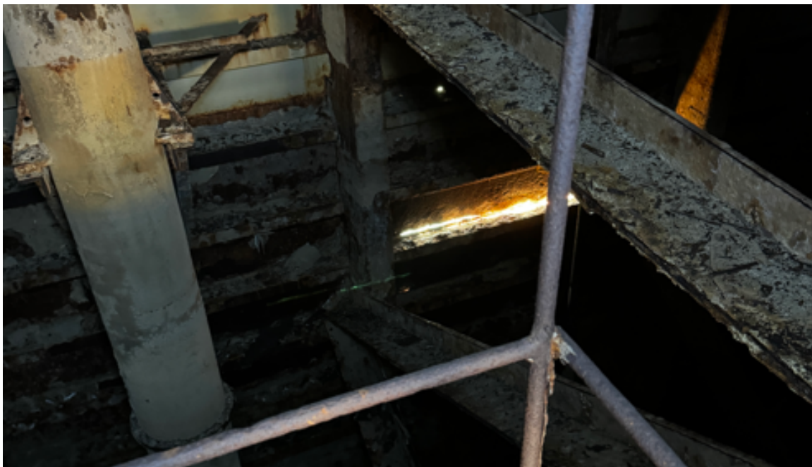
Photograph 8 - Internal view of side shell tear at Tank 8
