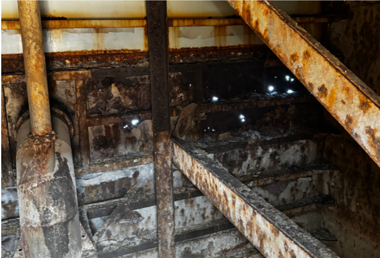
Photograph 24 - Holed through side shell plating at Tank 11
