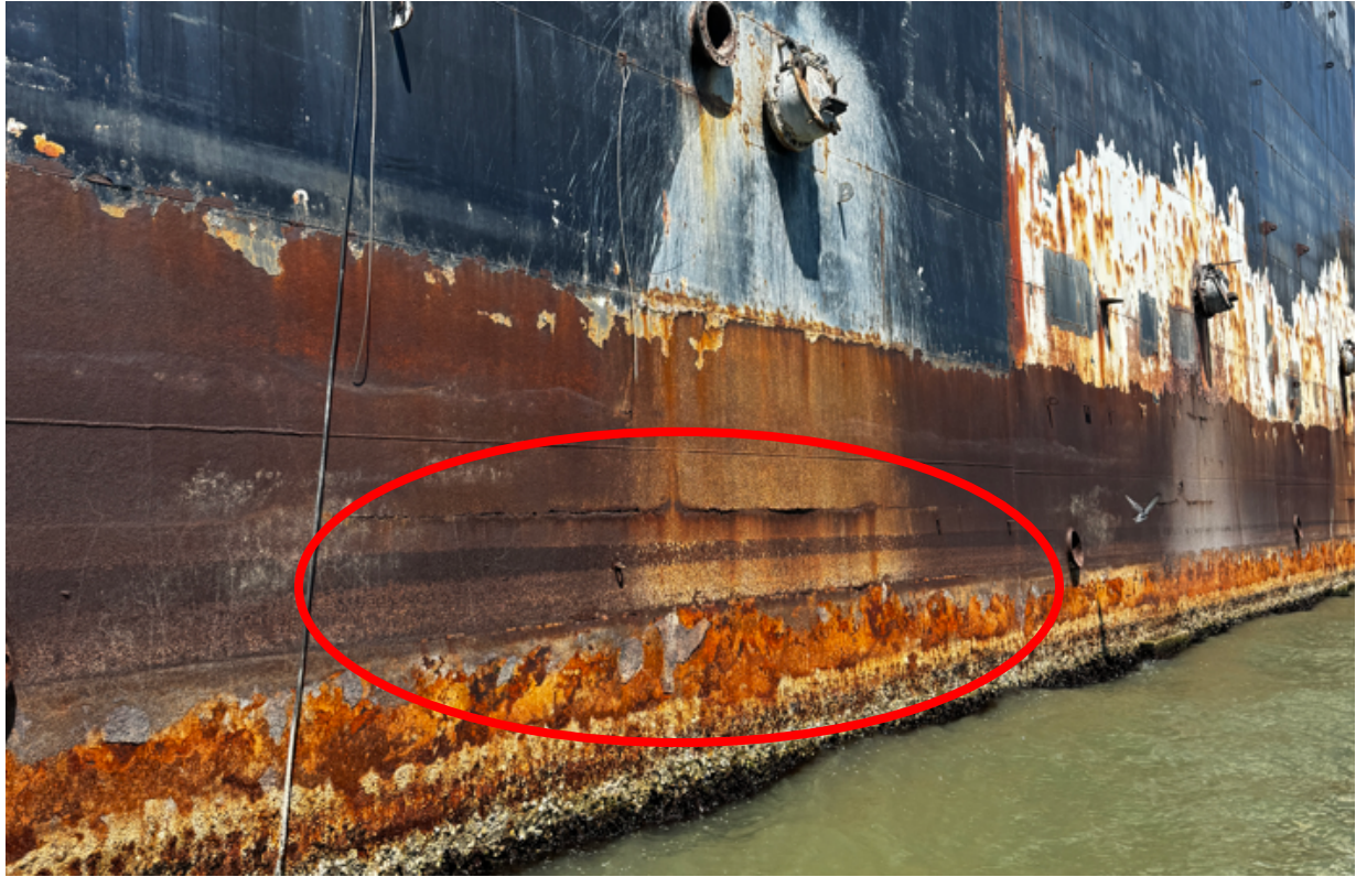
Photograph 13 - External view of Tank 14 side shell tear
