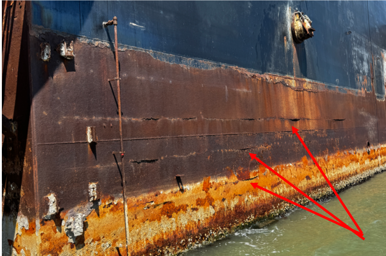
Photograph 3 - Outboard Shell tears at SE corner of dock (Tank 2)
