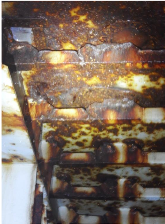
Photo 1: Multiple stiffeners in “severe condition” (as referenced in Appendix F Material Condition Survey Deficiencies ).
