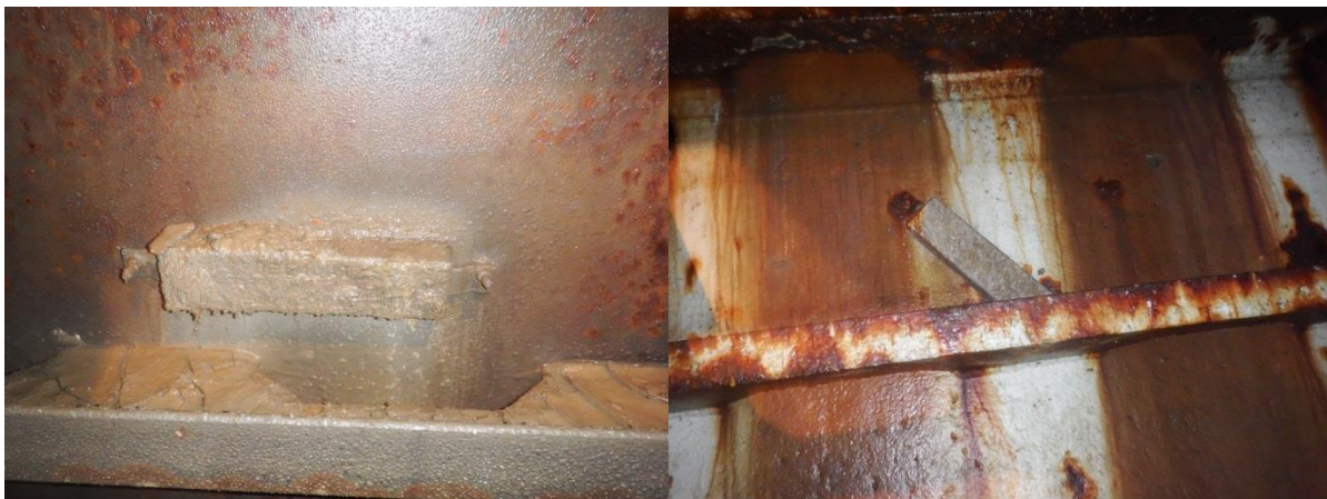
Photos 4 and 5: Typical condition of zinc anodes throughout the dock.
