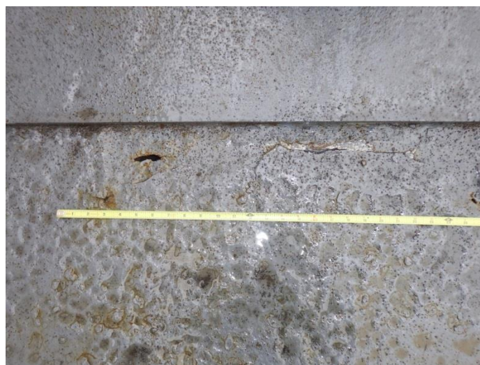
Photo 6: Tension crack over tank 9.
