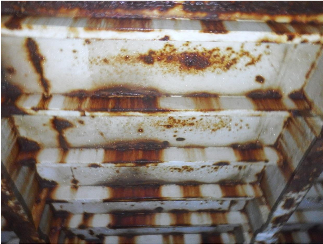
Photo 5: Typical condition of solid stiffeners. Notice skip welding and corrosion at unwelded contact between the stiffener and pontoon deck.
