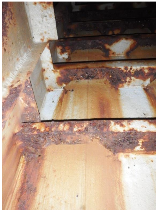
Photo 2: Typical notched condition of a stiffener.
