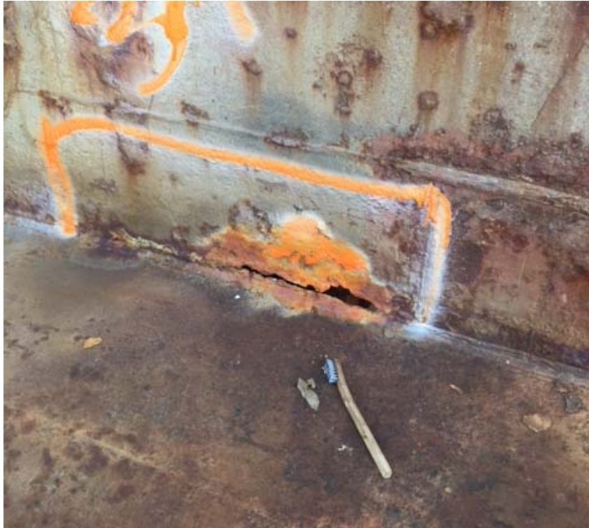
Photo 3: Inboard wing shell has become disconnected from Pontoon Deck in numerous places along the docks length on the East and West wings. Above picture shows a typical corrosion hole along the weld seam of the pontoon deck and inboard wing shell.
