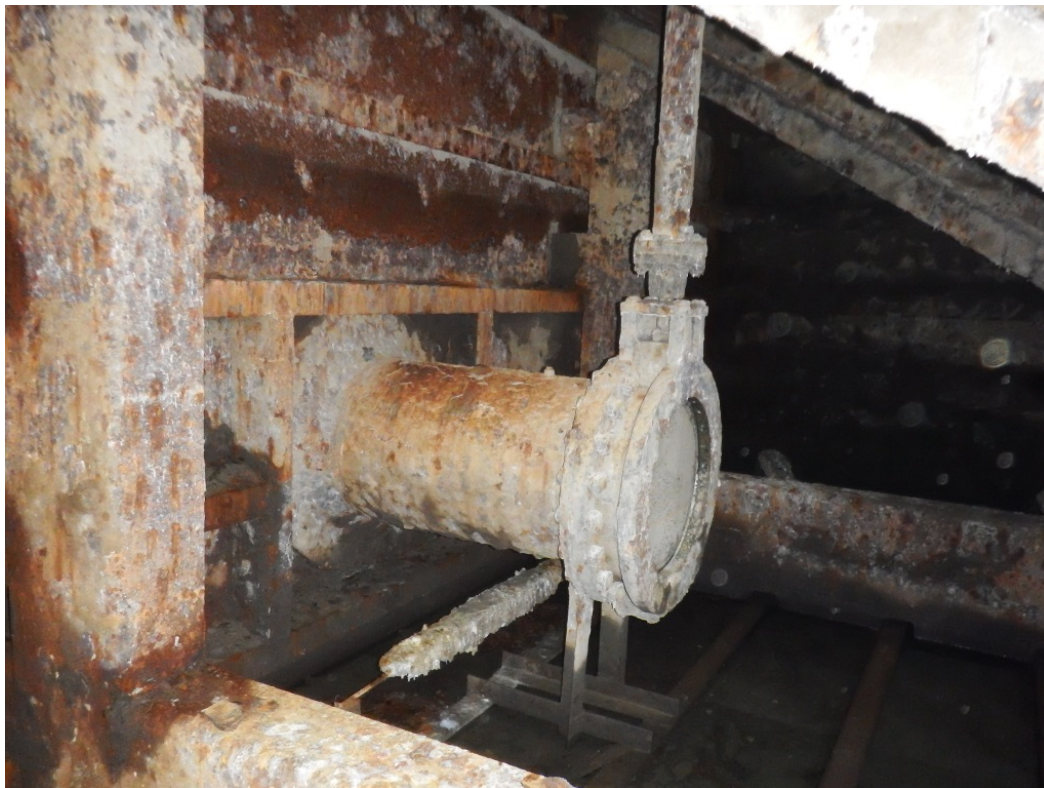
Photo 8: Typical flood valve.
