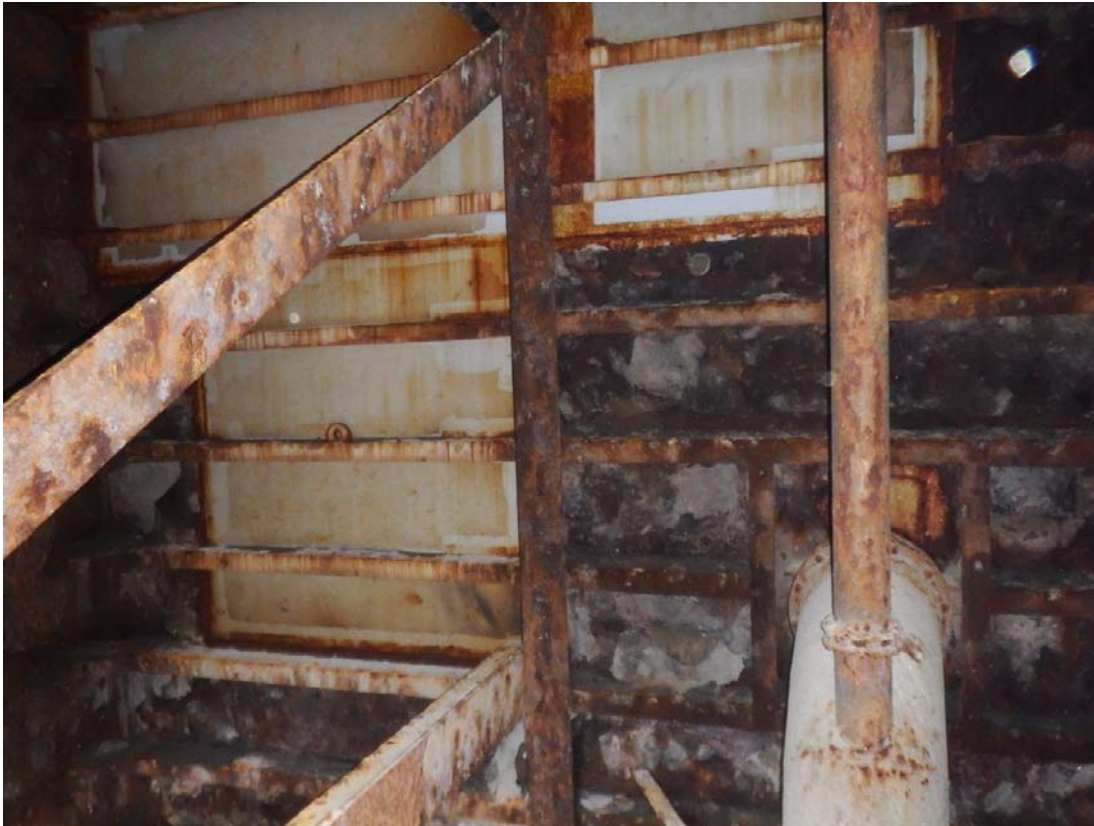
Photo 16: Internal outboard wing structure in way of renovated panel. The renovated panel is in good structural condition with paint 75% intact. Surrounding original plate is heavily scaled with no protective system.
