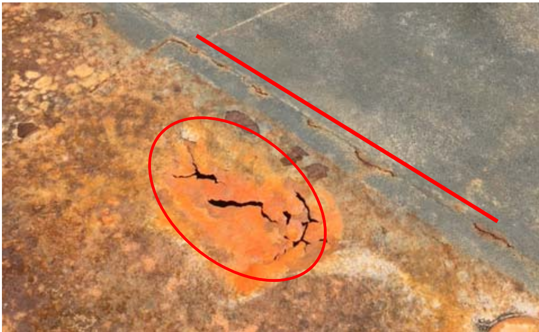
Photo 2: Pontoon deck hole circled in red. Pontoon deck crack along transverse frame 21 outlined in red. Similar failure mode located along first longitudinal stiffener inboard of West wing between frames 6 & 7, 75 & 76, and 78 & 79.
