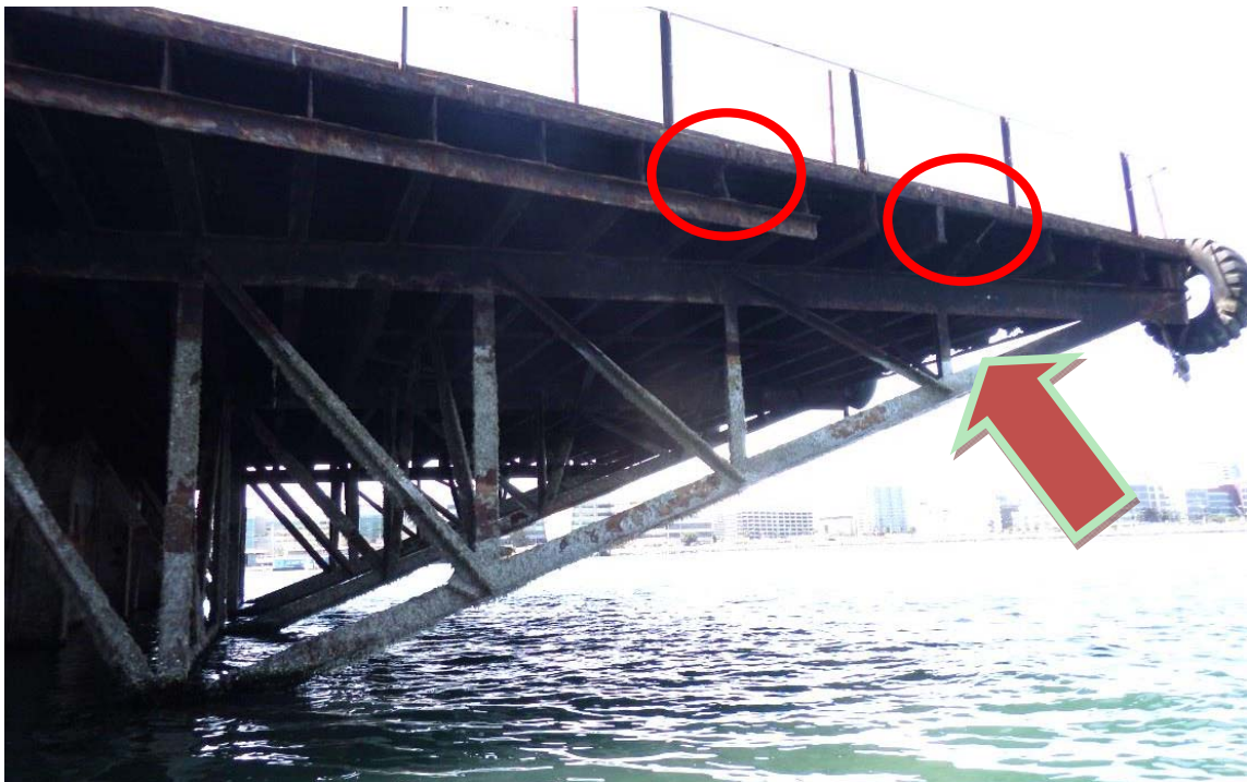
Photo 15: Two buckled transverse beams in the North apron, East edge circled in red. End plate of apron has developed significant corrosion holes indicated by arrow.
