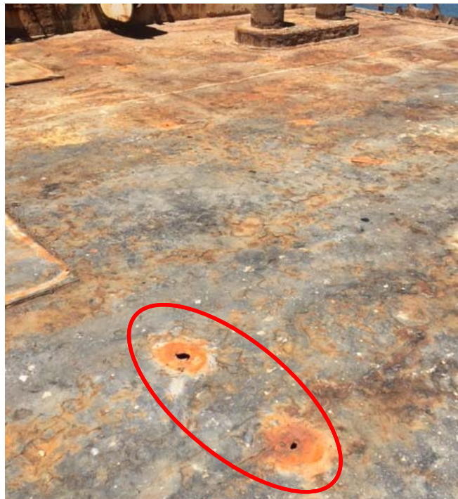
Photo 17: Pontoon Deck at Northwest corner of dry dock. Original plating has heavy pitting and rust film with isolated holes shown circled in red.
