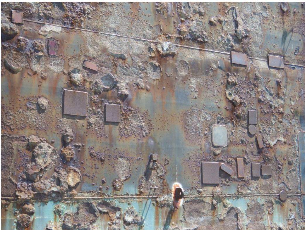
Photo 13: Example of the extensive amount of doubler plates found on the West outboard wing wall. Doubler plates server as a temporary water tight fix for a deteriorating plating structure.
