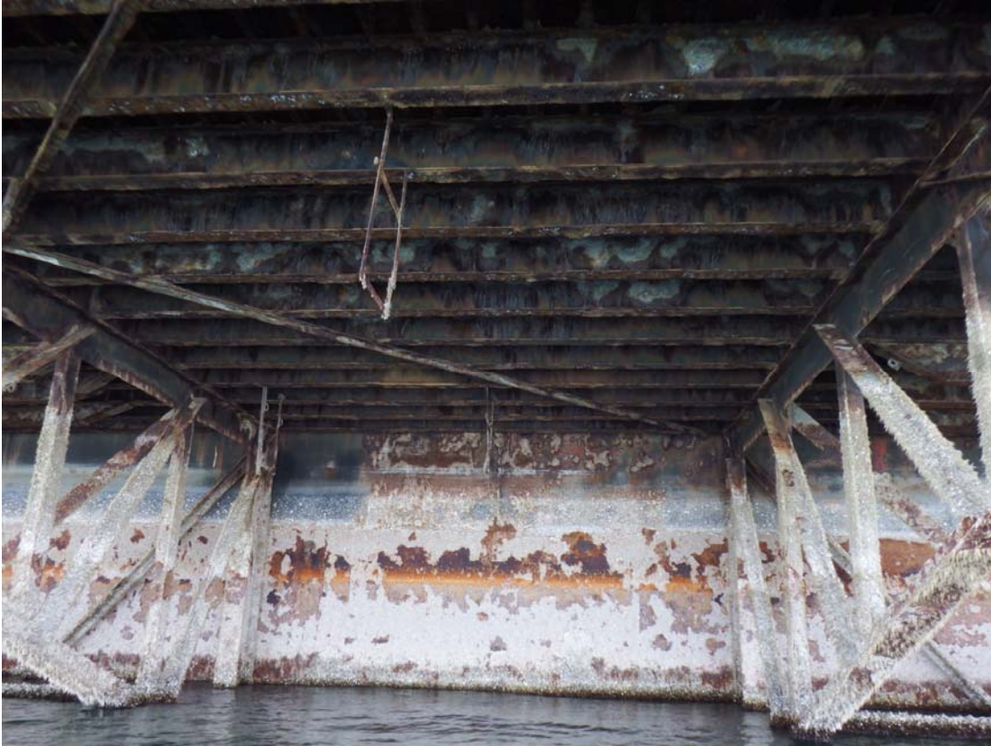
Photo 14: Typical condition of the North Apron structure. Paint failure with heavy scaling and noticeable metal loss due to corrosion throughout.
