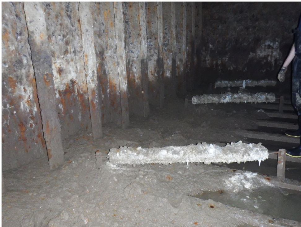
Photo 4: Typical condition of pontoon ballast tanks. Paint failure with medium rust scale on hull structure, zinc anodes intact, and about 18 inches of mud throughout.
