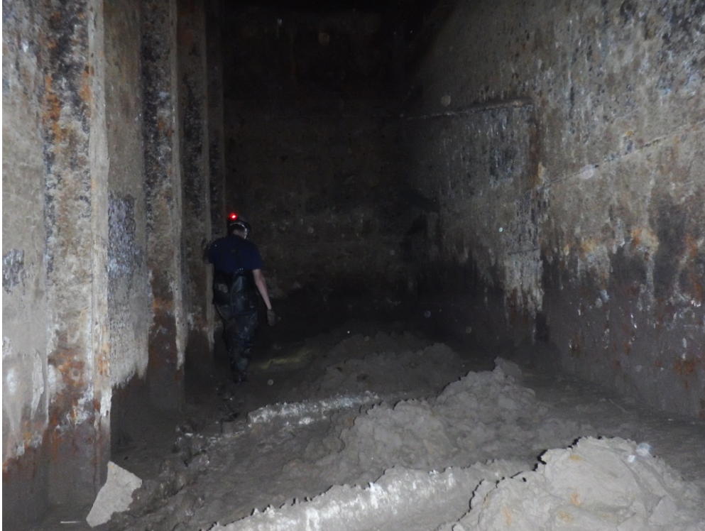
Photo 5: The extent of accumulated mud and sediment in the ballast tanks. Covered zinc annodes cannot adequately protect steel from deteriorating.
