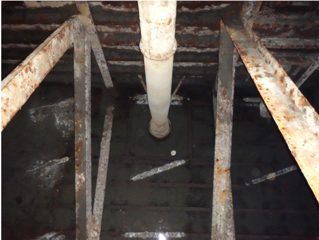
Photo 7: Typical dewatering intake and piping.
