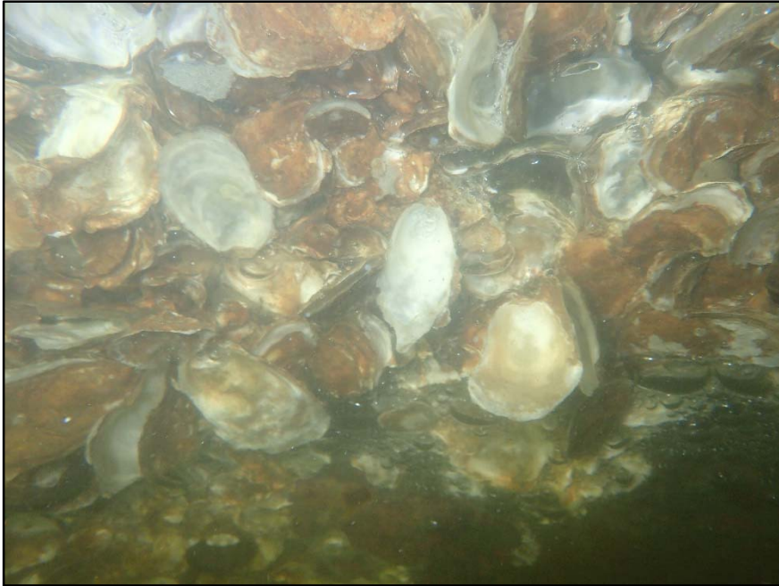
Photograph 3 : Underwater view of typical marine growth located along outer hull perimeter.
