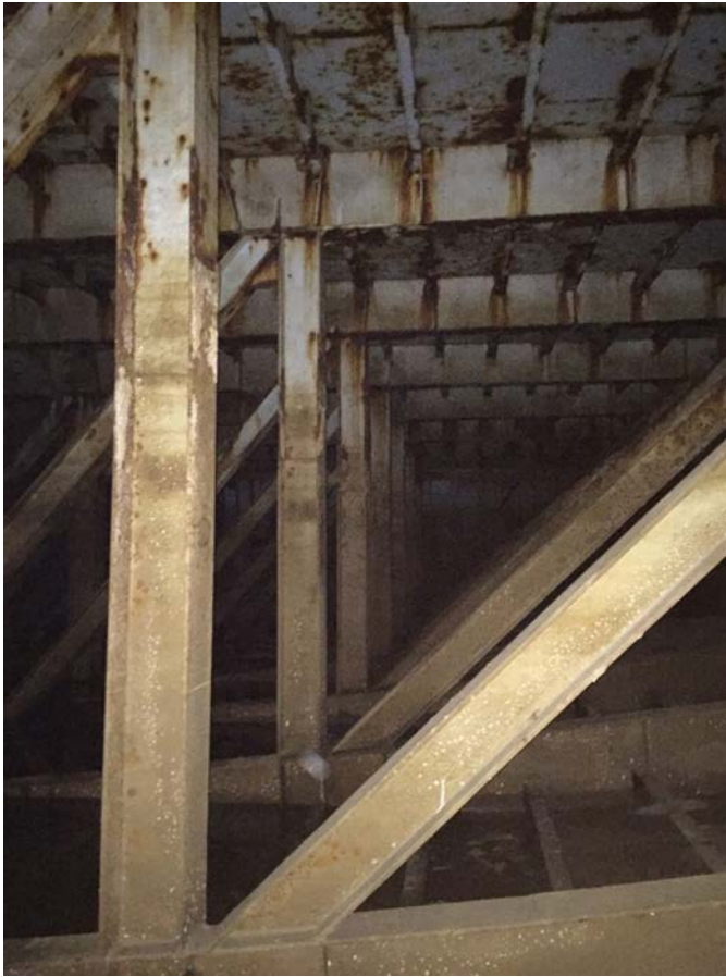
Figure 17: Tank 5 Corroded Members
