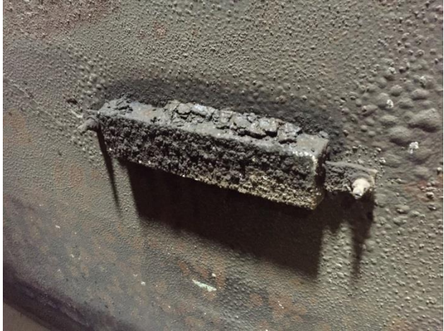
11. Sacrificial anode in Tank 9
