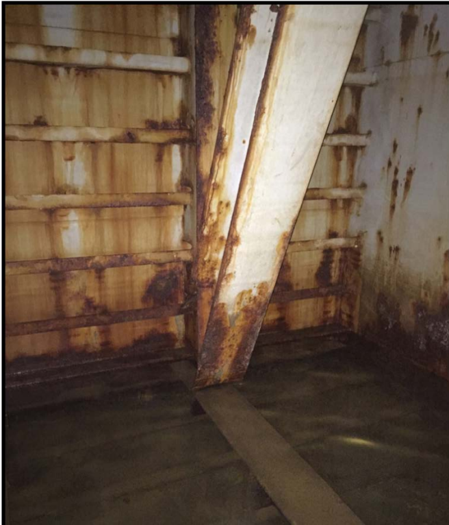
Figure 9: Corrosion Observed on Framing at Keel
