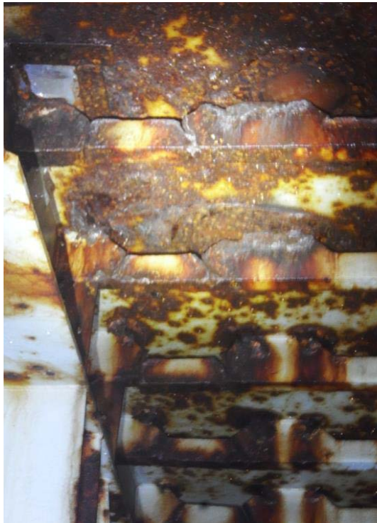
Figure 5: Pontoon Deck Stiffener Damage Example
