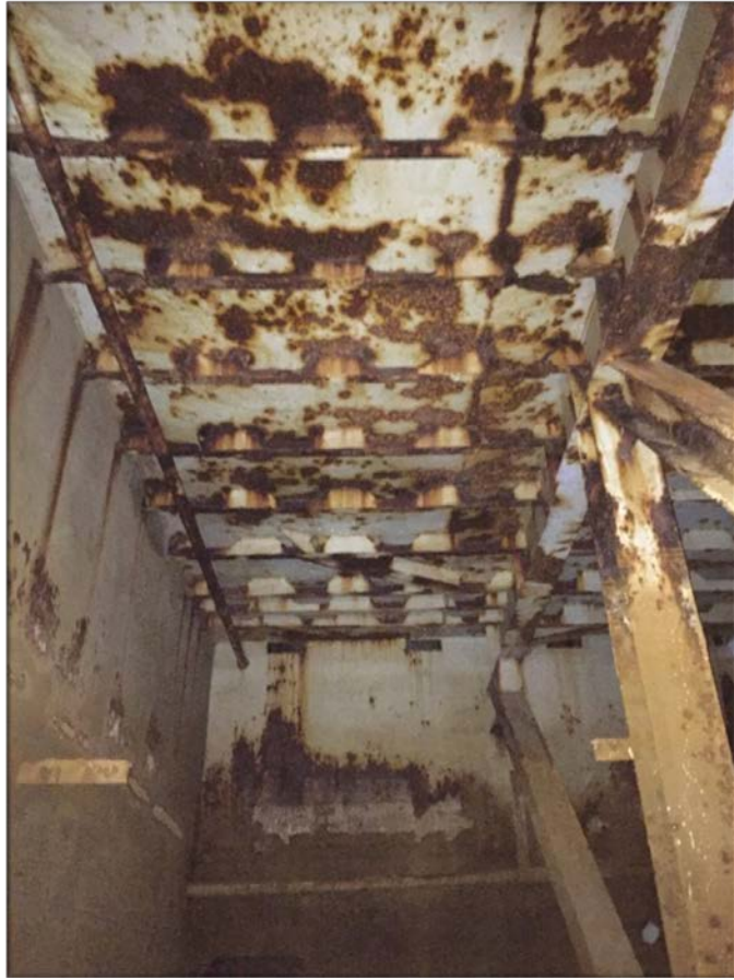
Figure 18: Typical Corrosion at Roof of Tank 6A
