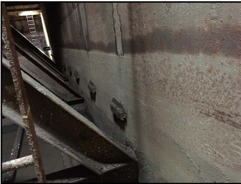
Figure 8: Interior Shell Plates and Anodes
