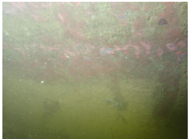
24. Typical hull deterioration after removal of marine growth
