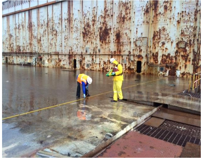
Figure 2: UT Reading on the Pontoon Deck topside.
