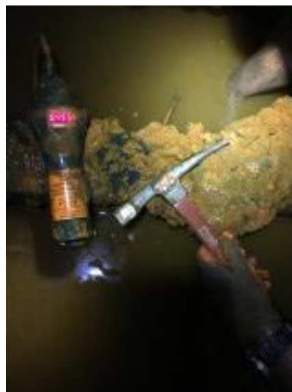
Figure 1: Technician holding the Cygnus 1 UT gauge probe against bottom steel after superficial rust and mud was removed with chipping hammer.
