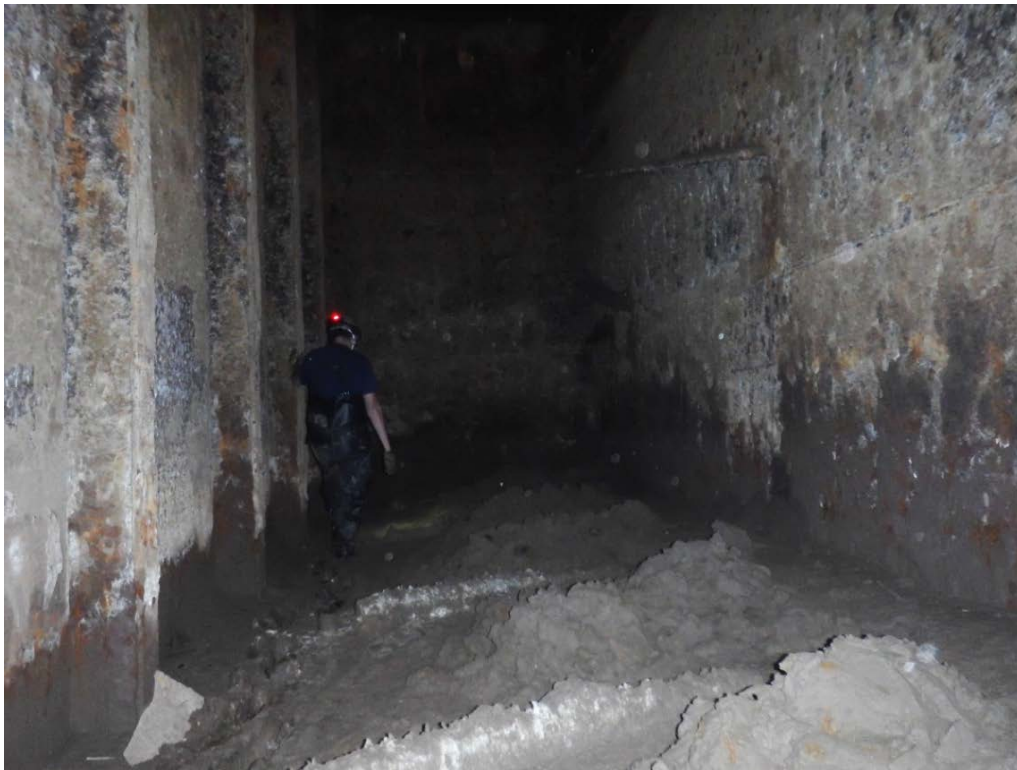
Figure 9: Mud and sediment in the ballast tanks (Heger Dry Dock Inc.)
