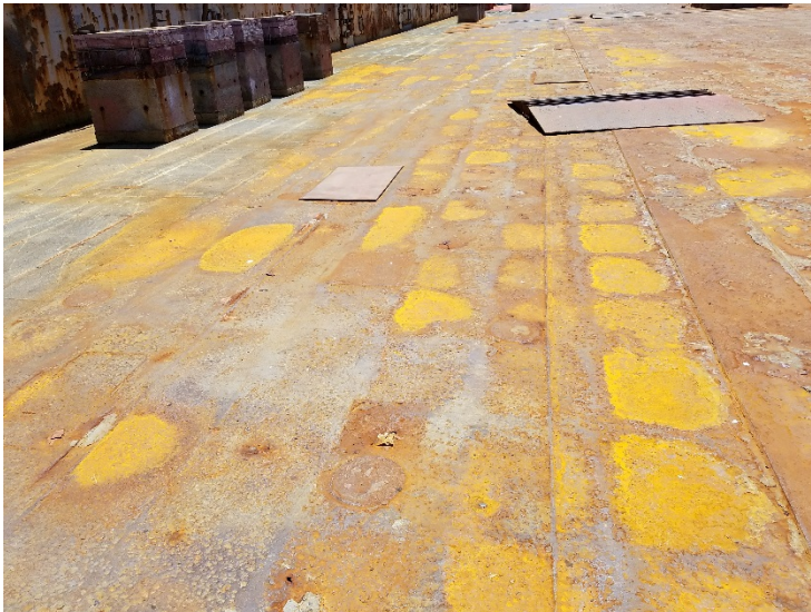
Figure 6: Typical Pontoon Deck Corrosion
