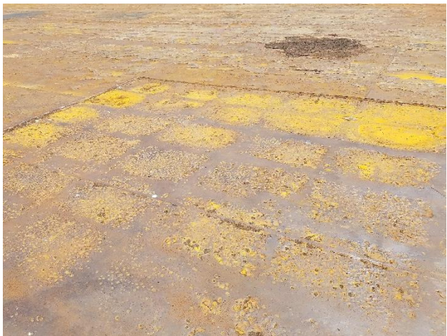
3. Close up of deflection and pitting
