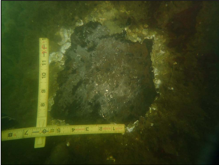
Photograph 11 : Underwater View of the Typical Steel Condition on the Steel Pipe Piles (Southeast Pile at Dolphn 4 Shown).
