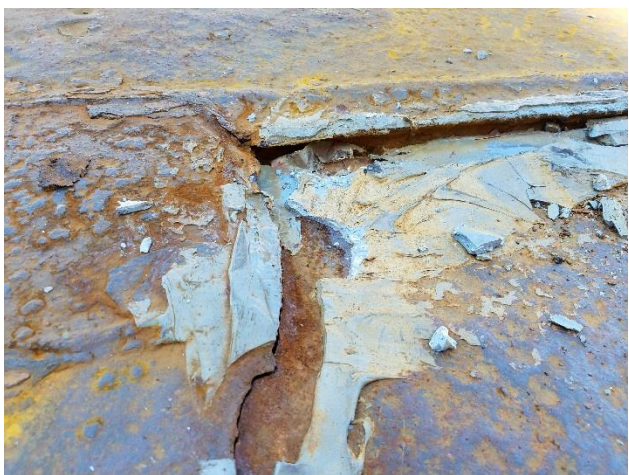
5. Failed epoxy repair of sheared plate at stiffeners
