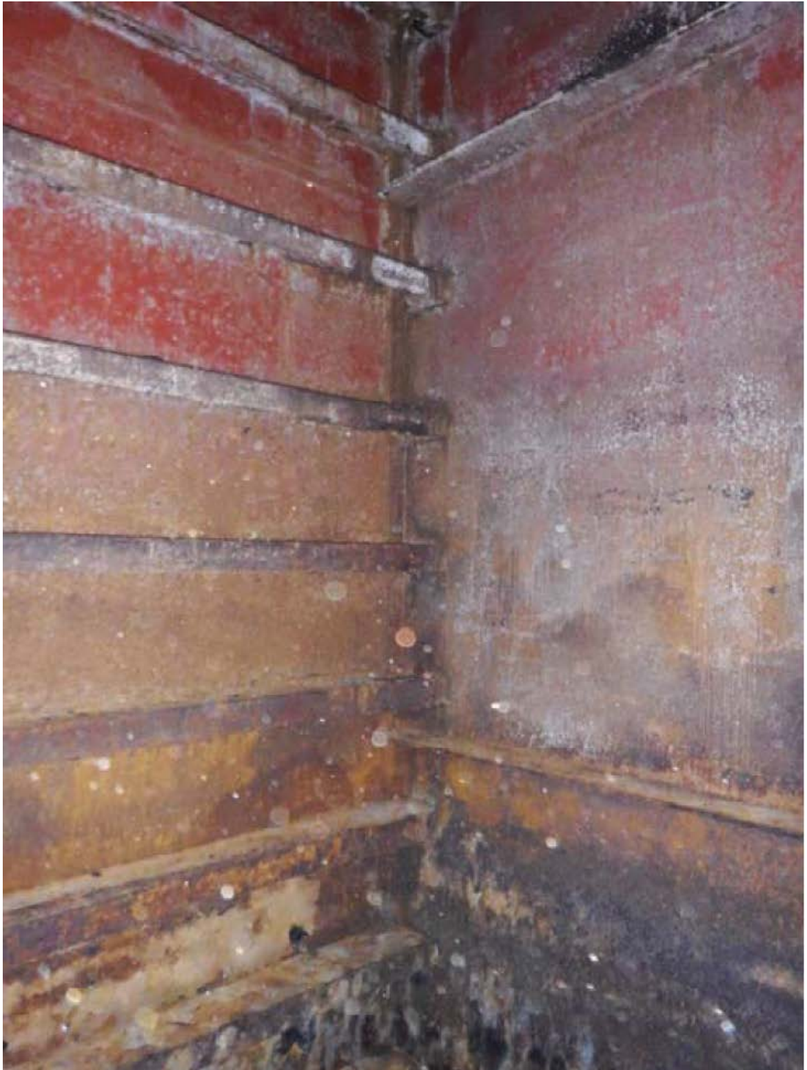
Figure 11: Typical condition of a buoyancy chamber. Paint failure and rust film beginning in lower 10 feet of tank with paint 70% intact in upper 10 feet (Heger Dry Dock Inc.)
