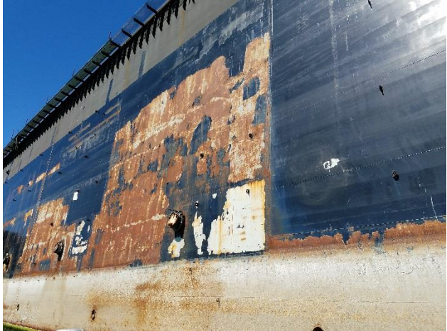
13. Outer shell panels – note recently replaced plates and corroding existing plates
