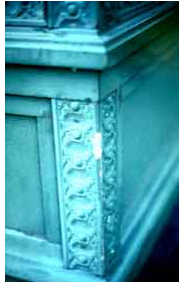
Substitute materials need to be located with care to avoid damage. The fiberglass column base has chipped, whereas the historic cast iron would have remained sound. Photo: NPS files.
