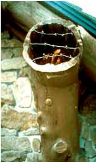
The core of a deteriorated wood outrigger was first drilled out. Photos (left and right): Courtesy, Harrison Goodall.
