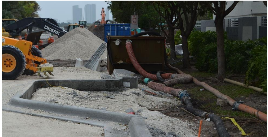
Elevated roadway construction - Miami Beach, FL ©User B137/Wikimedia Commons/This file is made available under the Creative Commons CC0 1.0 Universal Public Domain Dedication.
