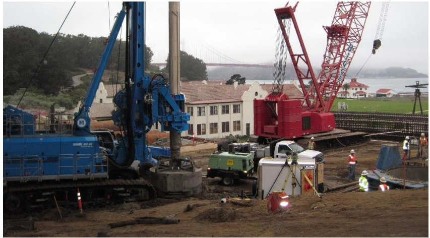
Installation of large drilled shafts to stabilize the shoreline would require large equipment as shown here - San Francisco, CA ©Fugro
