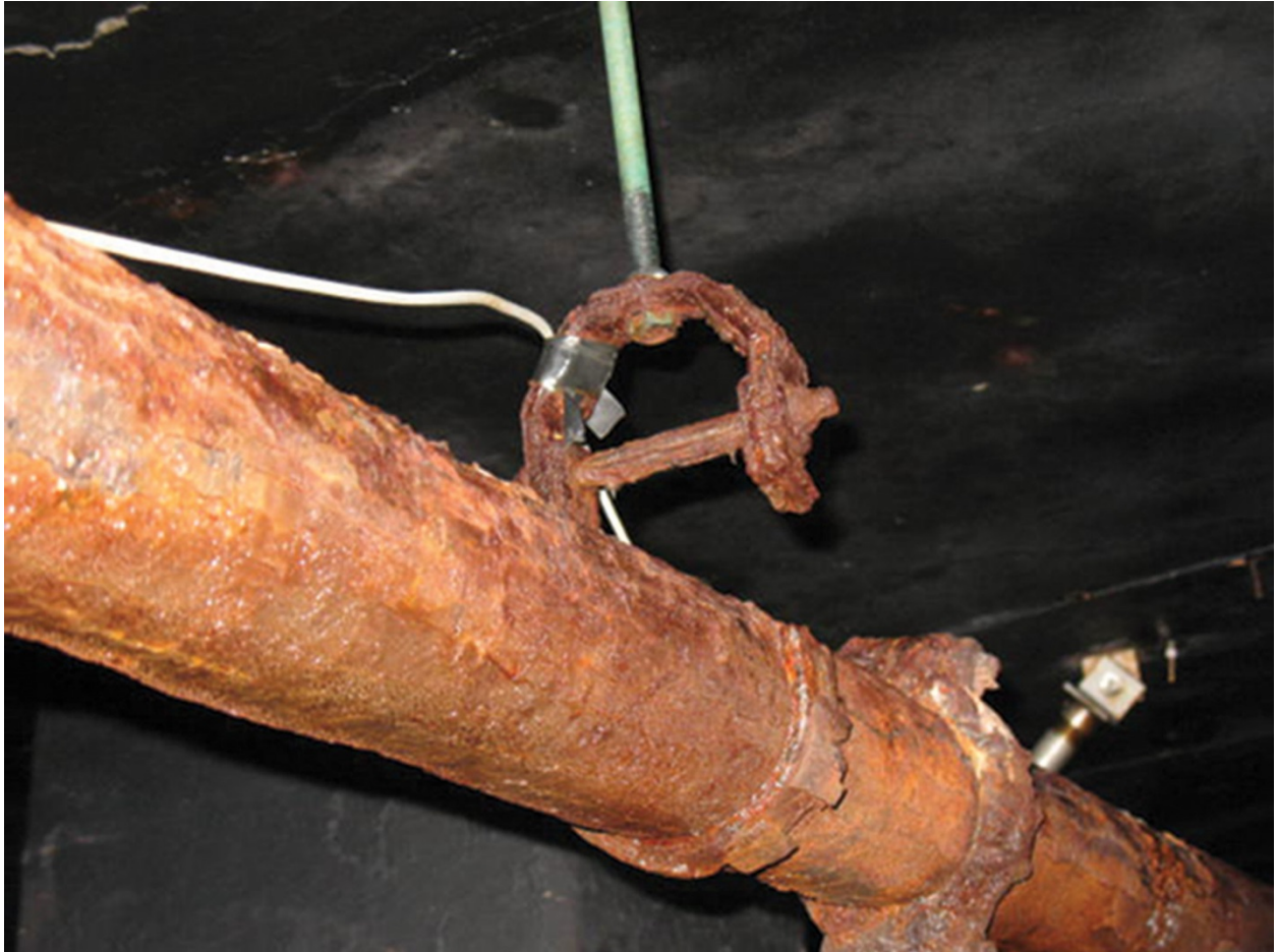
PHOTO 5 – Pipe Hanger Failure
