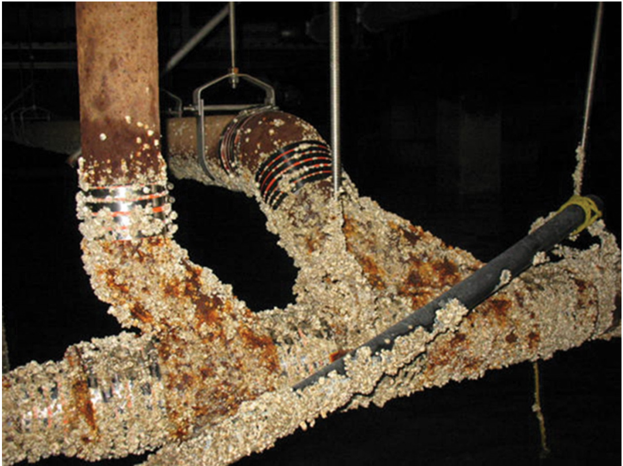
PHOTO 6 – Pipe with Barnacles
