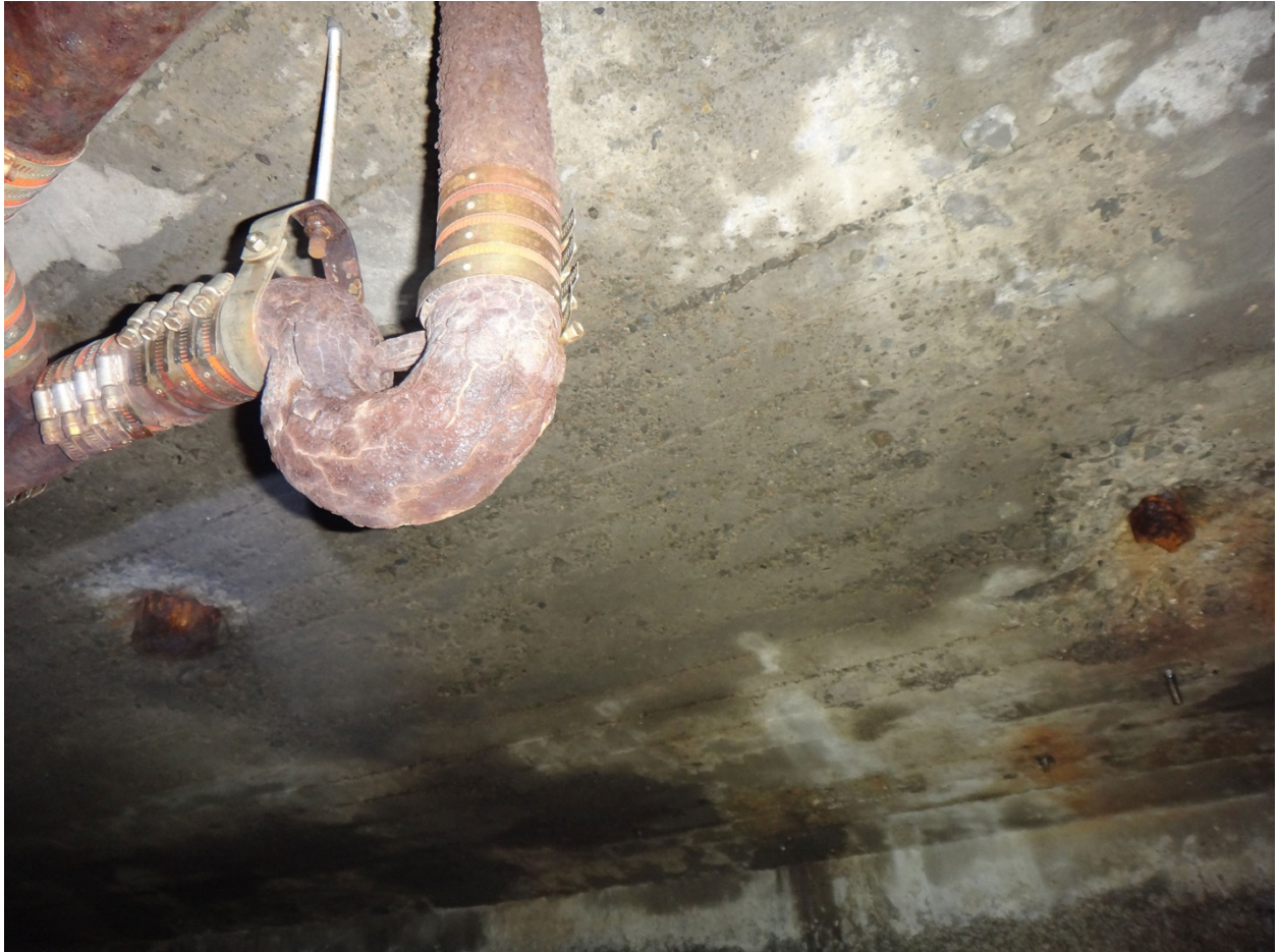
PHOTO 4 – Cast Iron Pipe - Flaking
