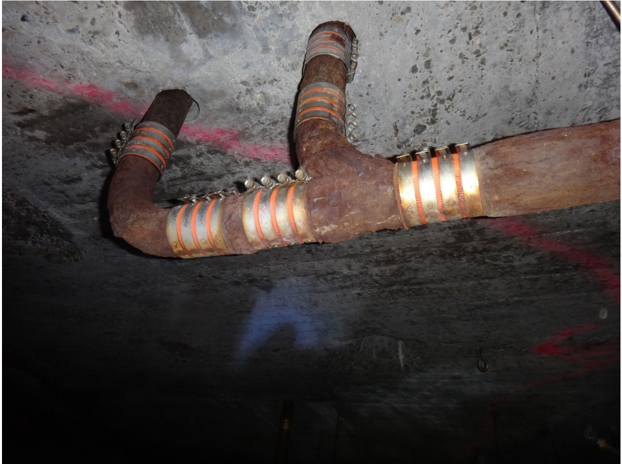
PHOTO 3 – Cast Iron Pipe – Pipe Diameter Is Larger than Band
