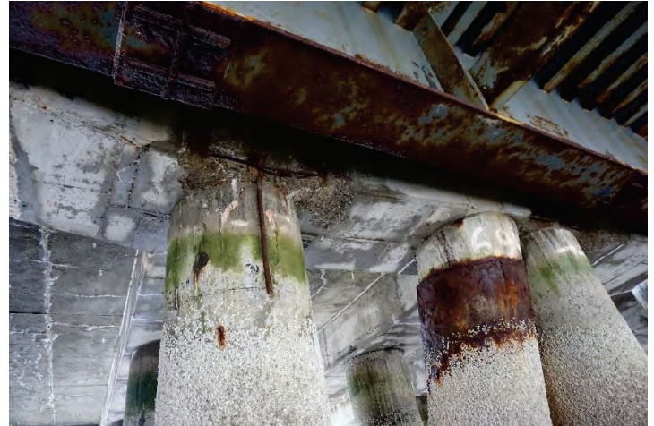
Figure 34 - Loss of Protective Coating on Bridge, Spalled Pile Cap
