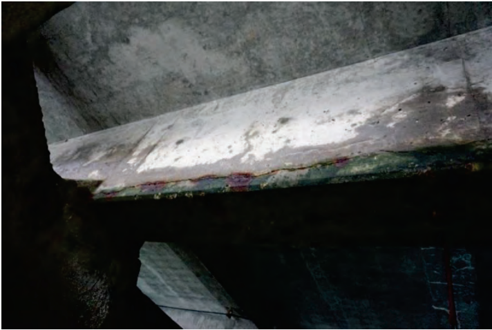
Figure 4 – Crack in Protective Concrete Over Steel Girder, Indicating Corrosion
