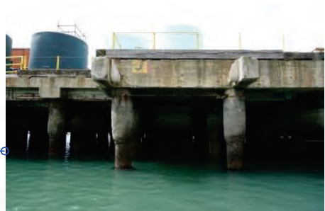
Cracked Pile Cap
