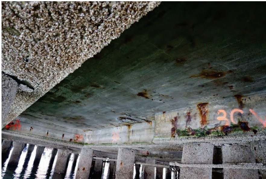
Figure 22 – Spall on Deck & Corrosion Stains
