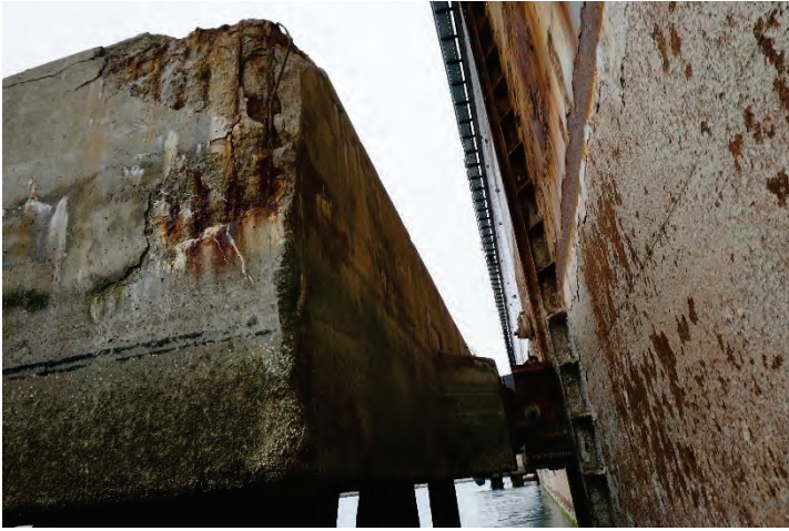
Figure 37 - Spall on Edge of Pile Cap
