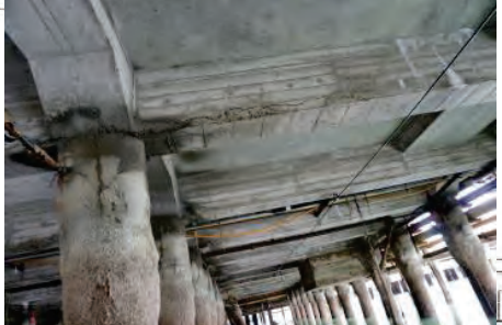
Crack on Beam
