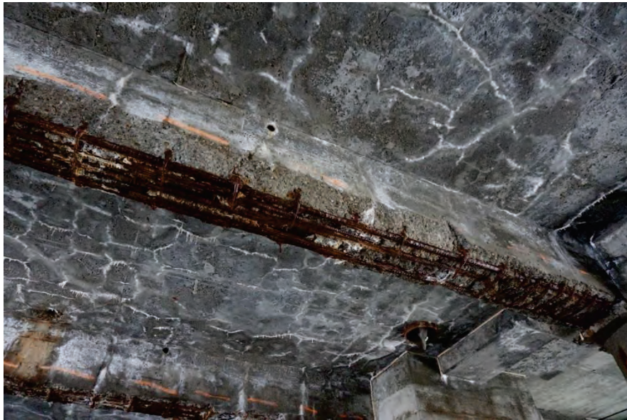
Figure 24 – crack on deck
