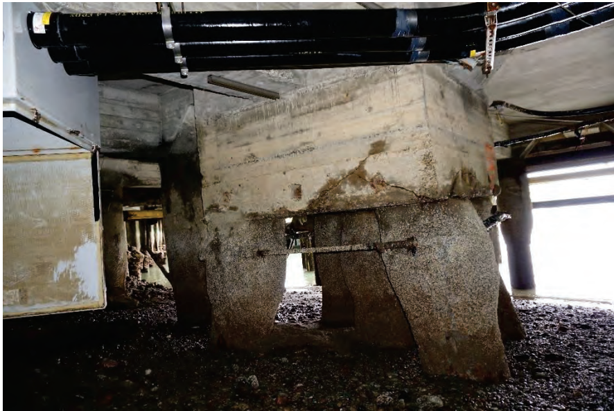
Figure 18 – Cracked Pile Cap
