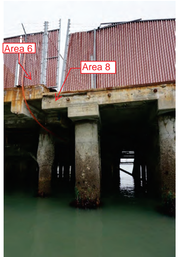
Figure 27 - Settlement of Piles
