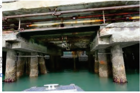
Spalled Pile Cap
