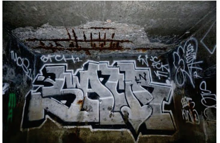
Figure 15 – Spall on Overhead Deck
