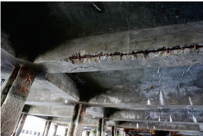
Figure 31 – Spall on Beam
