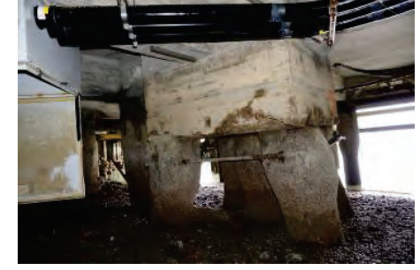
Major Crack on Pile Cap
