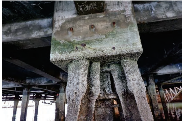
Figure 30 – Crack on Pile Cap
