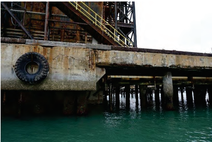
Figure 39 - Crack and Spalling on Dolphin
