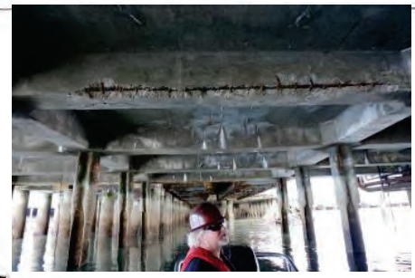
Severe Spall on Beam
