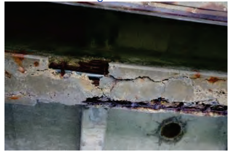
Spalled Duct Bank
