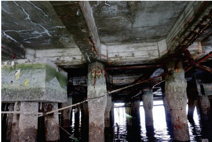
Figure 21 – Spall and Crack on Beams
