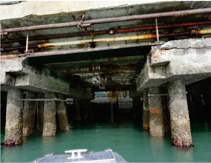
Figure 9 - Crack on Pile Cap
