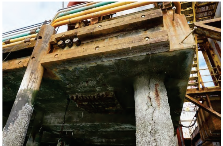
Figure 32 – Spall on Deck
