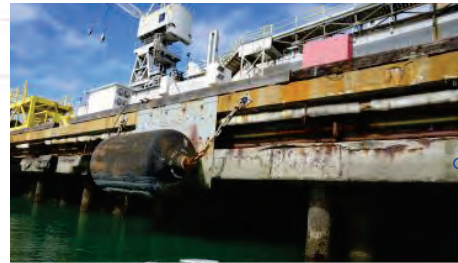
Pile Cap Spall and Crack
