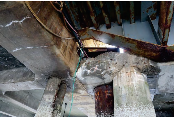
Figure 35 - Minor Corrosion and Loss of Protective Coating
