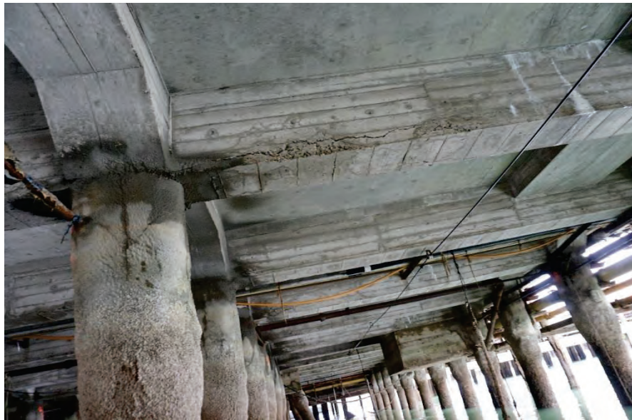
Figure 19 – crack on Beams
