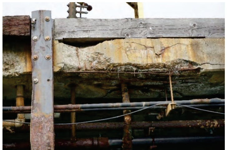
Figure 7 – Spall on Deck Edges
