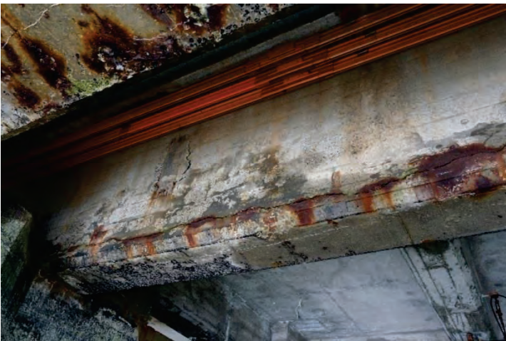
Figure 11 - Cracks on Beam
