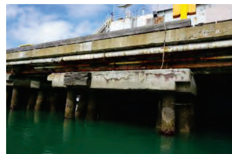
Major Crack on Pile Cap
