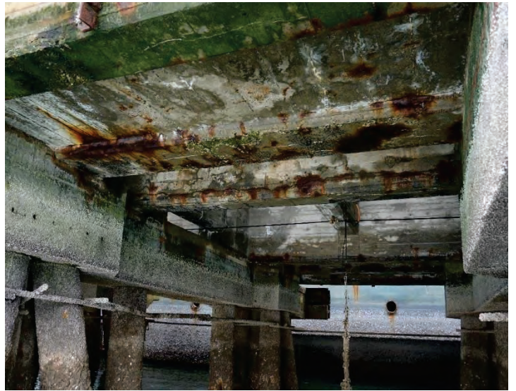
Figure 10 - Cracks and Corrosion on Beams
