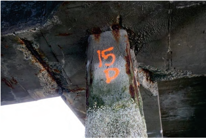
Figure 29 – Spall on Beam and Pile Cap
