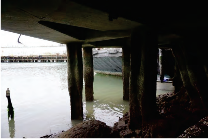
Figure 14 – Exposed Steel Pile and Corrosion
