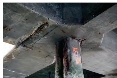
Spalled Beam & Pile Cap
