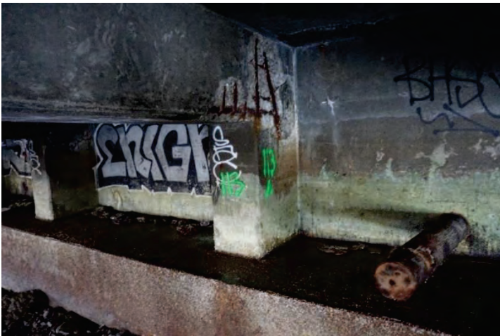
Figure 16 – Spall on Bulkhead Column and Beam
