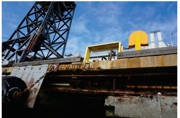
Figure 12 - Spall on Deck Edge
