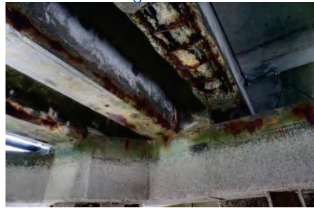
Spalled Duct Bank & Exposed Conduit
