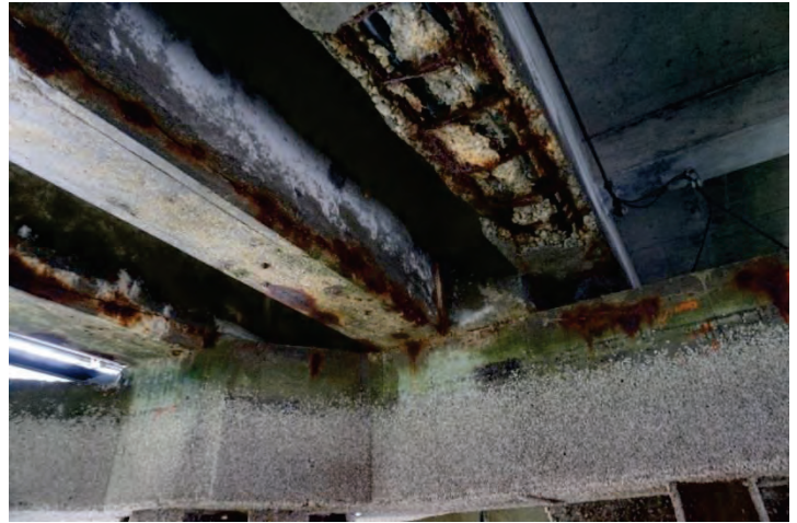
Figure 5 - Spalled Duct Bank and Exposed Conduit
