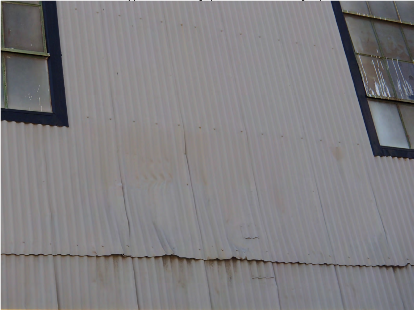
Photo 9. View of the typical impact damage in the metal siding
