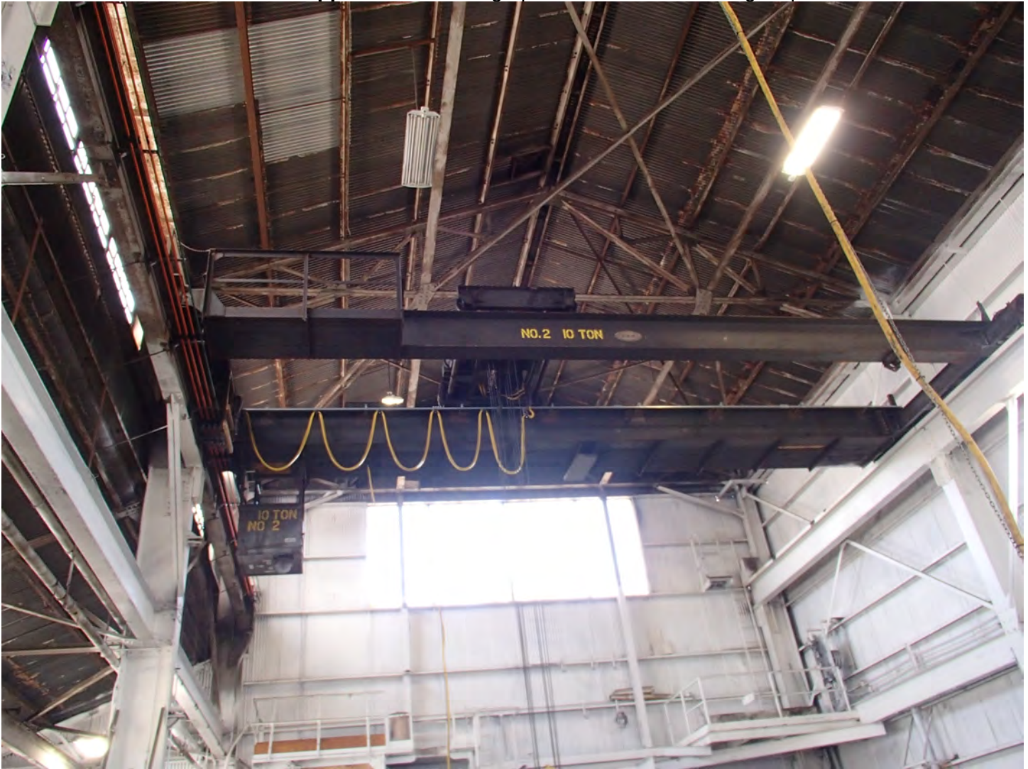
Photo 2. View of the 10-ton cranes
