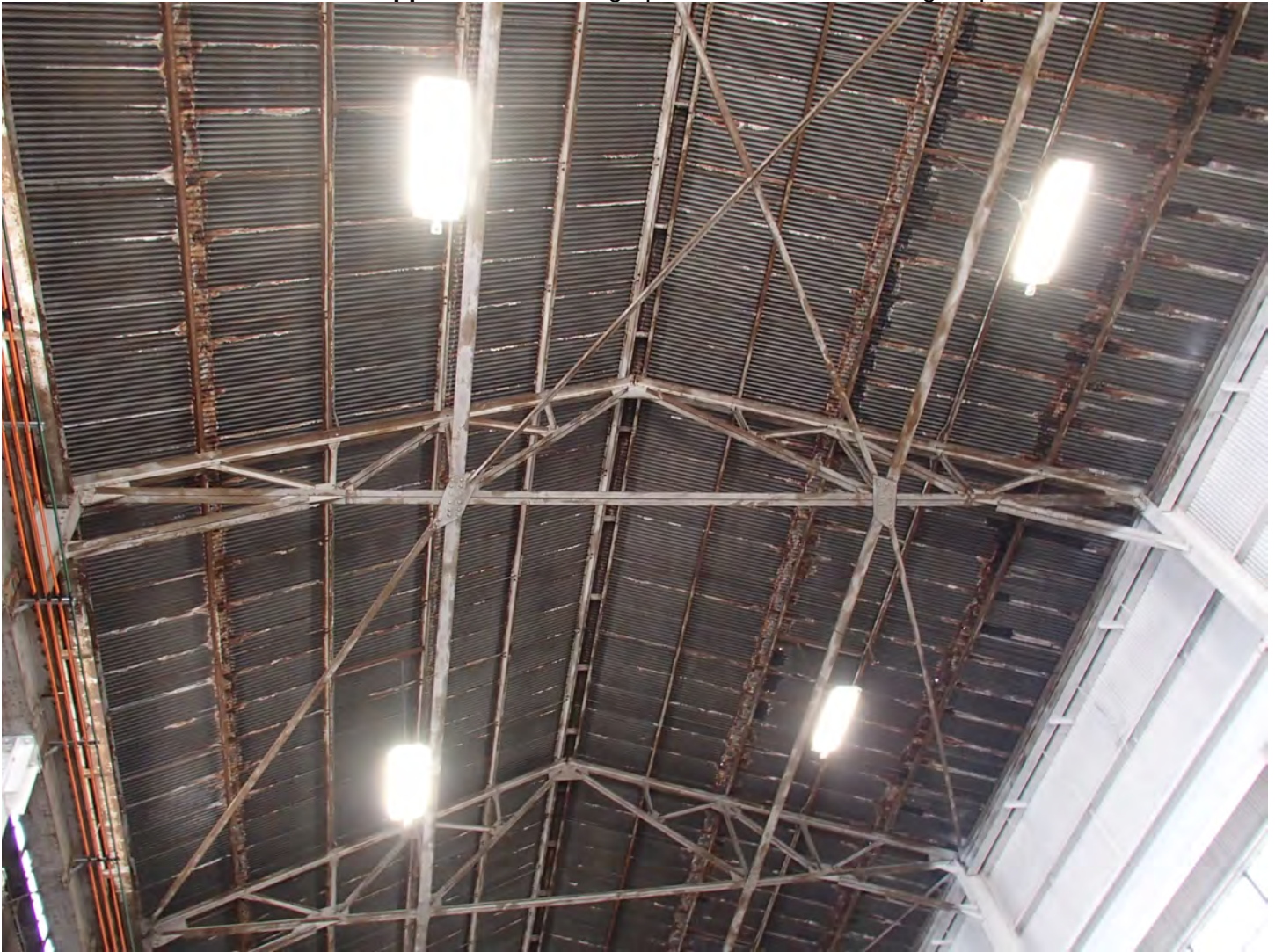
Photo 5. View of the steel roof truss and underside of the metal deck
