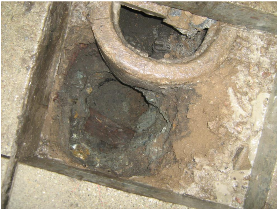
Photograph 7 - Air-knife boring located two feet west of suspect vent line. Photograph shows abandoned water valve inside valve box.
