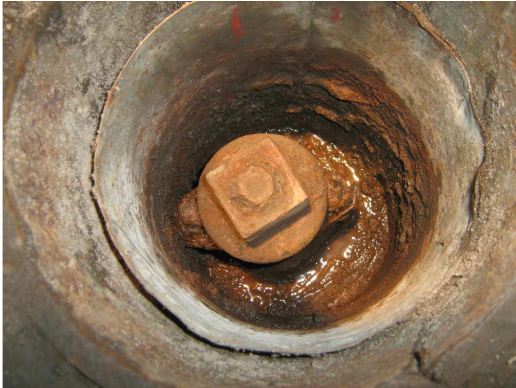
Photograph 10 – Valve inside circular steel vault east of Building 14
