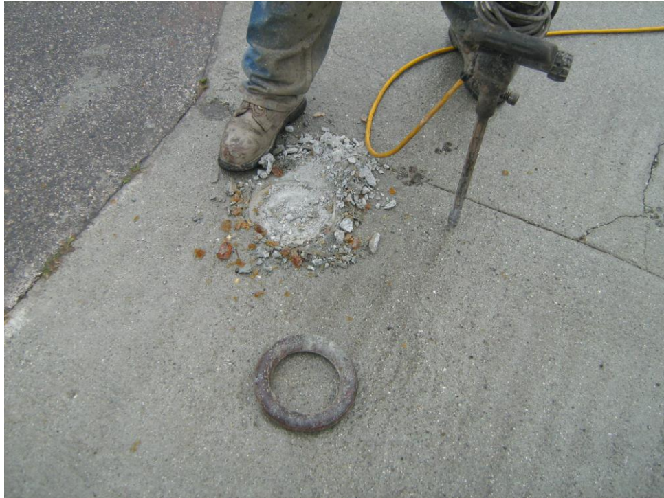
Photograph 13 – Previously unidentified metal object imbedded in concrete near Building 11 is removed and identified as a steel ring
