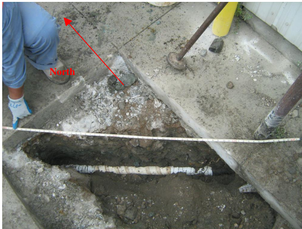
Photo 9 - Continuation of the suspect vent line plunging approximately 11 degrees in the northwest direction towards Illinois Street
