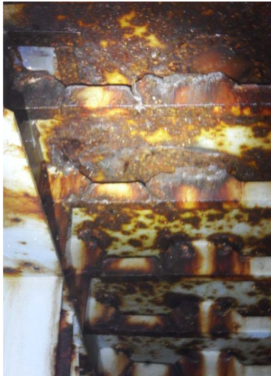
Figure 5: Pontoon Deck Stiffener Damage Example
