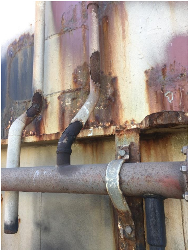
9. Typical pipe and steel corrosion at wing wall
