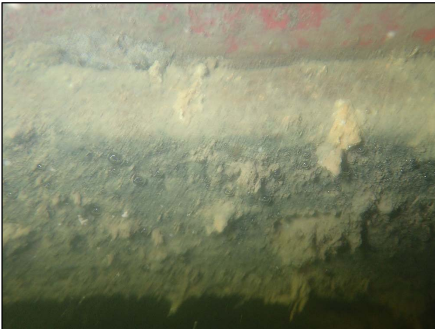
Photograph 6 : Underwater view of typical sacrificial anode condition.
