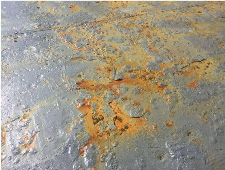
Figure 4: Typical Pontoon Deck Corrosion
