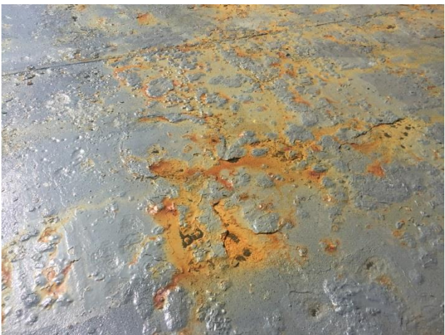
5. Close up of pontoon deck corrosion
