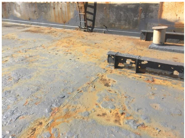
6. Wide view of pontoon deck corrosion
