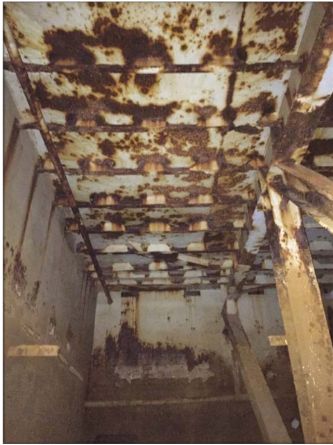
Figure 18: Typical Corrosion at Roof of Tank 6A
