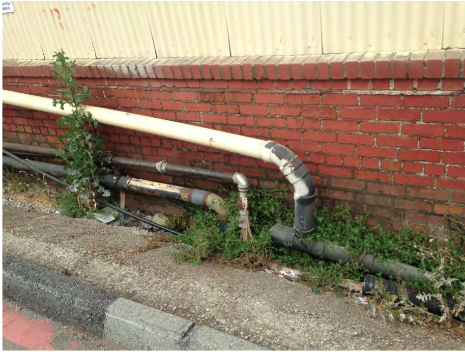
Figure 16. 2" compressed air service located at the exterior of building
