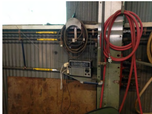
Figure 40. Natural gas distribution piping
