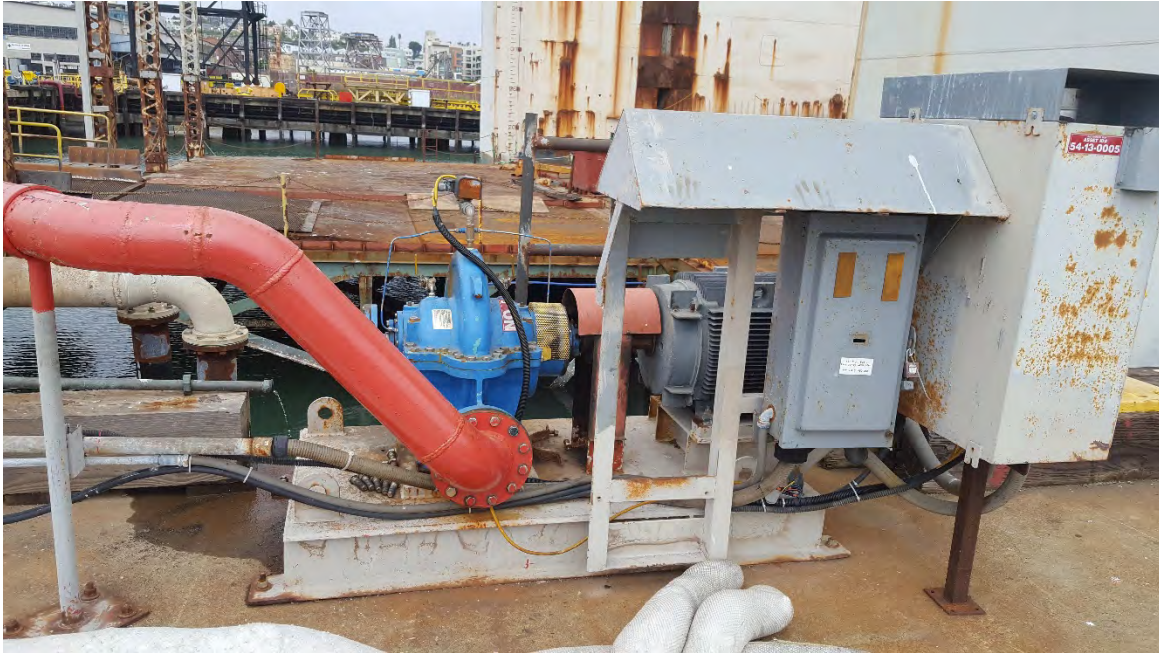
Figure 55. 100 HP Pier 4 Salt Water Pump (P4SWP)
