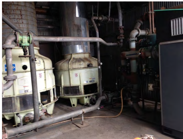
Figure 3. Cooling Towers in Building 107
