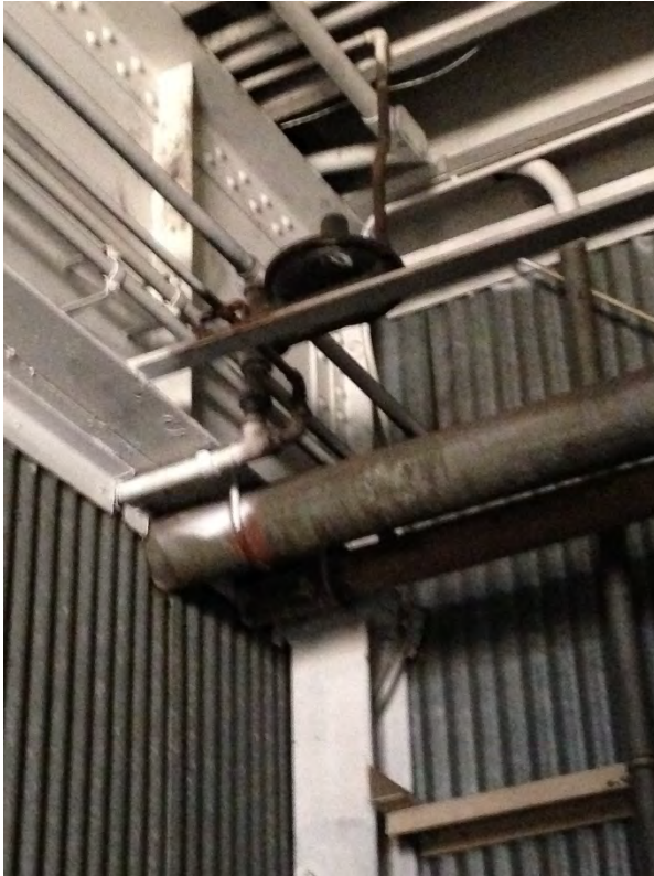
Figure 38. Natural gas 1/2" regulator, may be main service
