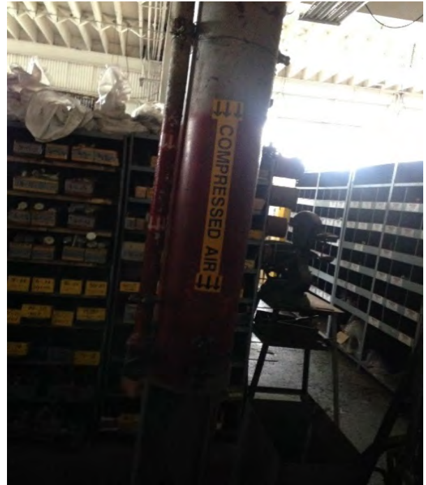
Figure 19. Compressed air 6" service size valve
