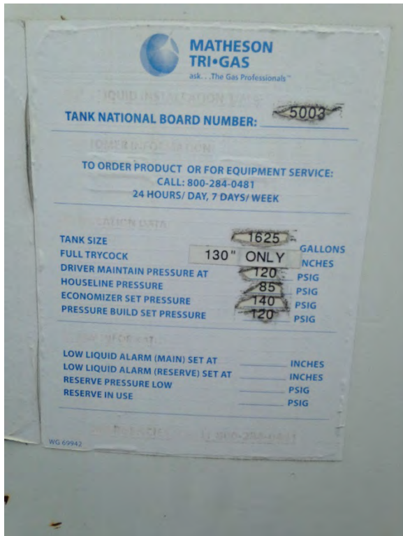
Figure 43. Oxygen tank nameplate
