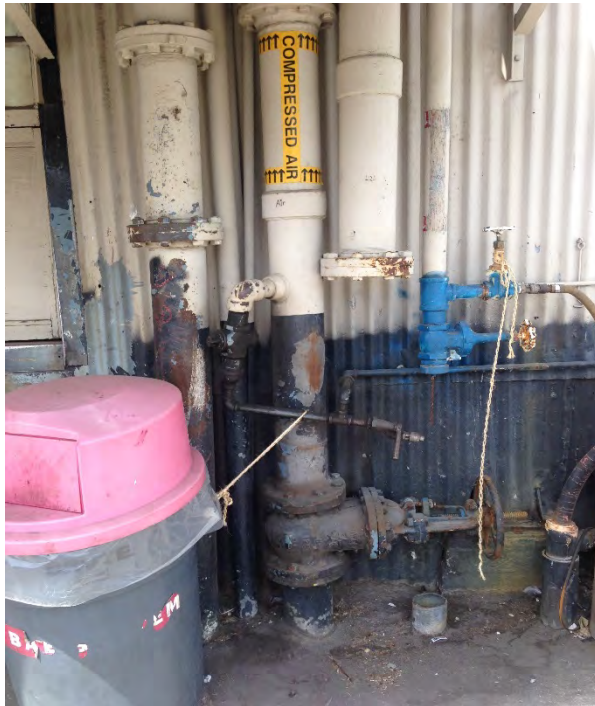
Figure 18. Compressed air 6" service size valve
