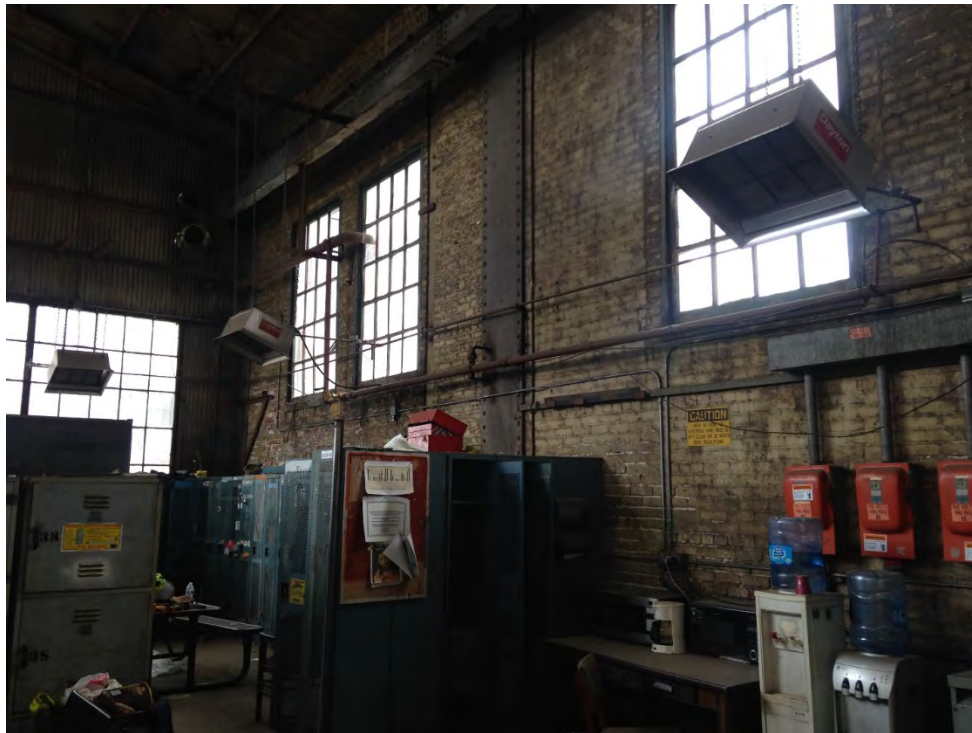
Figure 36. Building 105 gas heater
