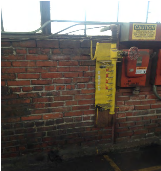
Figure 14. Interior compressed air 2" service size
