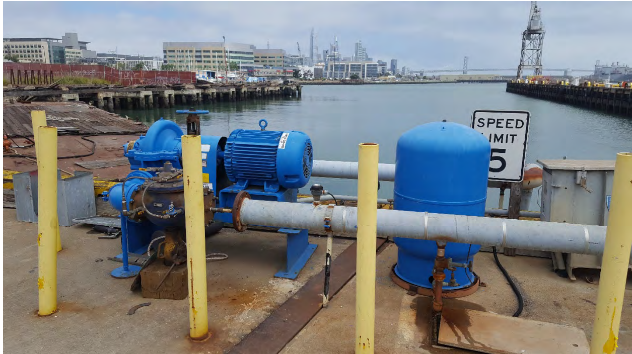
Figure 51. 75 HP Fresh Water Booster Pump
