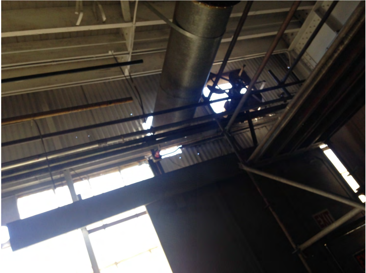
Figure 49. Disconnected Oxygen/Acetylene 1" service size
