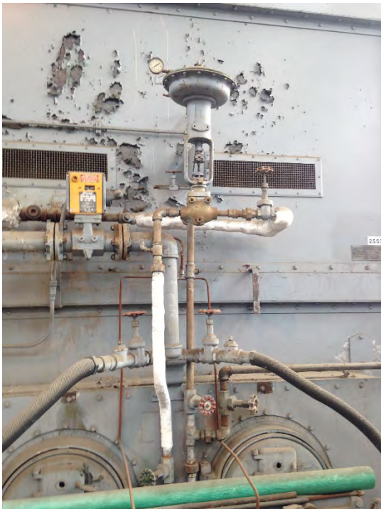
Figure 35. Boiler # 1 natural gas 2" distribution to each chamber
