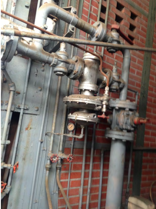
Figure 33. Natural gas Boiler # 1 - 4" service size
