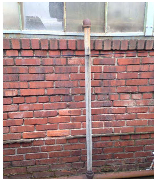
Figure 15. Exterior compressed air 2" service size
