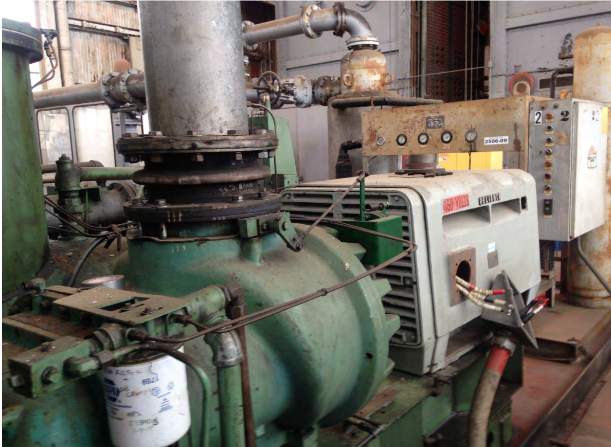
Figure 6. Compressors located in building 103
