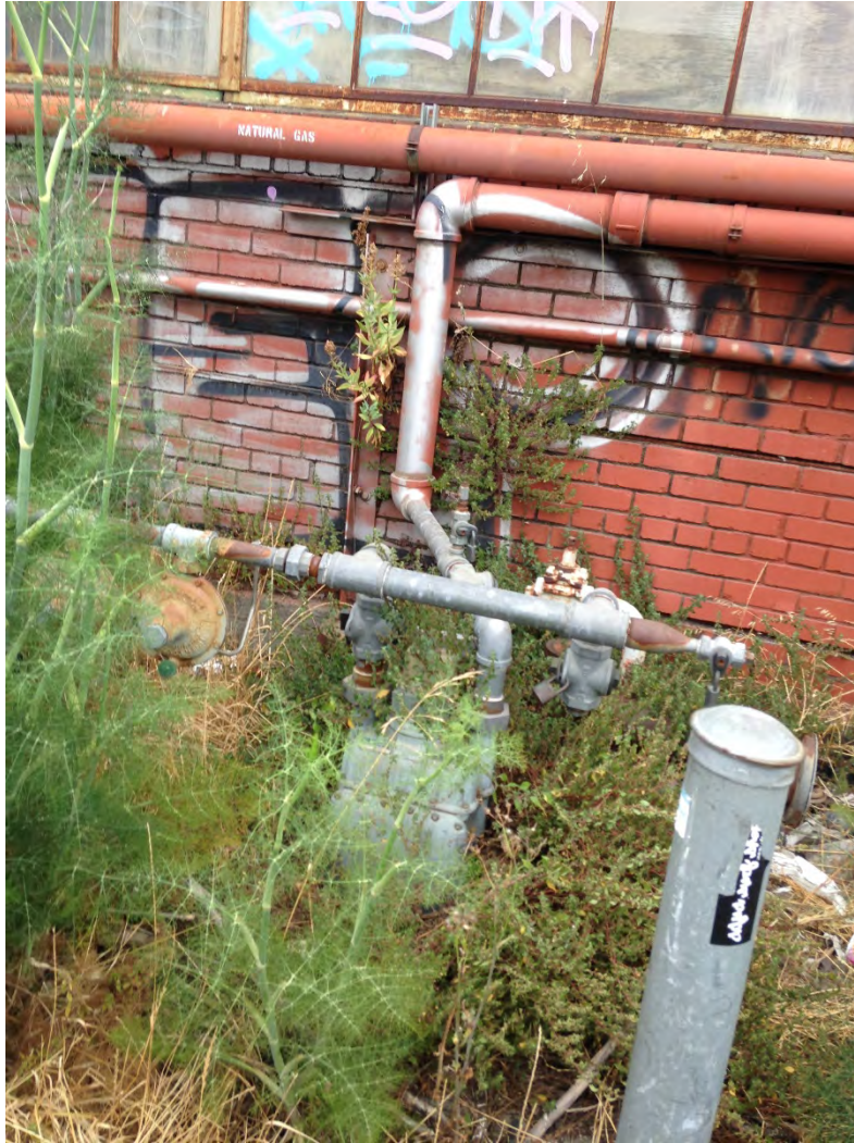
Figure 30. PG&E gas meter behind Building 103
