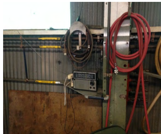
Figure 21 Compressed air 6" service size valve
