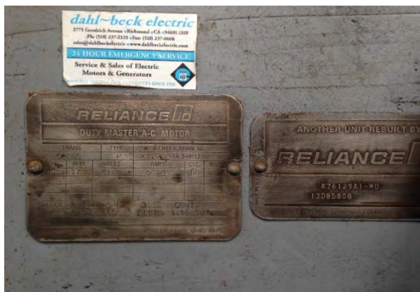
Figure 7. Compressor Motor Nameplate
