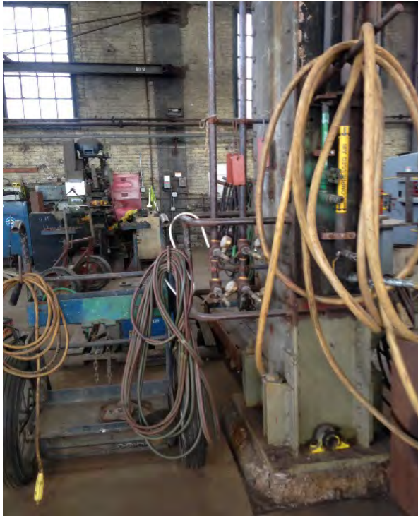
Figure 12. Compressed air connections
