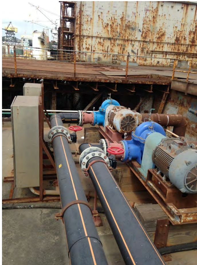
Figure 56. 125 HP Salt Water Auxiliary Cooling Pump #1 (SWACP1) - east pump- Installed in 2002 125 HP Salt Water Cooling Pump #2 (SWACP1) - west pump- Installed in 2002
