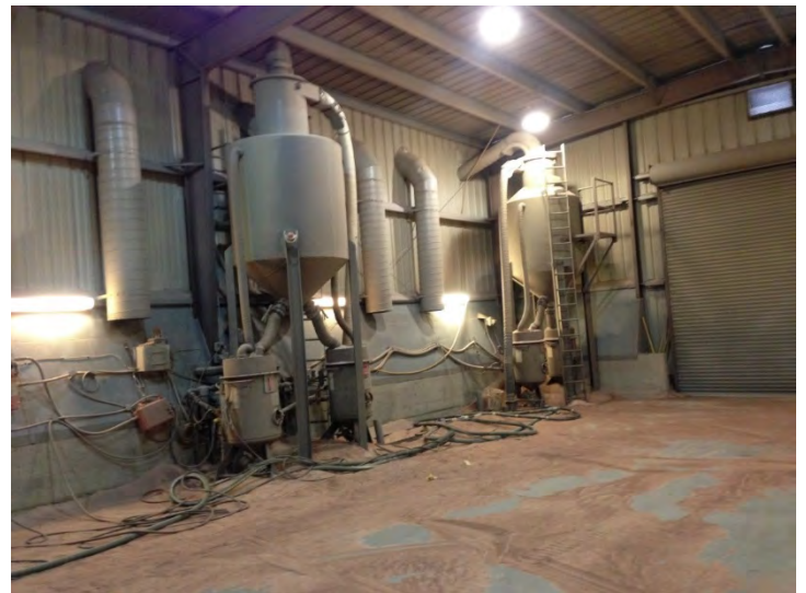
Figure 25. Compressed air distribution system
