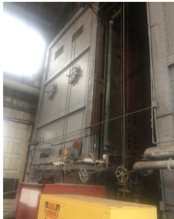
Figure 27. Steam system boilers
