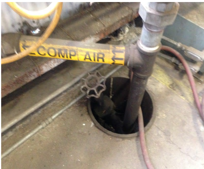
Figure 11. Compressed air main service valve
