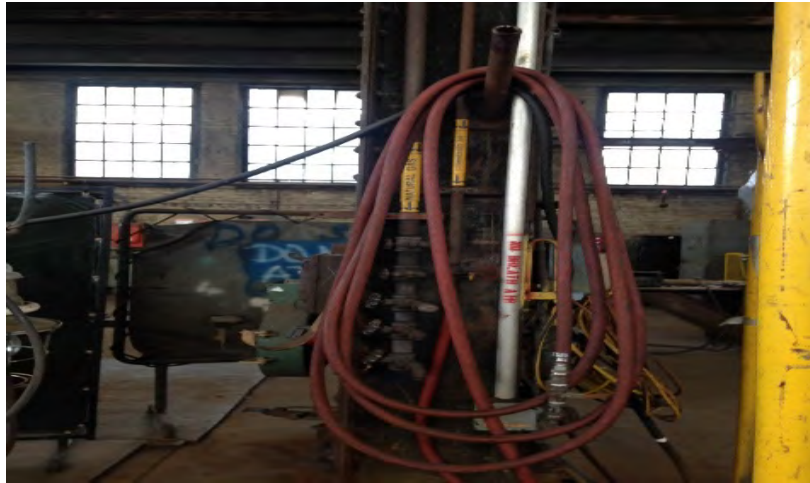
Figure 47. Welding gas (Oxygen/Acetylene) disconnect
