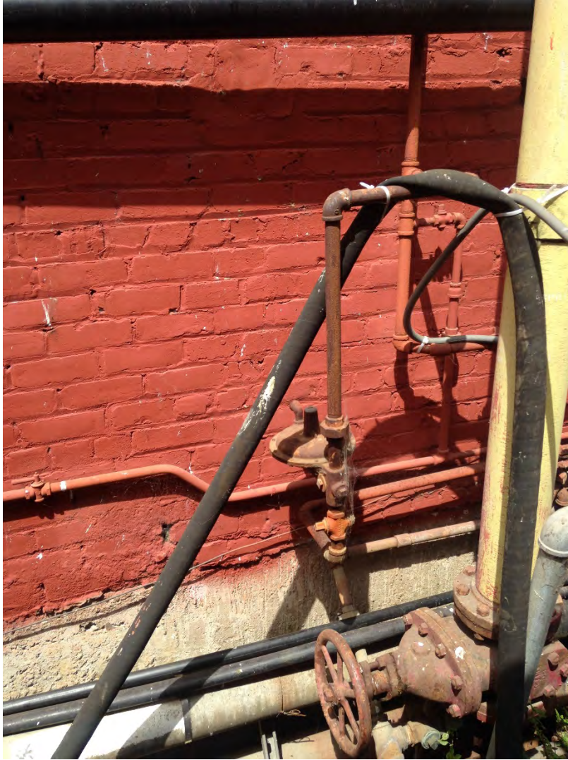
Figure 41. Natural gas ½" service size (behind Building 111)
