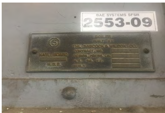
Figure 26. Steam system boiler nameplate
