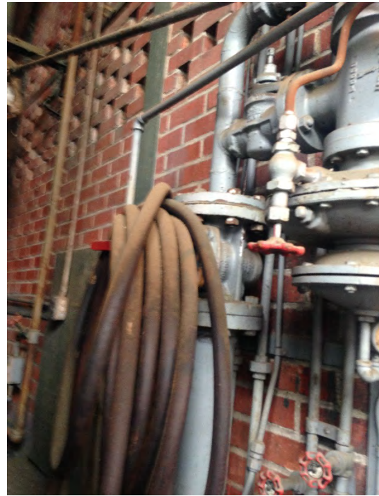
Figure 34. Natural gas Boiler # 2 - 4" service size
