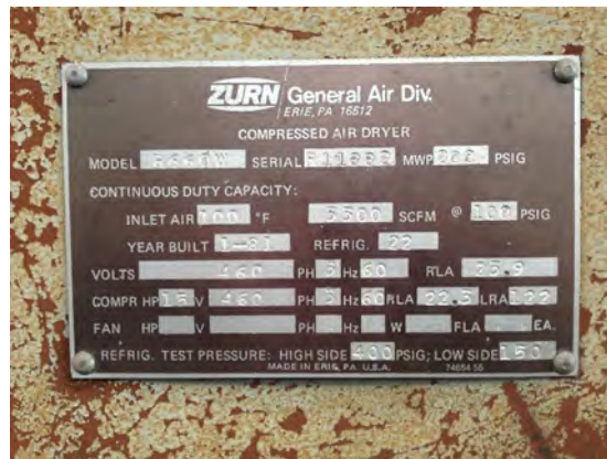
Figure 8. Air Dryer Nameplate
