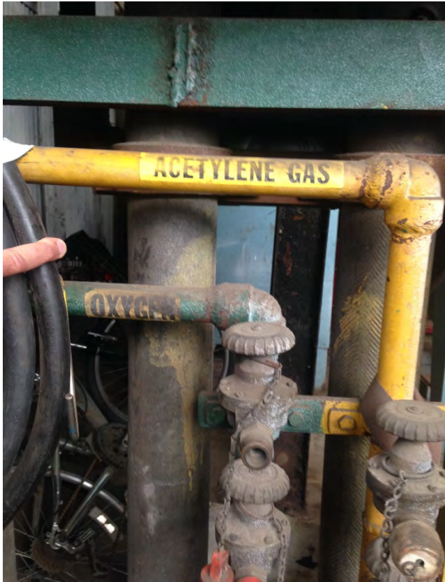
Figure 46. Oxygen/Acetylene Welding gas 1" service size
