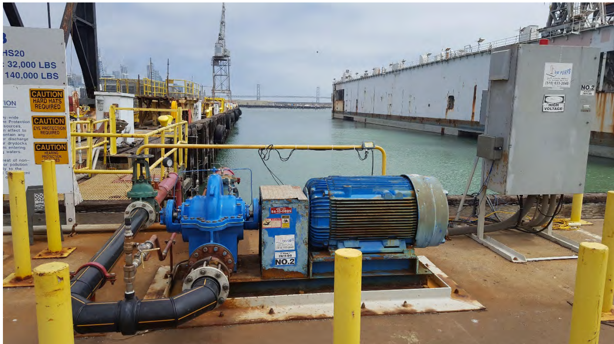
Figure 53. 250 HP Pier 3 Salt Water Pump (P3SWP)
