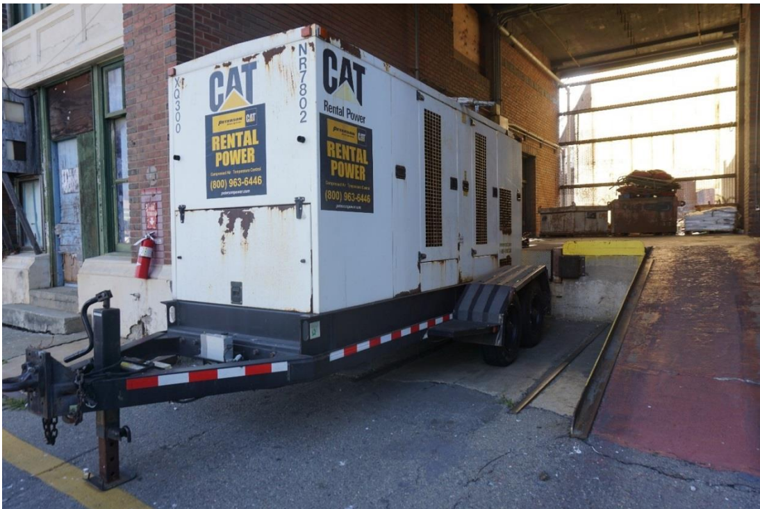
Caterpillar XQ300 Diesel Generator - 300KW (Yard)
