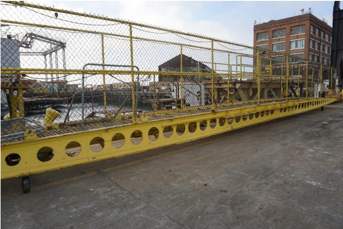
70 Ft Gangway (Wharf 3)
