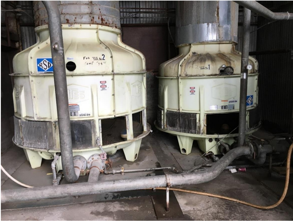
Cooling Tower Tanks -2 units (back of Bldg. 108)
