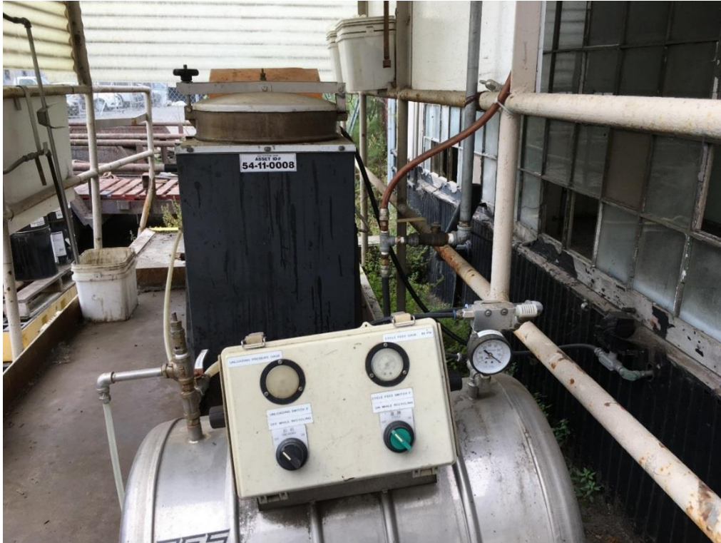
Solvent Recycler (outside Bldg. 109)
