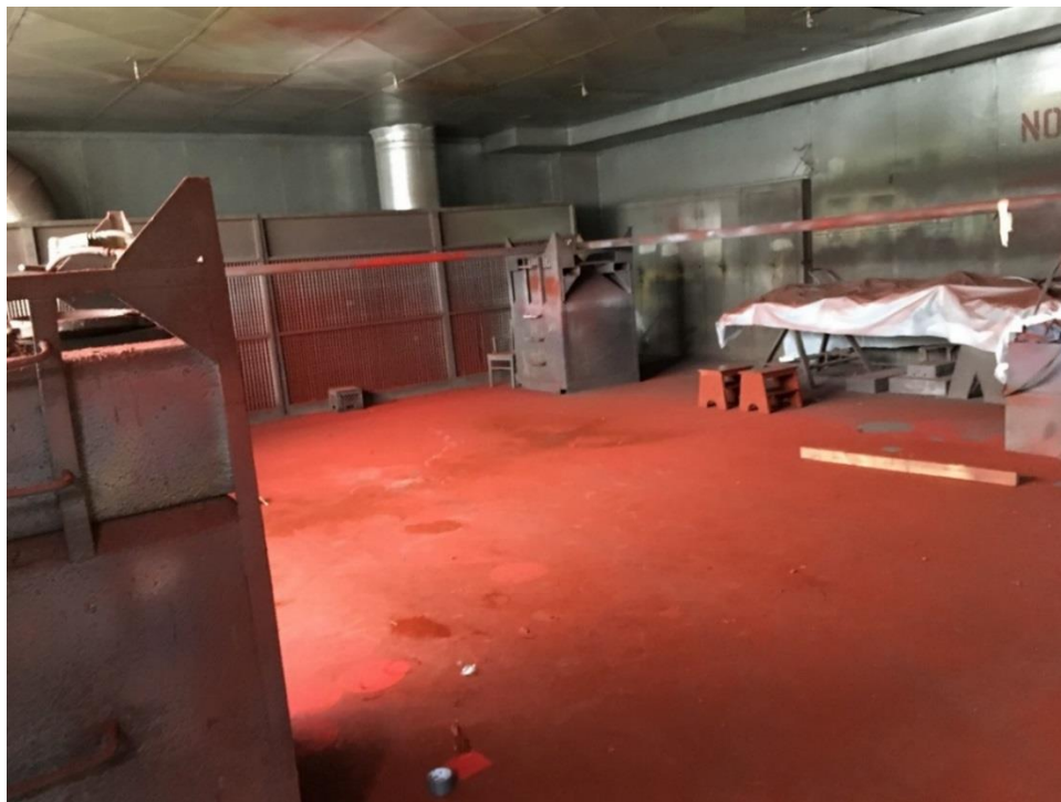
Paint Spray Booth (one of rooms in Bldg. 109) with Ventilation System
