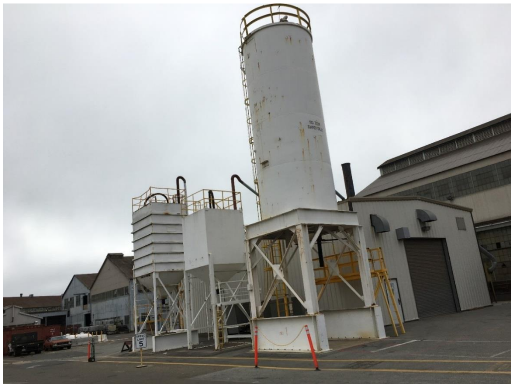
Sand Silos (3 units, largest unit is 90-ton capacity) outside Bldg. 251
