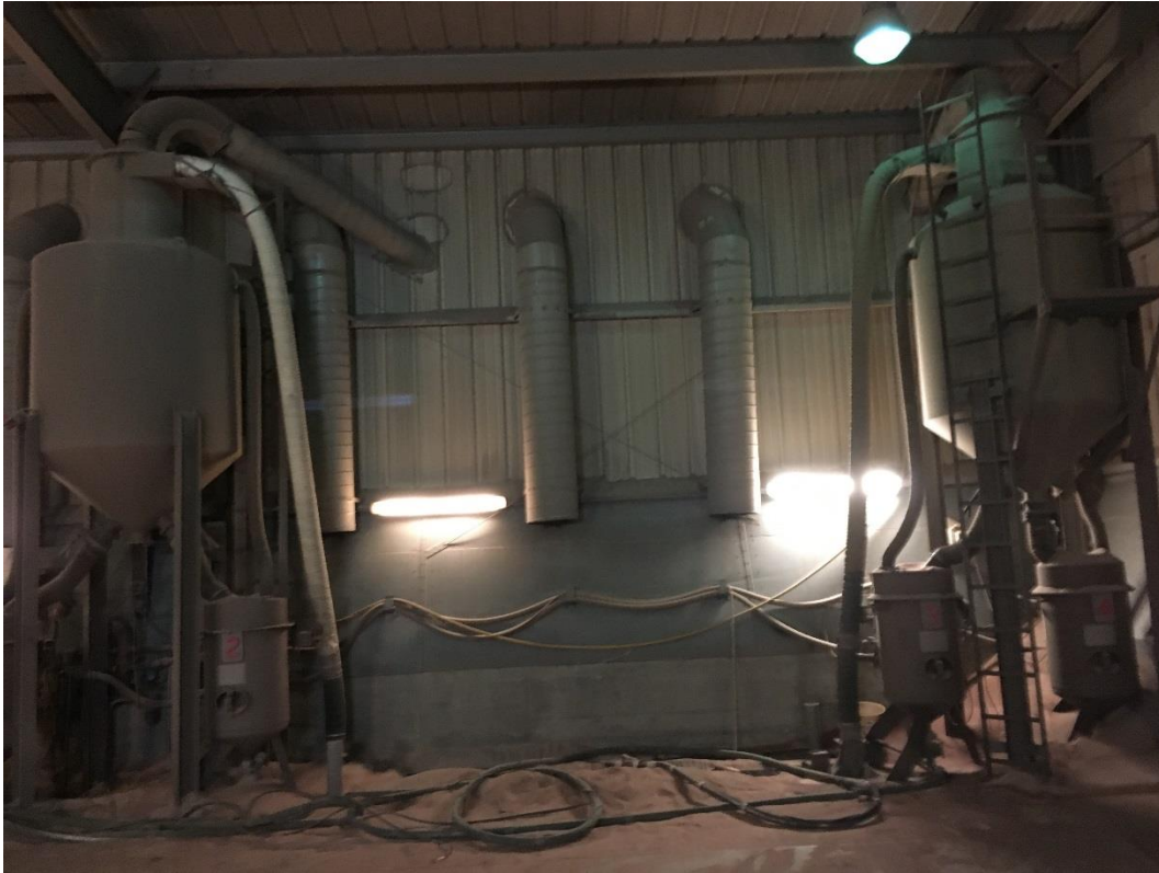
Sand Blast Equipment (inside Bldg. 251)
