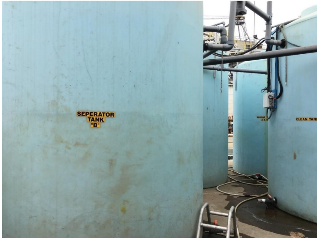
Heavy Metal & Dirty Water Separation Tanks near Bldg. 68
