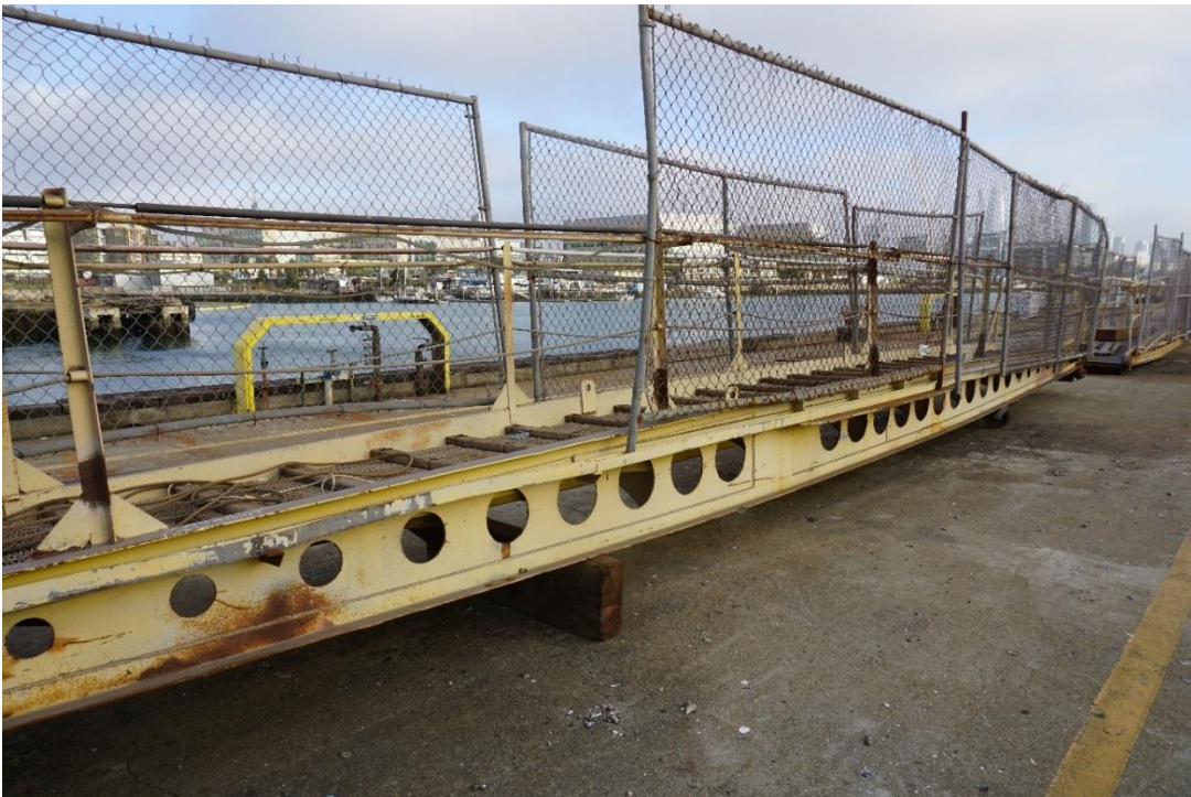
45 Ft. Gangway (Wharf 3)
