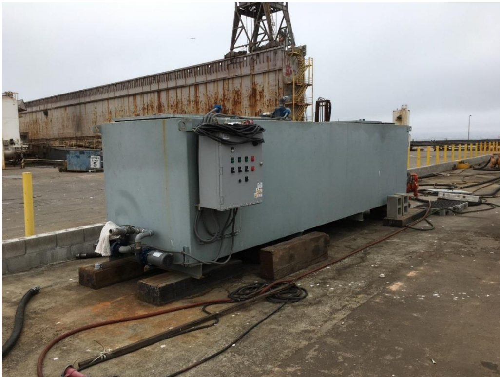
Oil – Water Separator – BW systems, PS International 2015 (near Drydock #2)
