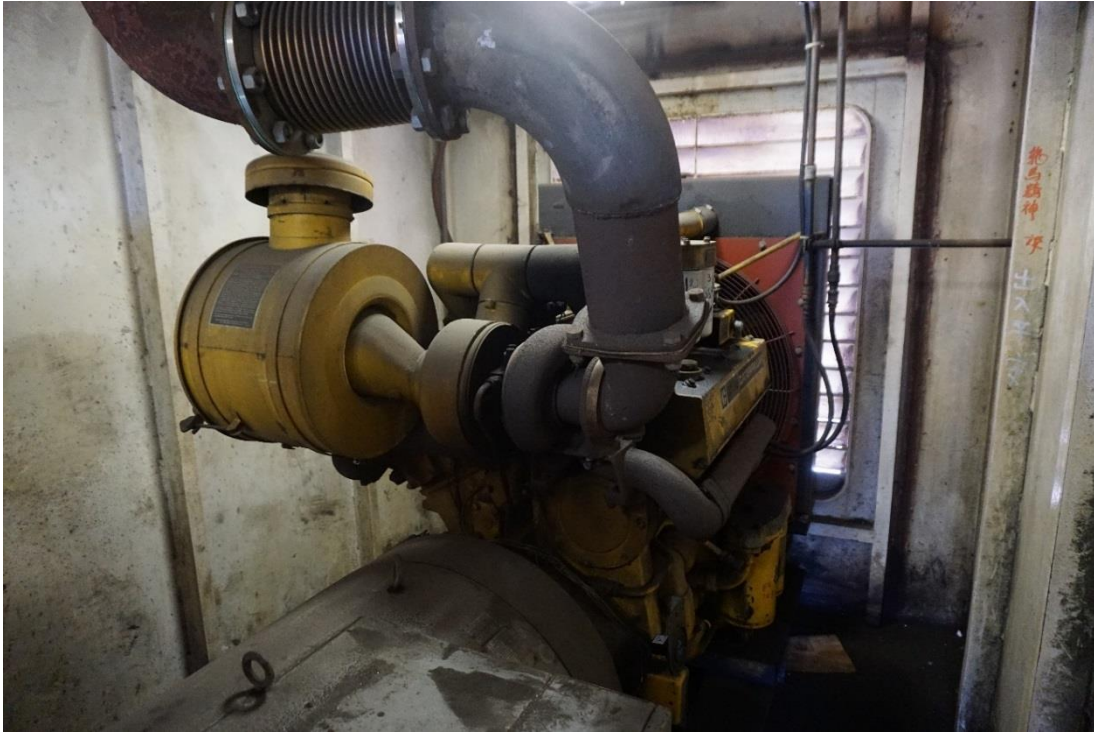
Diesel Generator 480V-300 AMP for DD #2
