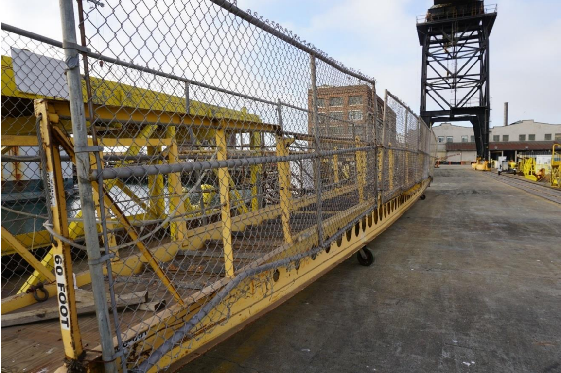
60 Ft. Gangway (Wharf 3)
