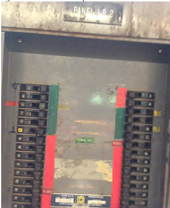
Figure 34. 100A service panel
