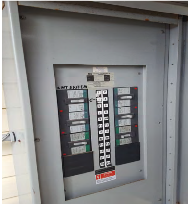
Figure 40. 225A 480V service panel
