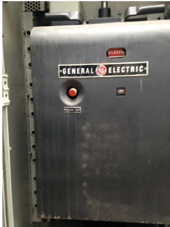
Figure 9. Substation #11 - Trip setting General Electric
