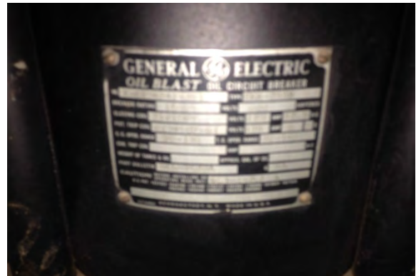
Figure 5. 50KVA Single-Phase PCB transformer nameplate
