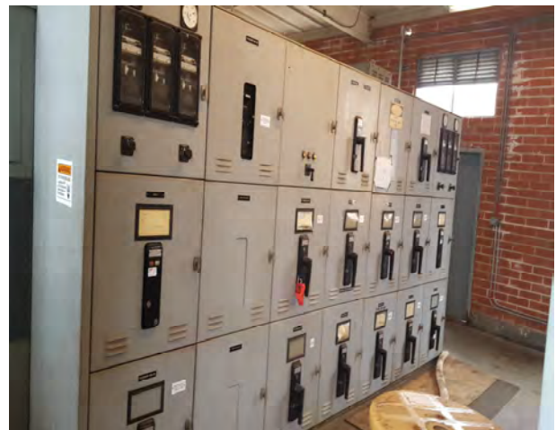
Figure 20. Substation #7A switchgear
