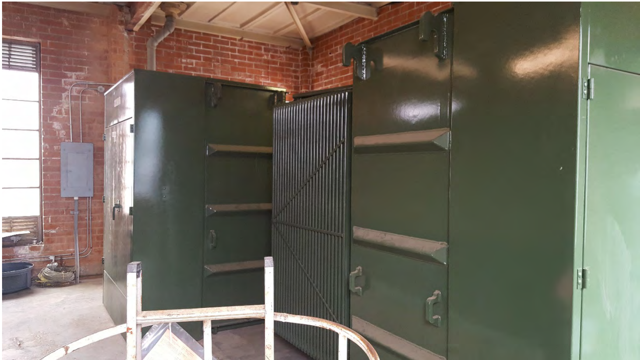
Figure 18. Substation # 7A transformers (2) 3000KVA - 12KV-480/277V
