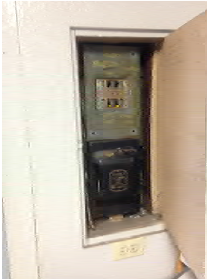
Figure 38. Power and lighting panel
