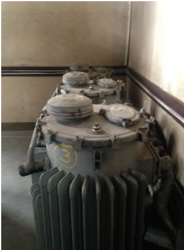
Figure 4. Three 50KVA Single-Phase PCB transformers
