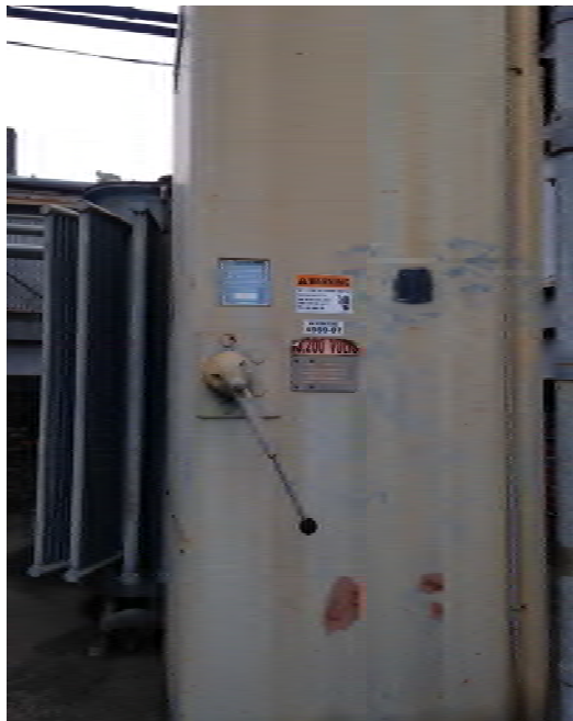
Figure 7. Substation #11 transformer - 1500KVA, 12KV-4160V
