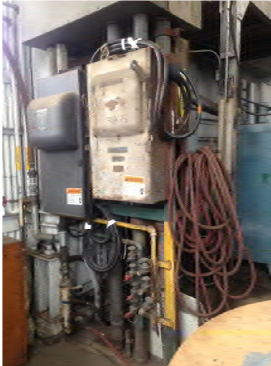
Figure 22. 400A 480V main service
