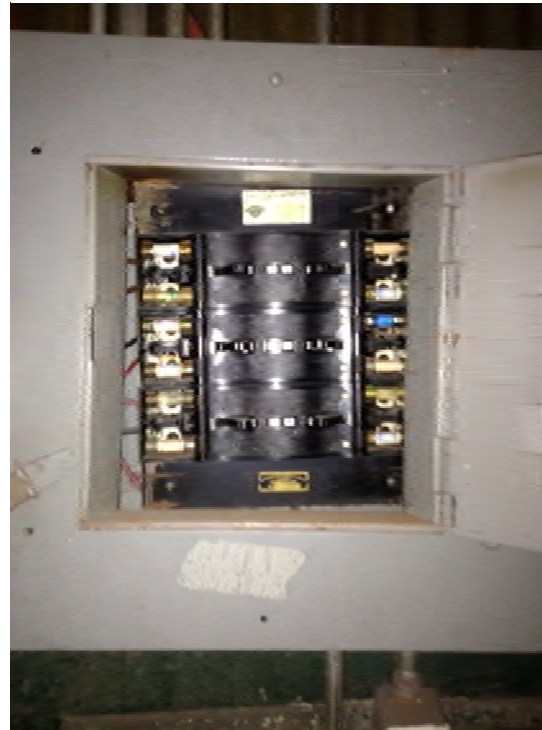
Figure 33. General electrical panel
