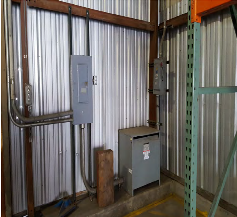
Figure 44. 100A 480V disconnect switch, 75 KVA transformer, 225A 208/120V panel
