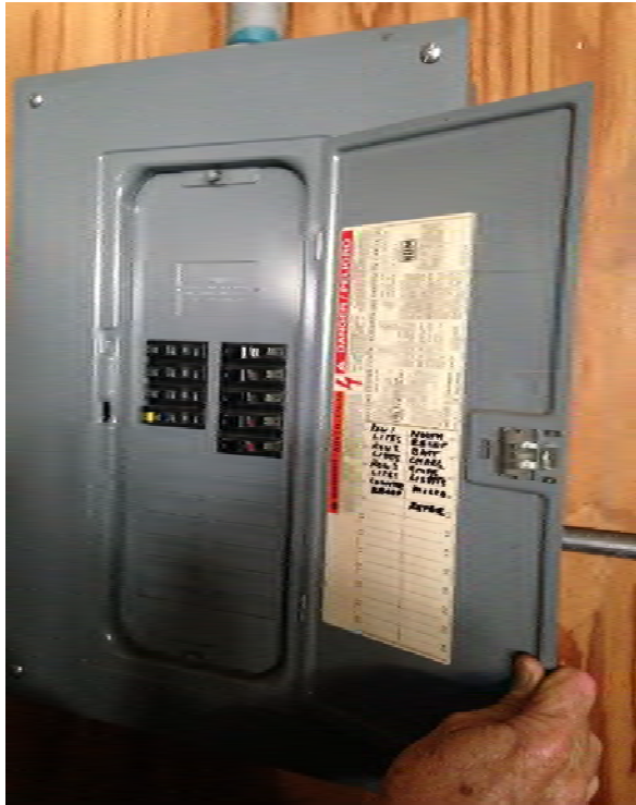
Figure 32. General electrical panel
