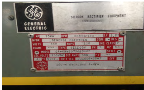
Figure 25. Nameplate for transformer
