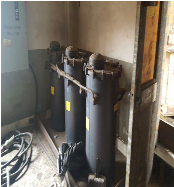
Figure 16. Three 50KVA Single-Phase PCB Transformers
