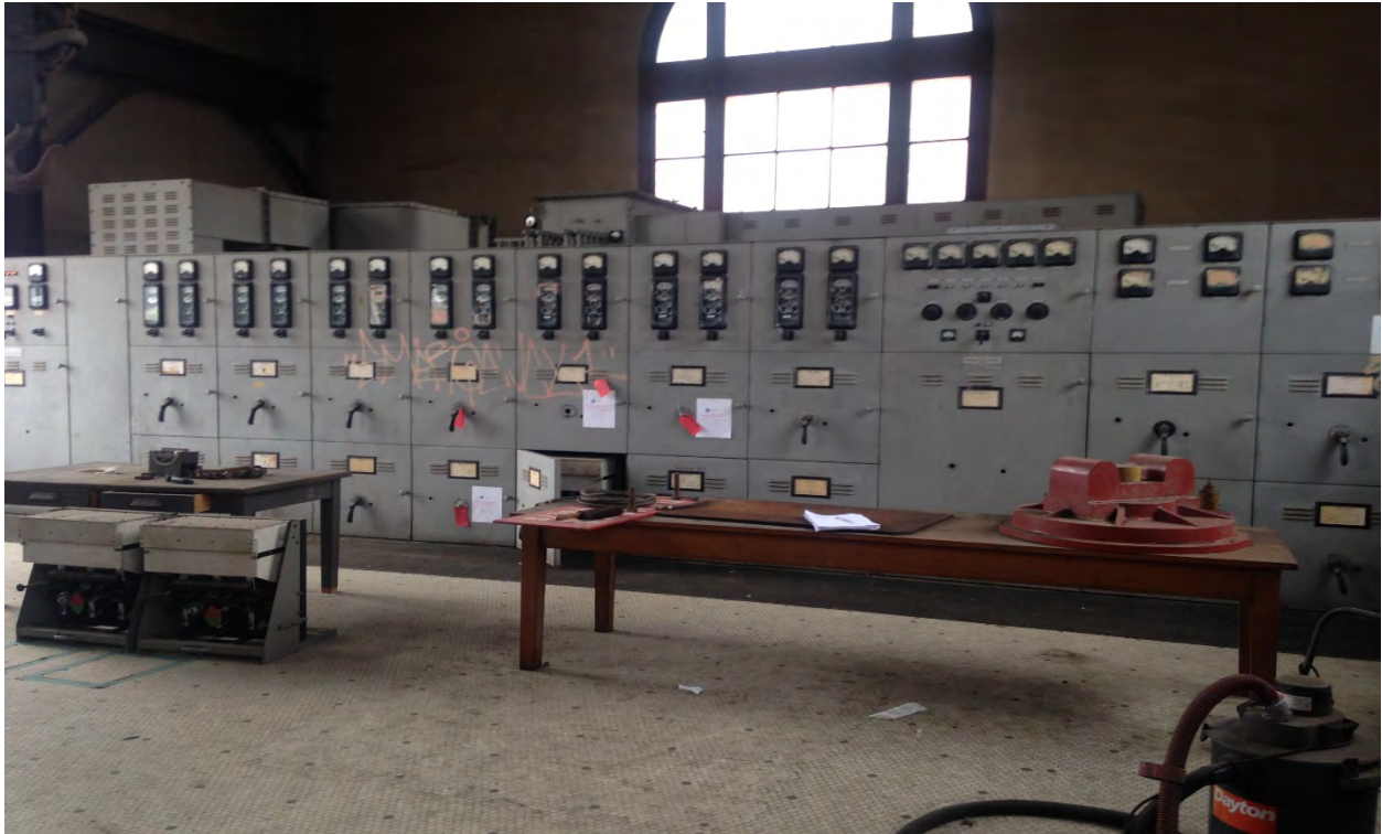
Figure 3. Building 102 second floor includes 480V Electrical Substation #1
