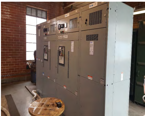
Figure 19. Substation #7A switchgear
