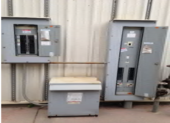
Figure 47. 400A, 480/277V panel, 45KVA transformer, 225A 208/120V panel
