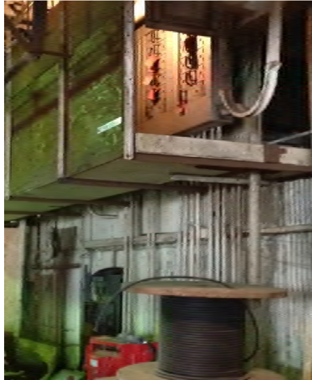
Figure 31. Power distribution system Mezzanine
