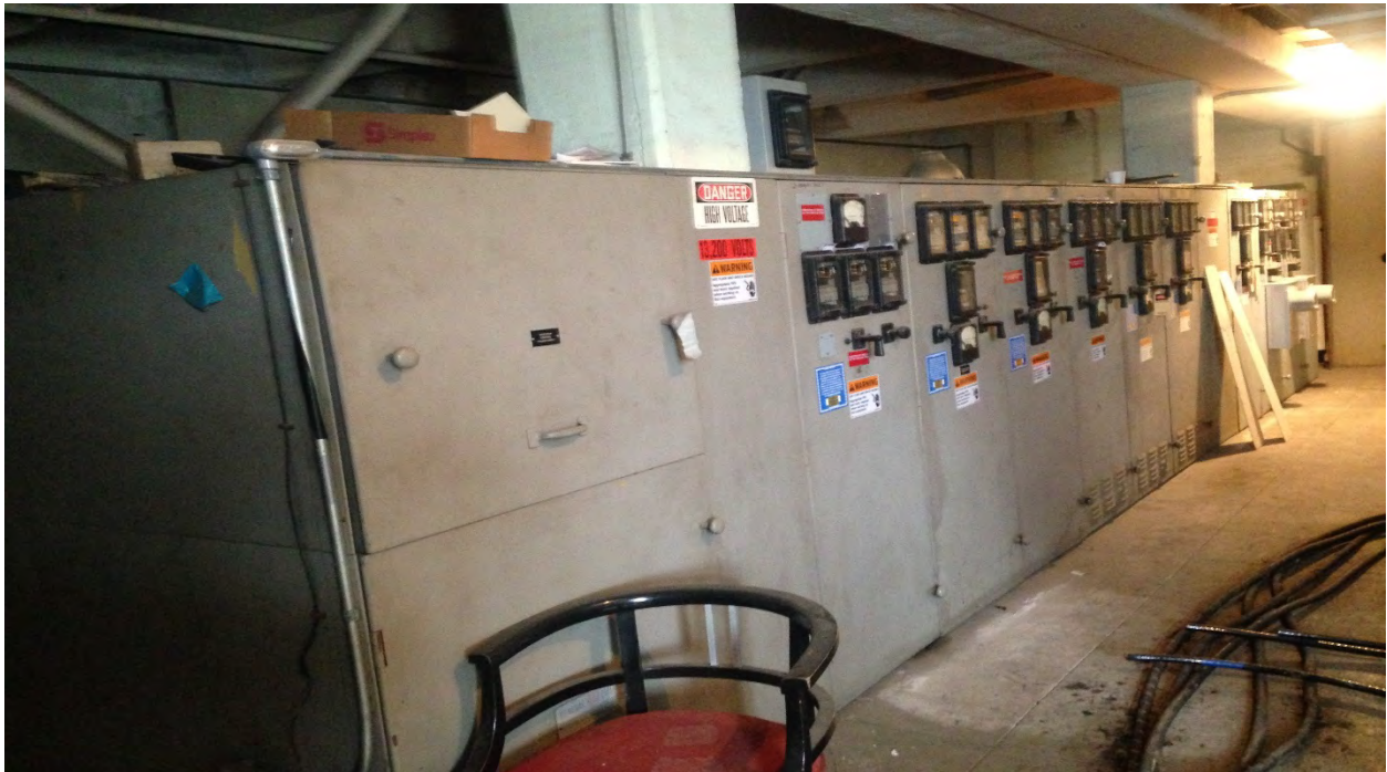
Figure 1. Building 102 first floor includes 12KV Electrical Substation #1
