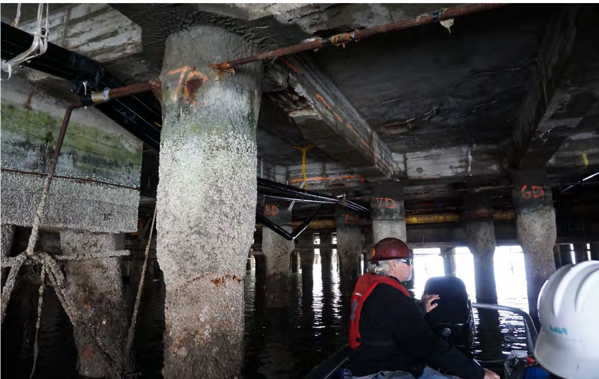
Figure 21. 3- 4" conduit 80' conduit run under Wharf (2 pictures)
