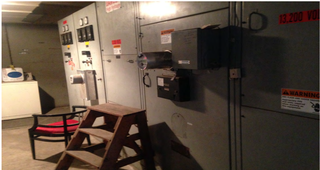
Figure 2. Building 102 first floor includes 12KV Electrical Substation #1
