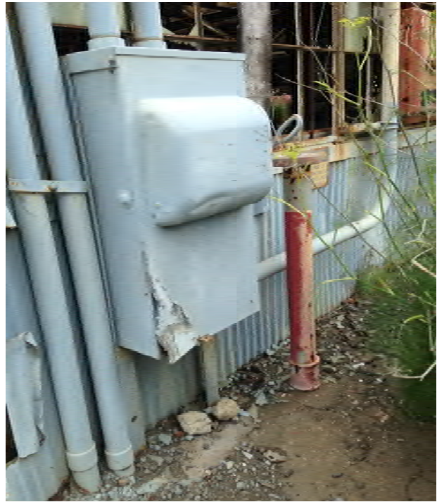
Figure 37. 400A main disconnect
