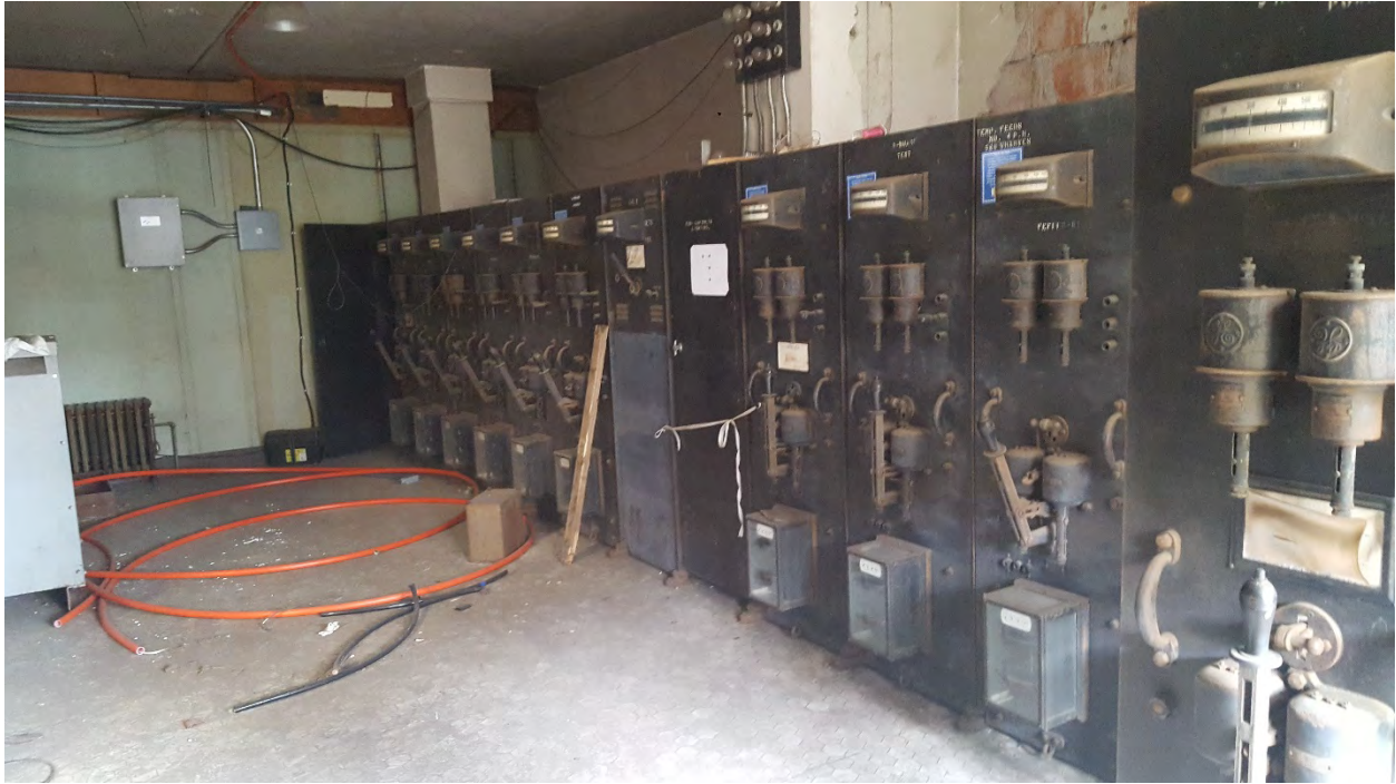
Figure 15. Substation #3 - 1000A 480 V 3P
