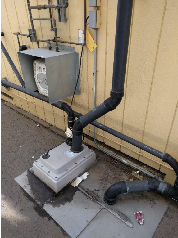
Figure 2. Medical Trailer Sewer Pump
