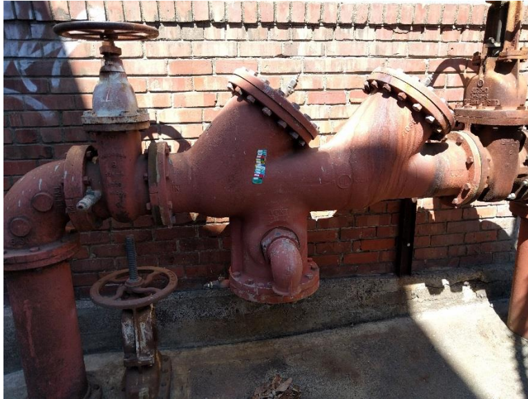
Figure 22. Main Double Detector Check Valve
