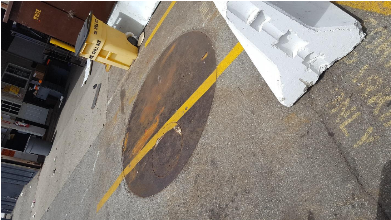
Figure 29. Sewer System CHT Pump Located Underneath the Wharf
