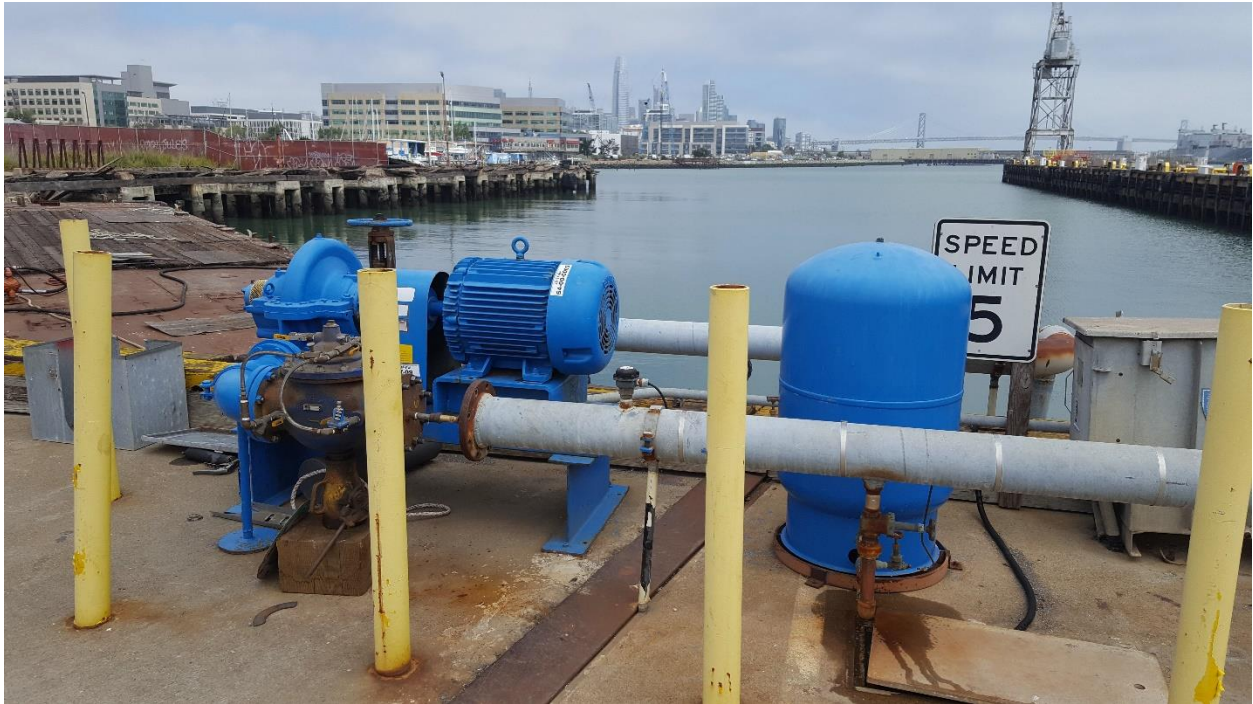
Figure 30. 75 HP Fresh Water Booster Pump
