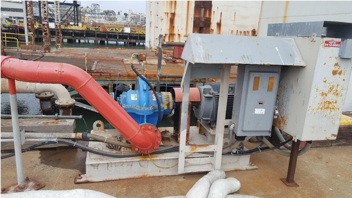
Figure 34. 100 HP Pier 4 Salt Water Pump (P4SWP)
