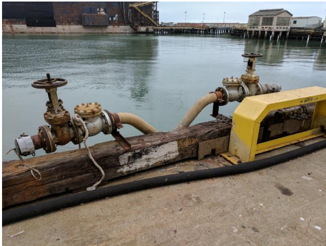
Figure 6. Sewer Ship Connection Pier 4 East
