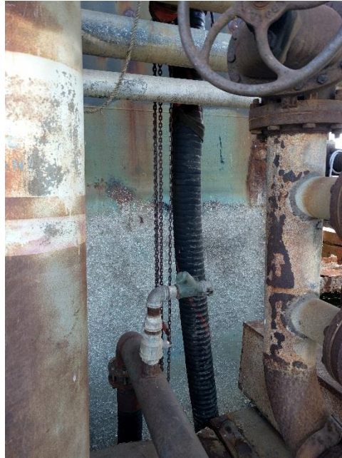
Figure 5. Highwater Platform Sewer Connection Drydock #2
