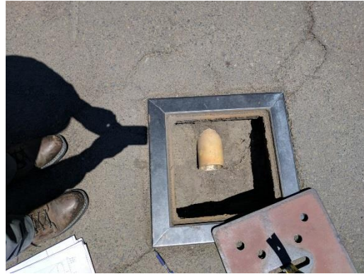
Figure 16. SD-20 Drain Inlet with Debris/Dirt and Plastic Pipe
