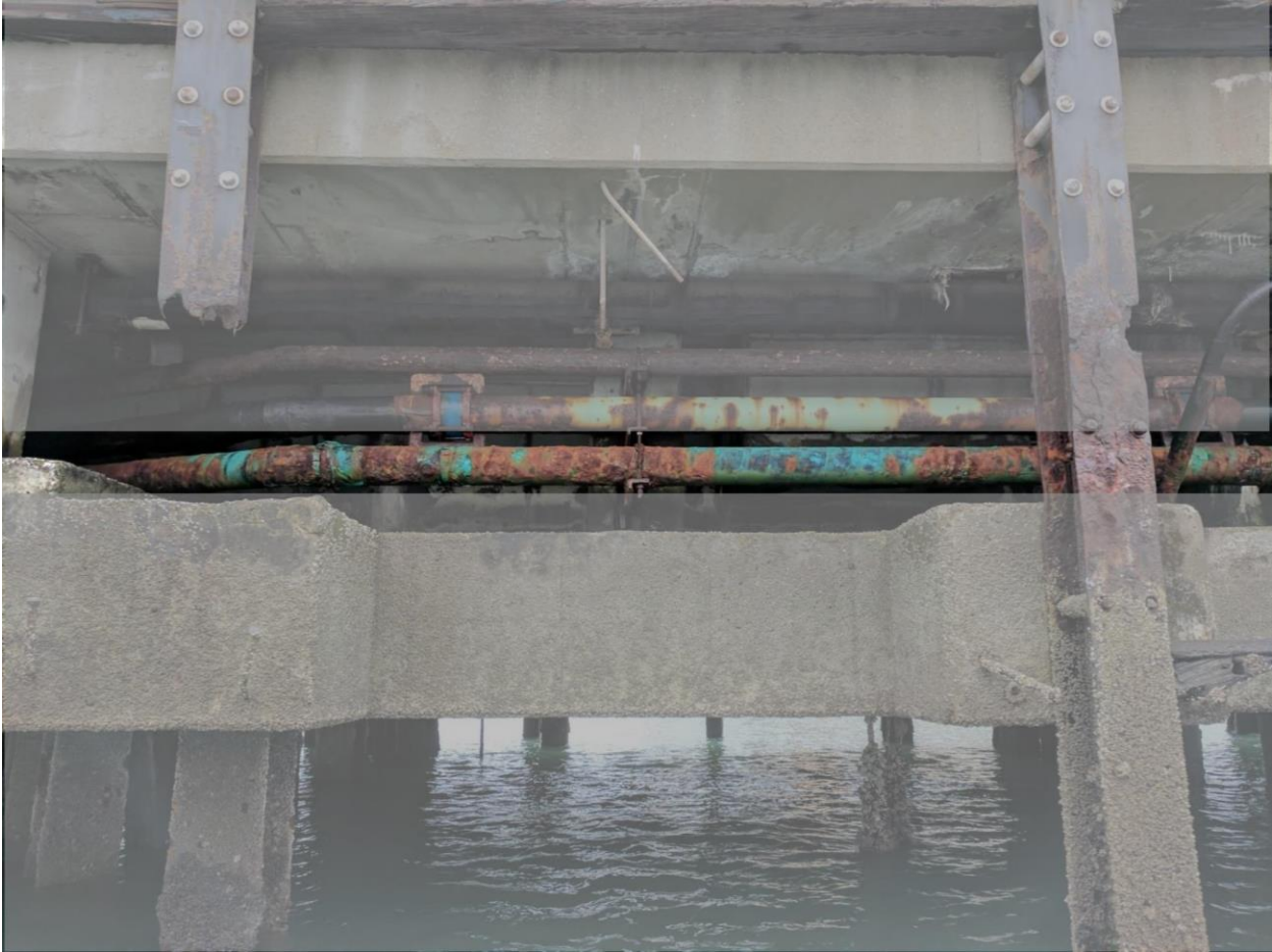
Figure 28. Salt Water Fire Protection Pipe beneath Pier
