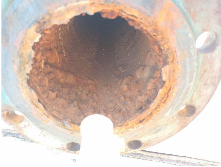
Figure 26. Fresh Water Booster Pump Pipe Rust
