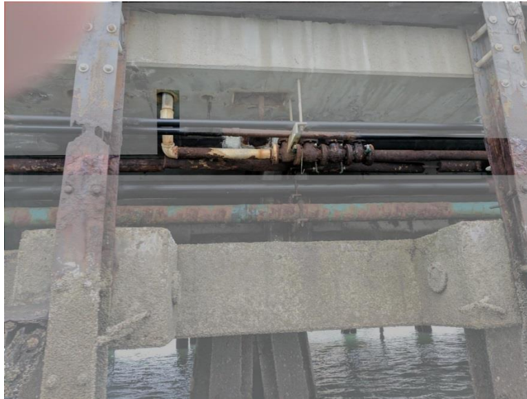
Figure 24. Fresh Water Pipe w/ DDCV at Pier 4
