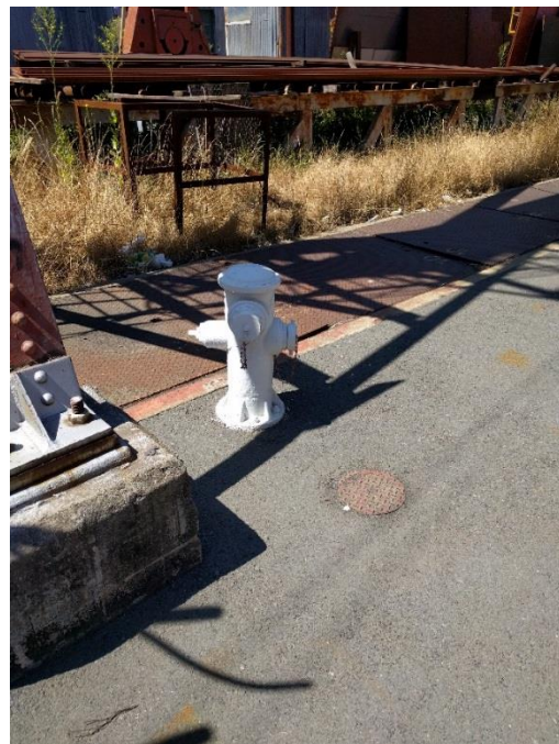
Figure 20. Typical Fresh Water Fire Hydrant
