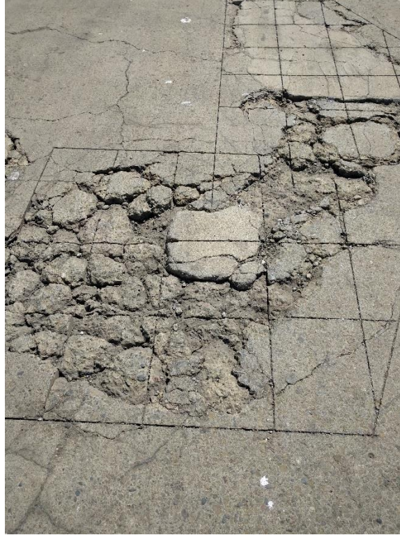
Figure 10. Wharf-side Concrete Deck Damage
