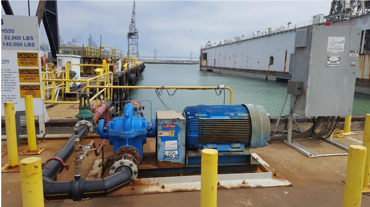
Figure 33. 250 HP Pier 3 Salt Water Pump (P3SWP)
