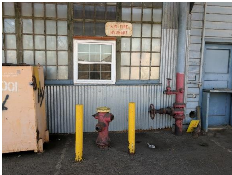
Figure 27. Salt Water Fire Hydrant
