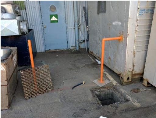
Figure 15. SD-13 Drain Inlet with Brackish Standing Water
