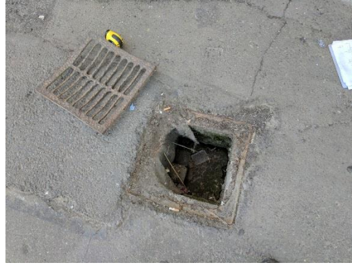
Figure 14. SD-20 Drain Inlet with Debris/Dirt
