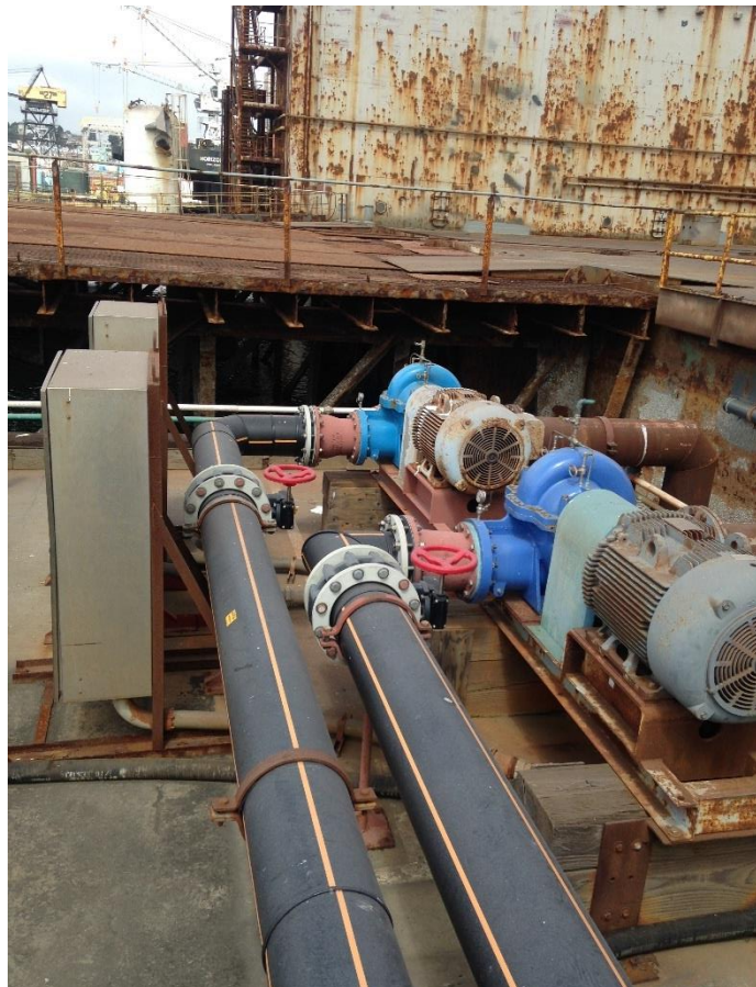
Figure 35. 125 HP Salt Water Auxiliary Cooling Pump #1 and #2 (SWACP1, SWACP2) East Pump Installed in 2002.
