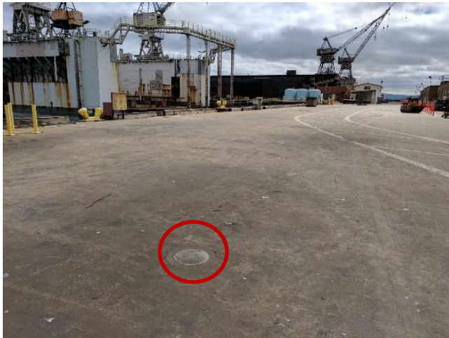
Figure 8. Wharf-side Plugged Drain
