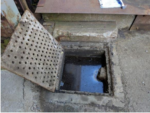
Figure 13. SD-13 Drain Inlet with Brackish Standing Water
