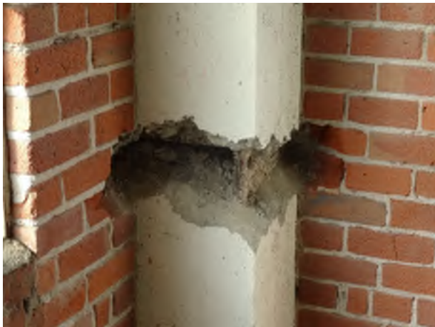
Figure 2 – Destructive testing of concrete column
