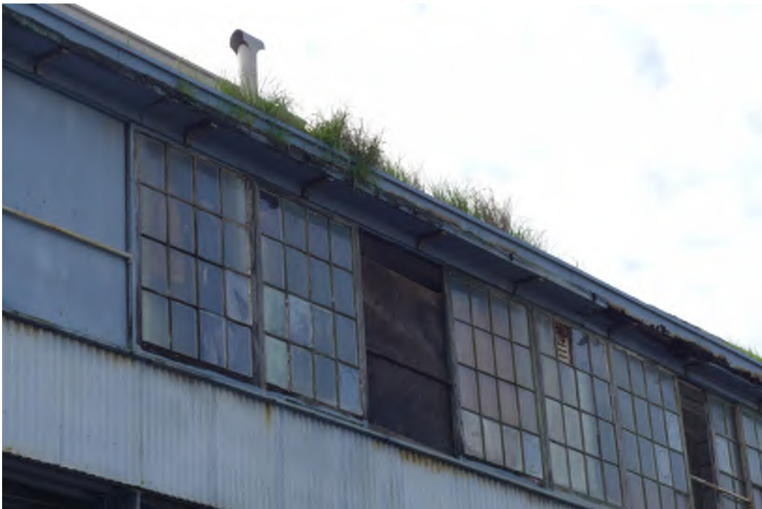
Figure 22 - Building 109, Mold loft windows, north elevation. Note gutter condition.
