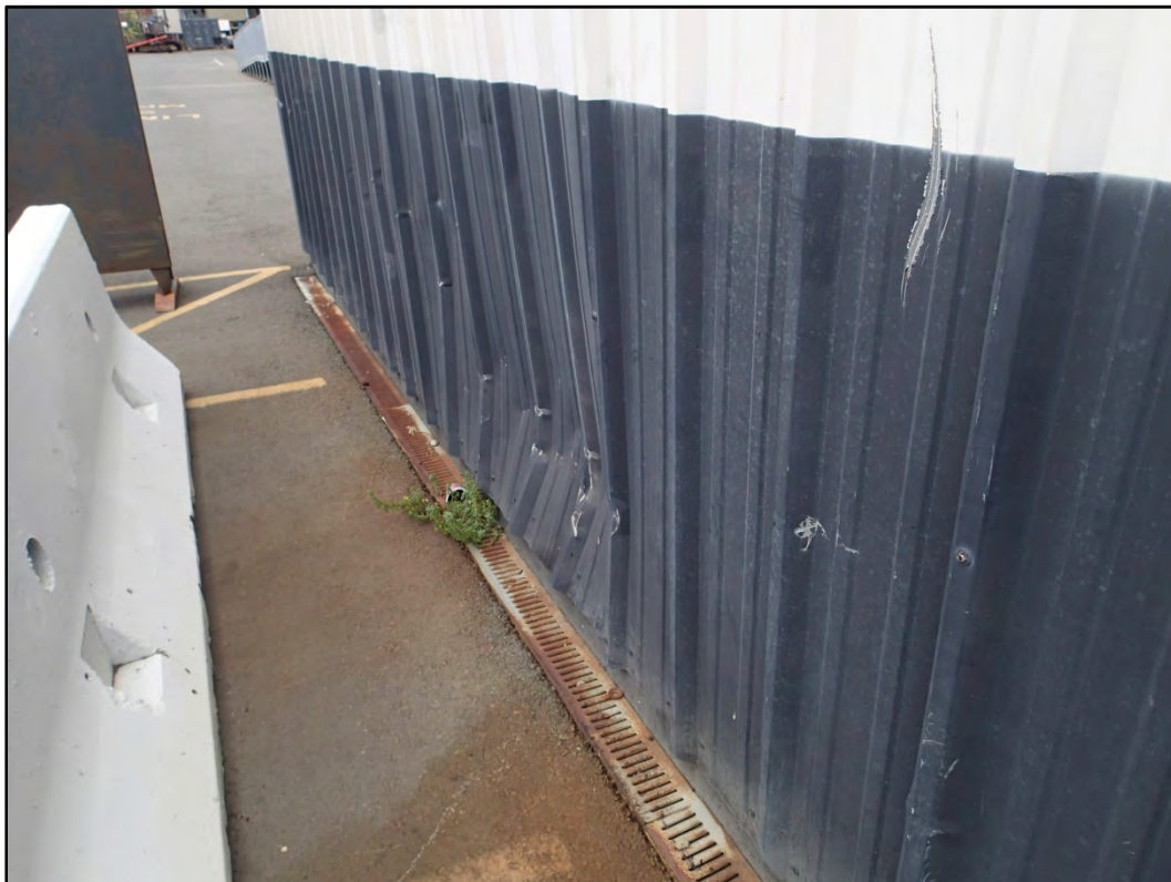
Figure 250-5 – View of the existing impact damage to the south wall at Building 250.
