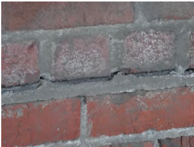
Figure 4 – Partial height masonry wall mortar damage
