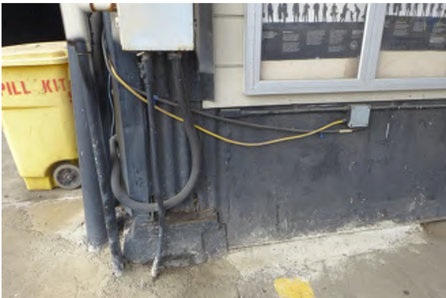
Figure 12 - Building 109, CMP damage at Tool Room, south east corner
