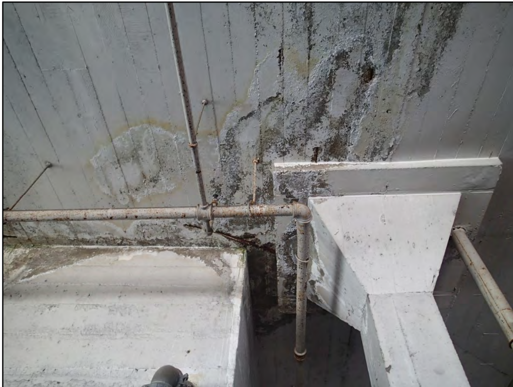
Figure 111-14 – View of fifth floor interior ceiling efflorescence in Building 111.
