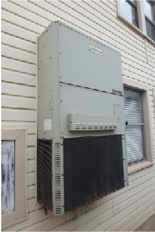
Figure 127-1 – Wall-mounted Heat Pumps
