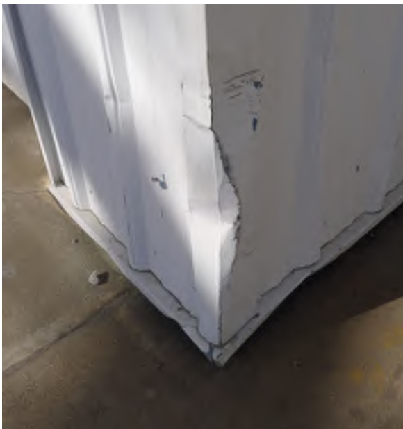
Figure 5 - Damaged southeast corner
