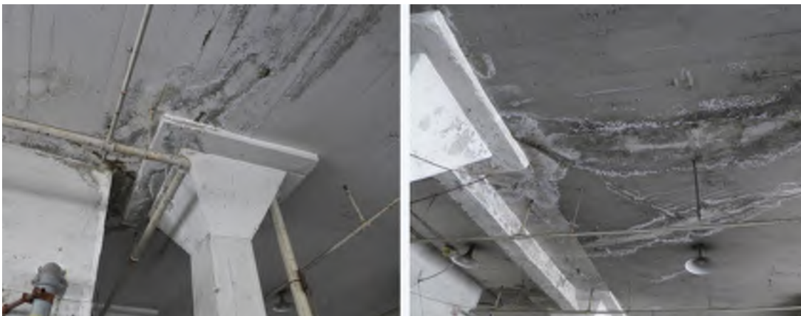
Figure 36 - Building 111, fourth floor ceiling
