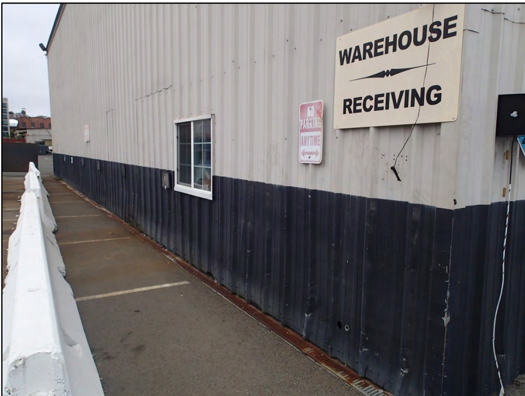
Figure 250-3 – View of the typical condition of the corrugated metal panels at Building 250.
