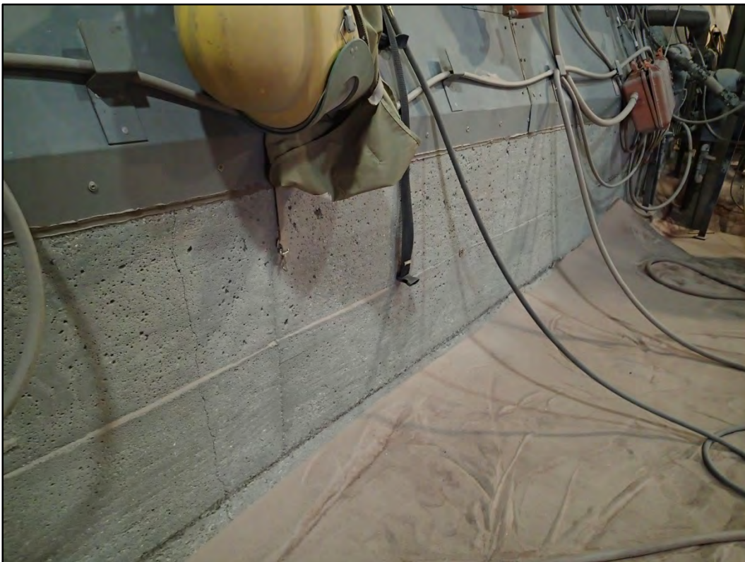
Figure 251-10 – View of the interior concrete stem wall along the north and south sides of Building 251.
