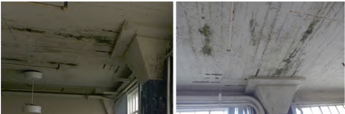
Figure 34 - Building 111, second floor ceiling
