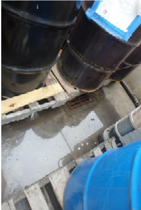
Figure 110-2 – Standing Water Inside Chemical Storage Sump at the Drain.
