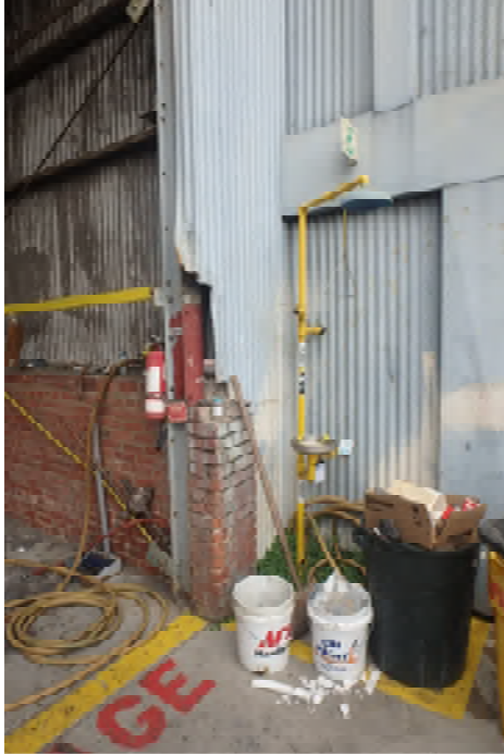
Figure 110-1 – Eyewash and Shower Facilities
