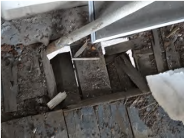
Figure 4 – Typical 2 nd floor damage at 2 nd floor punchout
