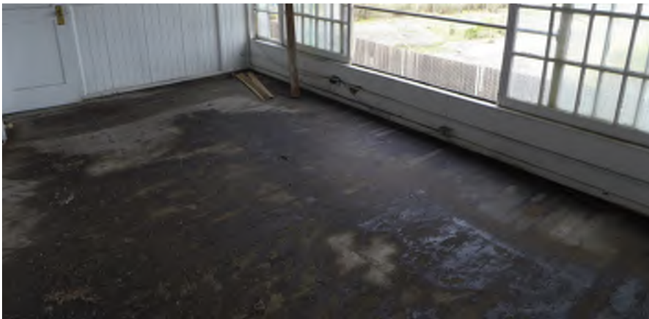
Figure 24 - Building 109, wood T&G floor. Note water from deteriorated gutter condition.
