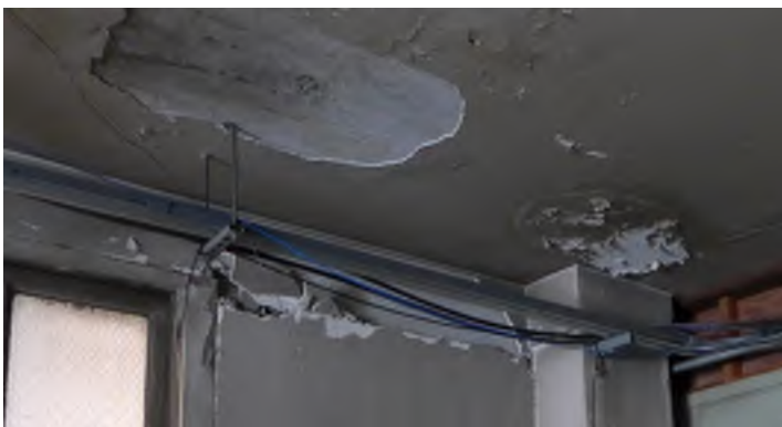
Figure 32 - Building 111, first floor substation # 3 ceiling
