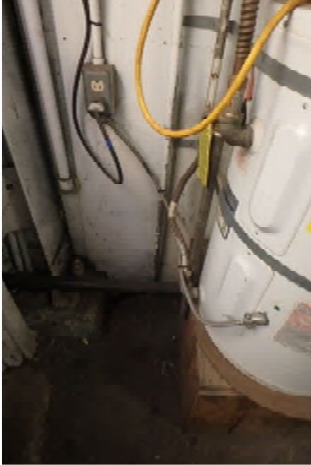
Figure 109-5 – Electric Water Heater Wired without Disconnect
