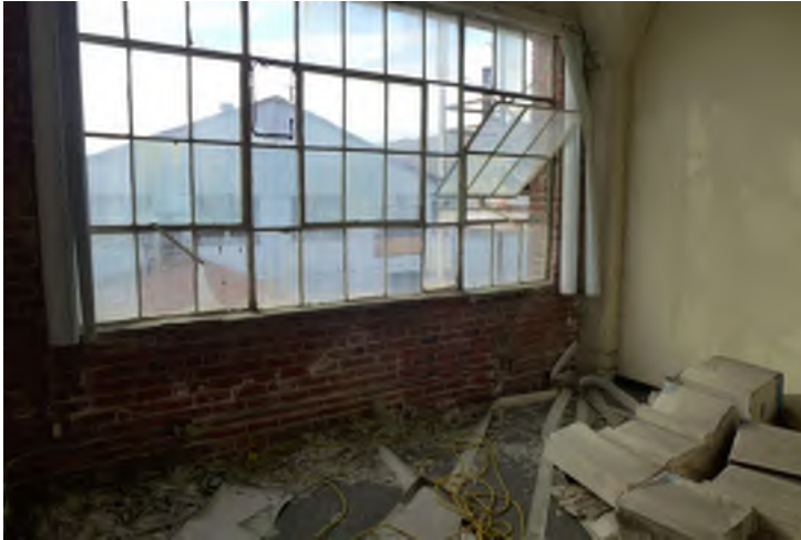
Figure 29 - Building 111, second floor exterior wall. Note moisture damage.
