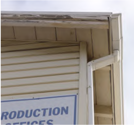
Figure 5 - Paint deterioration at fascia and eaves.
