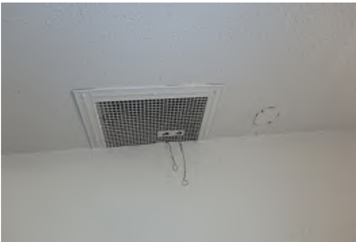
Figure 121-2 – Operable Ceiling Vents
