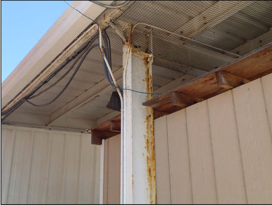
Figure 143-4 – View of the minor surface corrosion on the structural steel members at Building 143.
