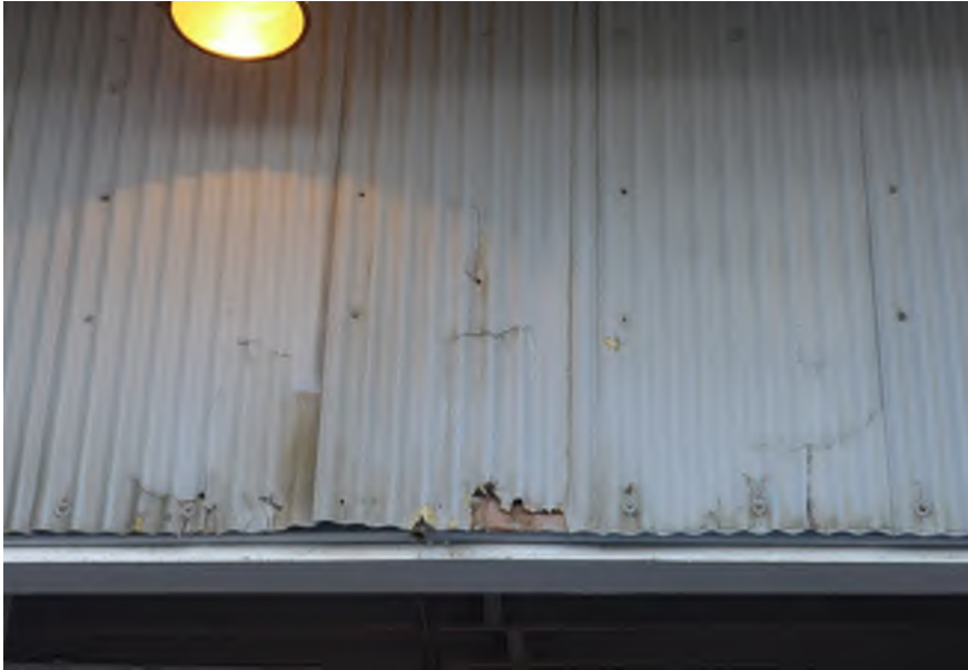
Figure 11 - Building 109, CMP damage at north elevation doorway.
