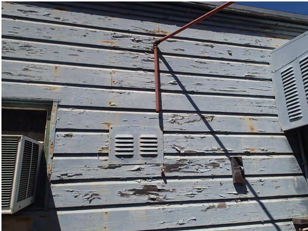
Figure 121-6 – View of the typical paint deterioration on the exterior of Building 121.
