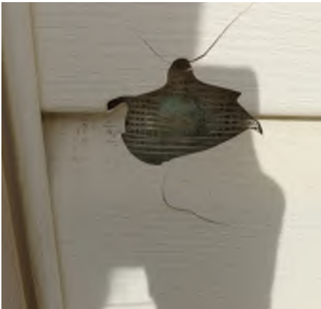
Figure 5 – Puncture damage to vinyl siding
