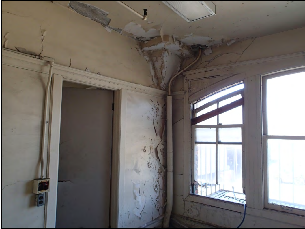
Figure 111-13 – View of typical interior paint deterioration in Building 111
