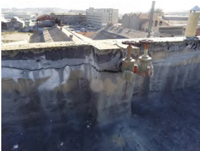
Figure 3 – Typical parapet cracking
