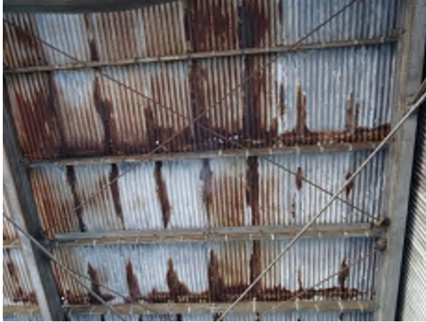
Figure 1 – Typical rusting to roof CMP
