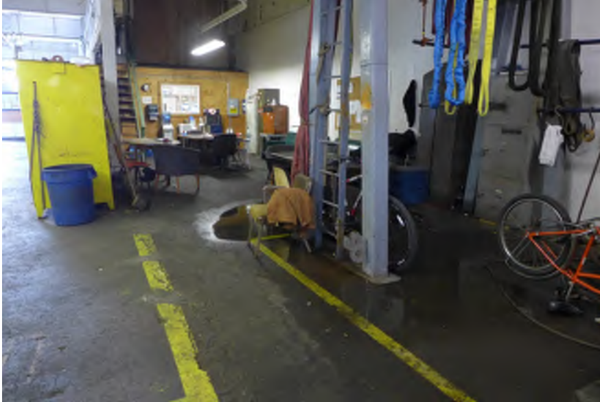
Figure 17 - Building 109, Asphalt Floor at Rigging/Break Room. Note ponding.
