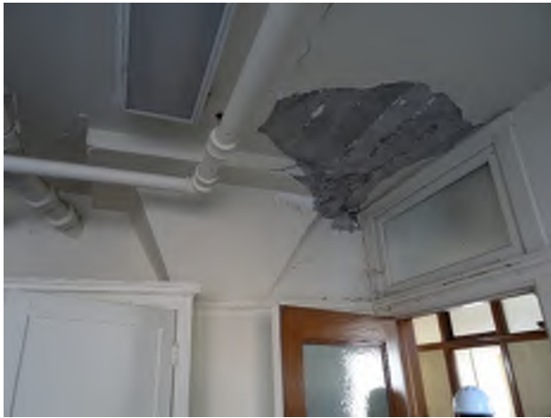
Figure 1 – Concrete capital damage
