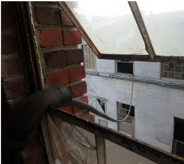
Figure 111-4 – Flexible Cable Feeding Power from Neighboring Building
