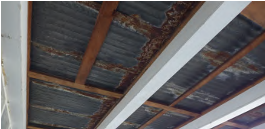
Figure 25 - Building 109, Mold loft CMP ceiling.
