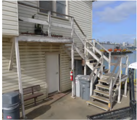
Figure 6 - Paint deterioration at second floor entry stair.
