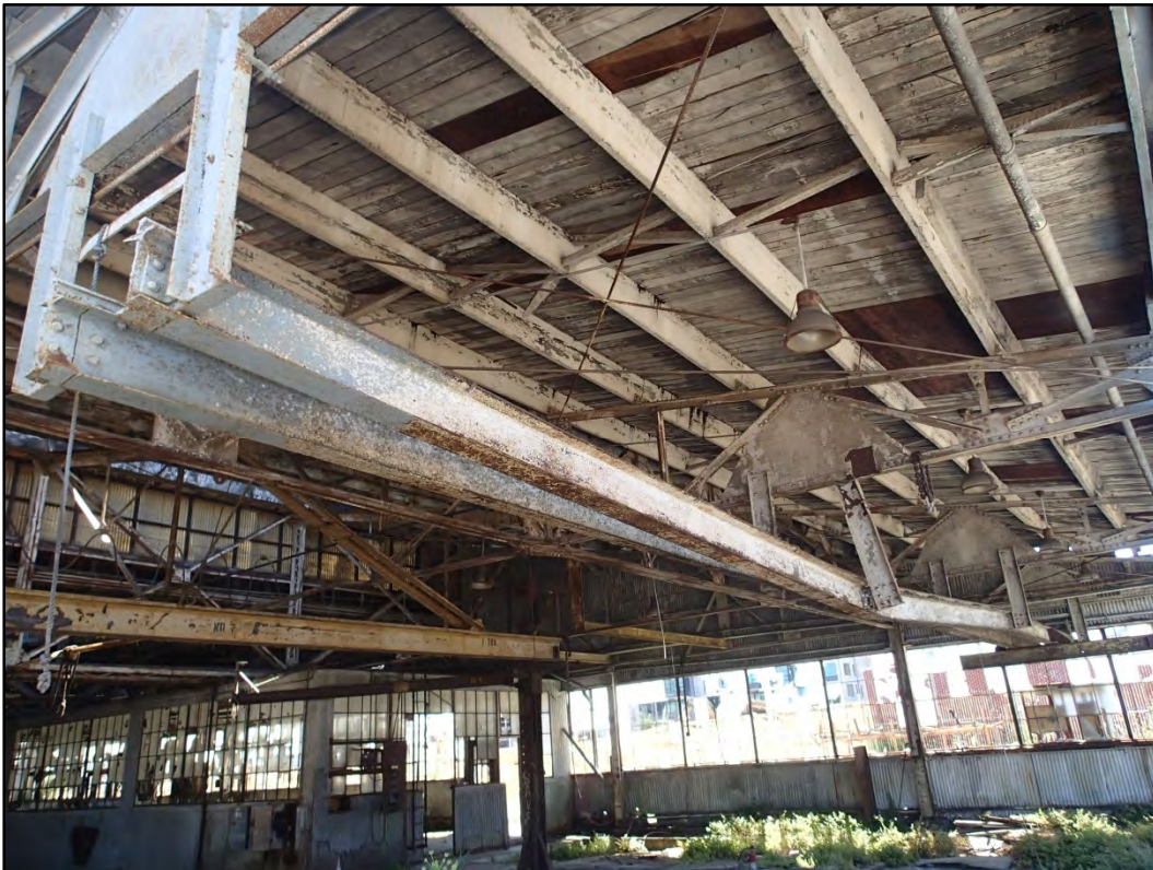
Figure 109-13 – Overall interior view of the abandoned west section of Building 109.
