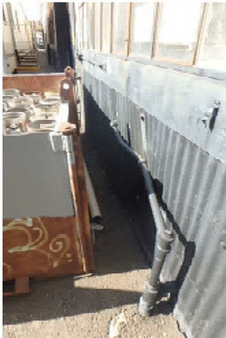
Figure 109-4 – Waste pipe bent & damaged from collision.
