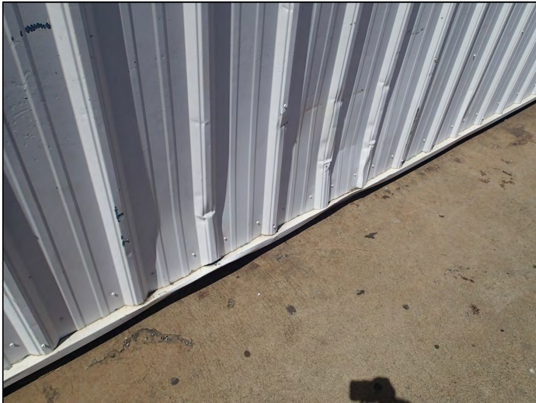
Figure 143-3 – View of previous damage to corrugated metal wall panel at Building 143.
