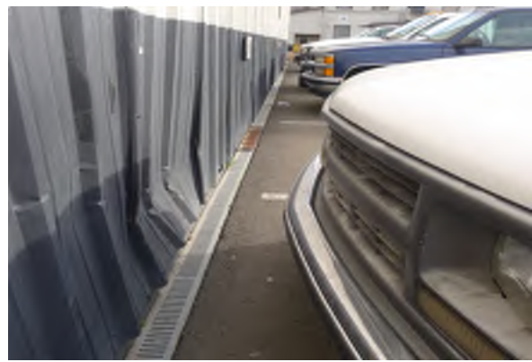
Figure 3 - Damage to the south wall caused by vehicles
