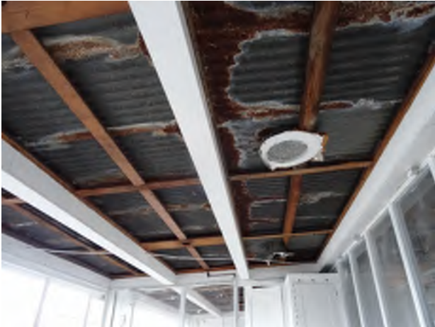
Figure 3 – Typical roof damage at 2 nd floor punchout
