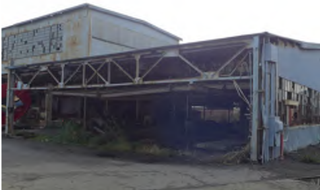
Figure 3 - Building 109, the north side of this portion of the building is open.
