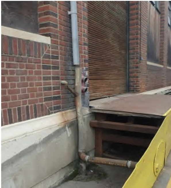
Figure 111-3 – Damaged Rainwater Leader
