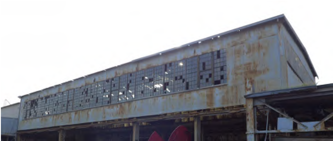
Figure 4 - Building 109, western section of building, north wall. Wood windows at second story.
