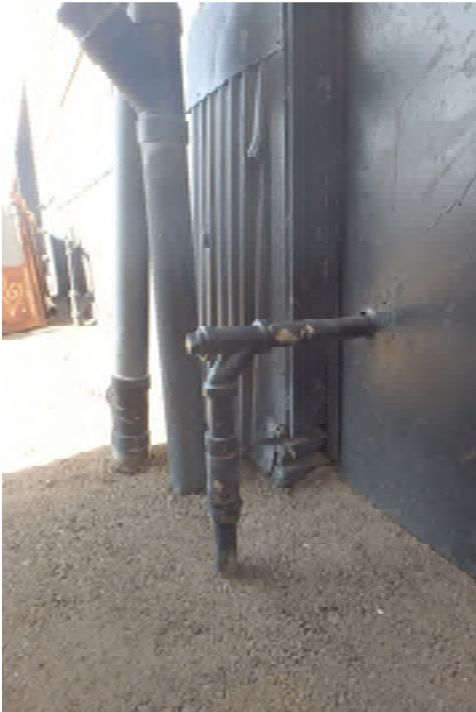
Figure 109-2 – Cleanout on drain installed backwards.
