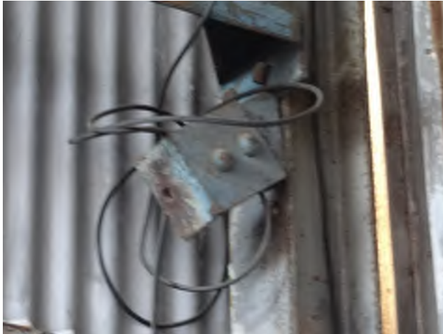
Figure 3 – Missing tension “x” brace
