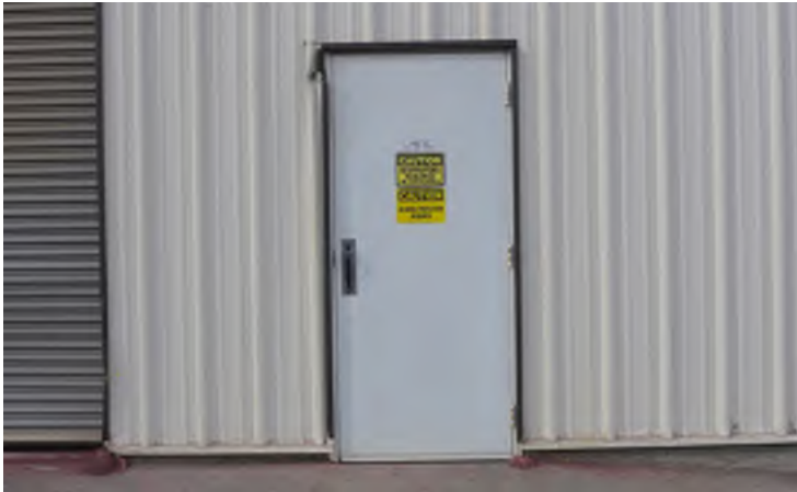
Figure. 4 - Building 250: East personnel door. Note damage at door trim.
