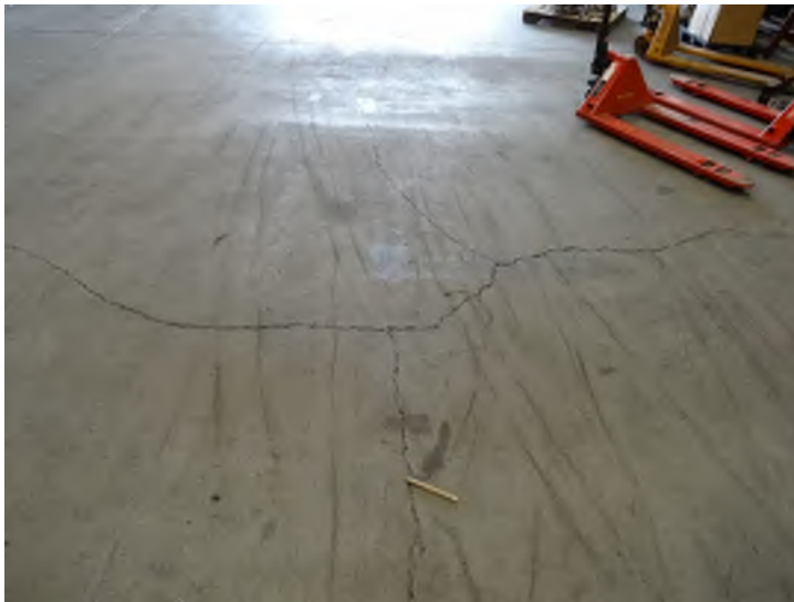
Figure 2 – Typical slab on grade cracks
