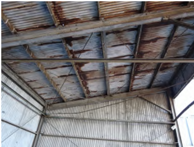
Figure 2 – Typical corrosion on steel members
