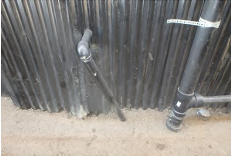
Figure 109-3 – Plumbing Pipe damaged from building shifting.
