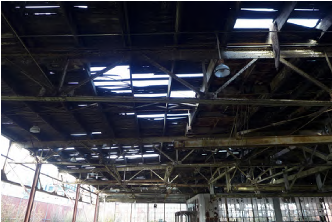
Figure 6 - Building 109, western section of building, looking west. Note missing wood T&G ceiling.
