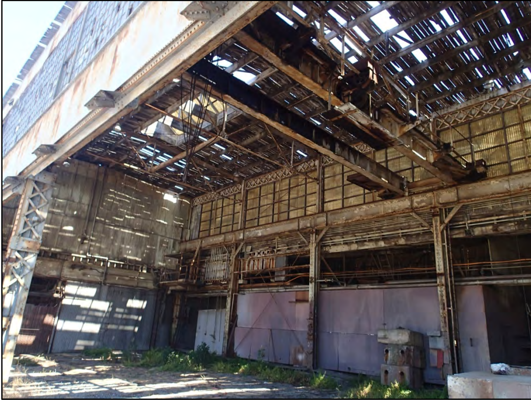
Figure 109-12 – Overall interior view of the abandoned west section of Building 109.
