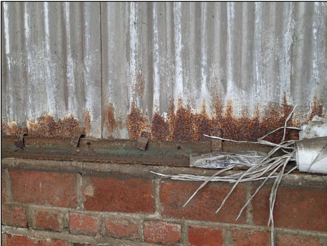
Figure 120-5 – View of the corrosion along the bottom edge of the interior corrugated metal wall panels.
