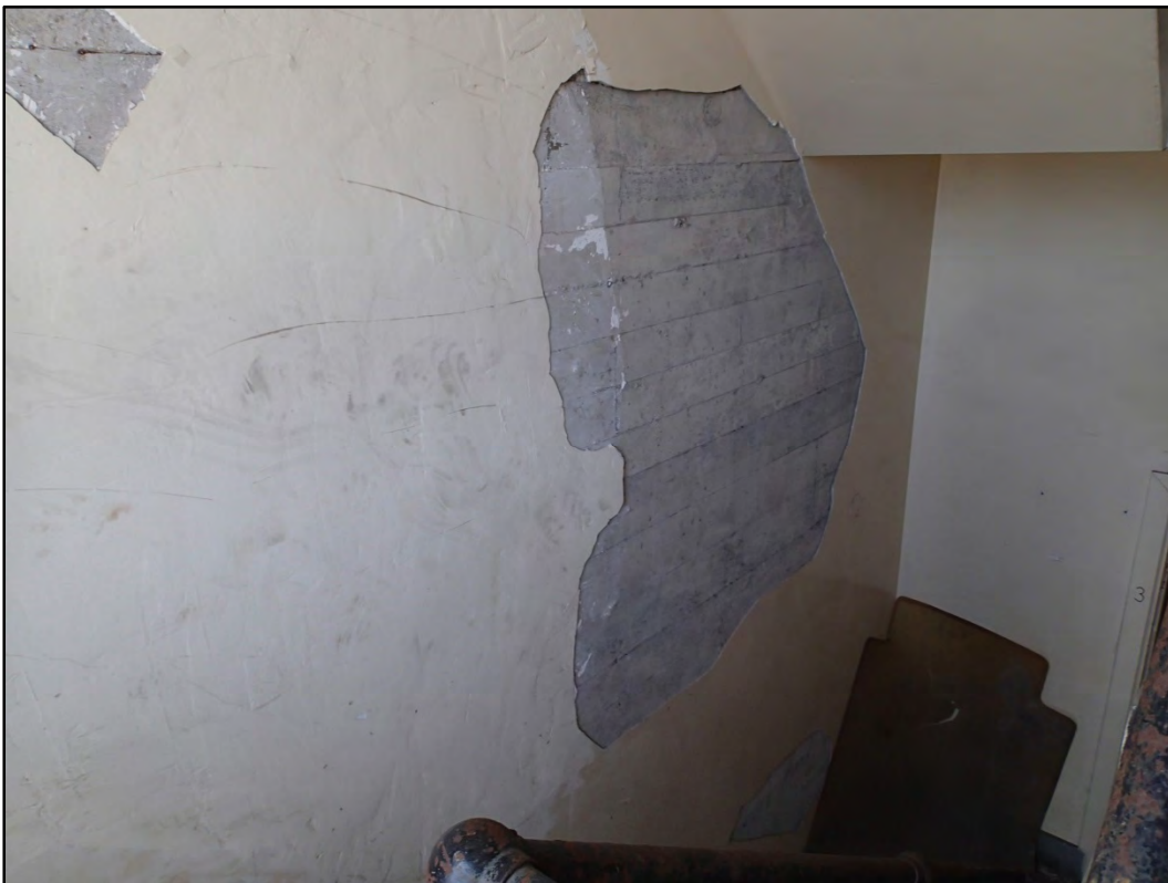
Figure 111-12 – View of typical interior plaster damage in Building 111.
