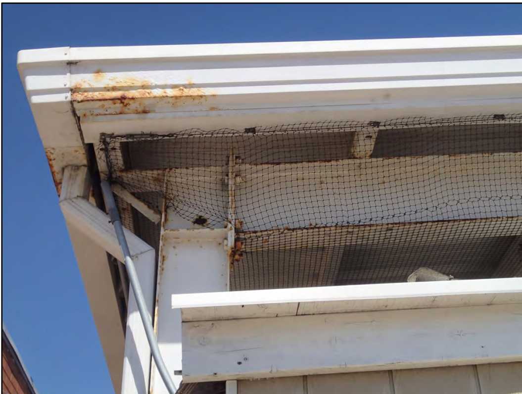
Figure 143-5 - View of the surface corrosion on the structural members and gutters at Building 143.
