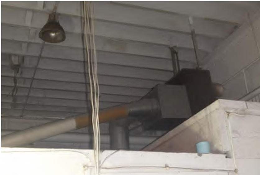
Figure 109-1 – Unit heater with ducted discharge. Possible noxious gas hazard from burning fuel.
