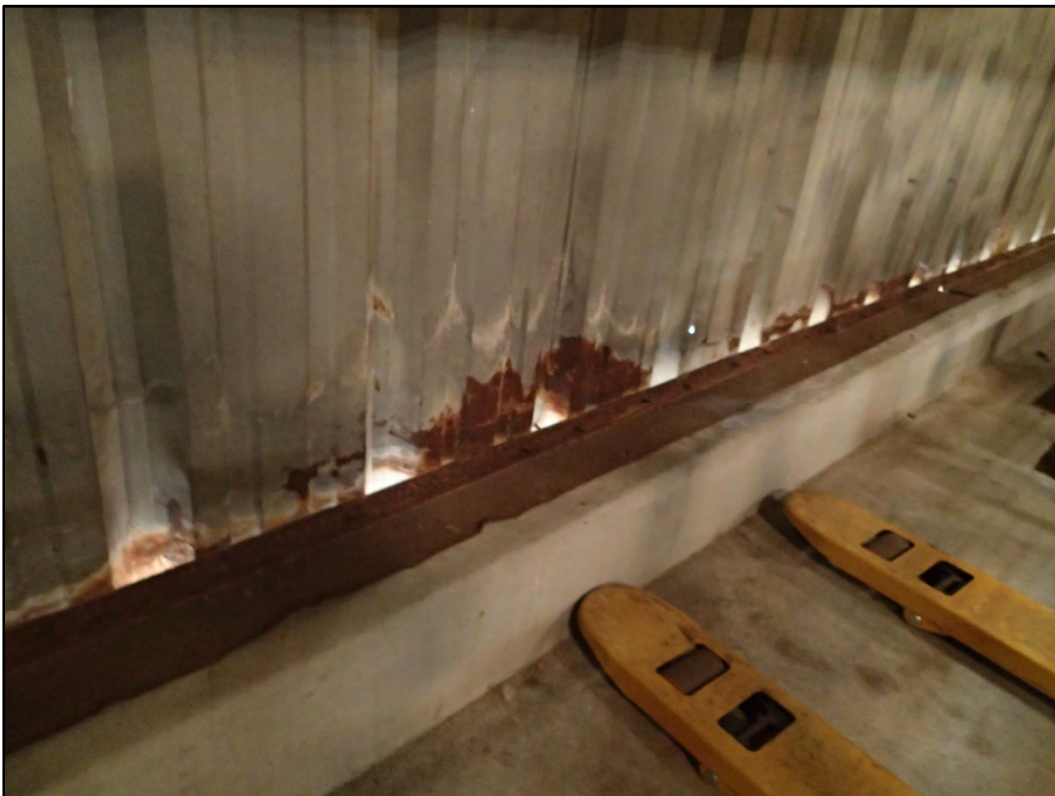
Figure 250-9 – View of the minor to moderate corrosion along the bottom of the corrugated metal panels.
