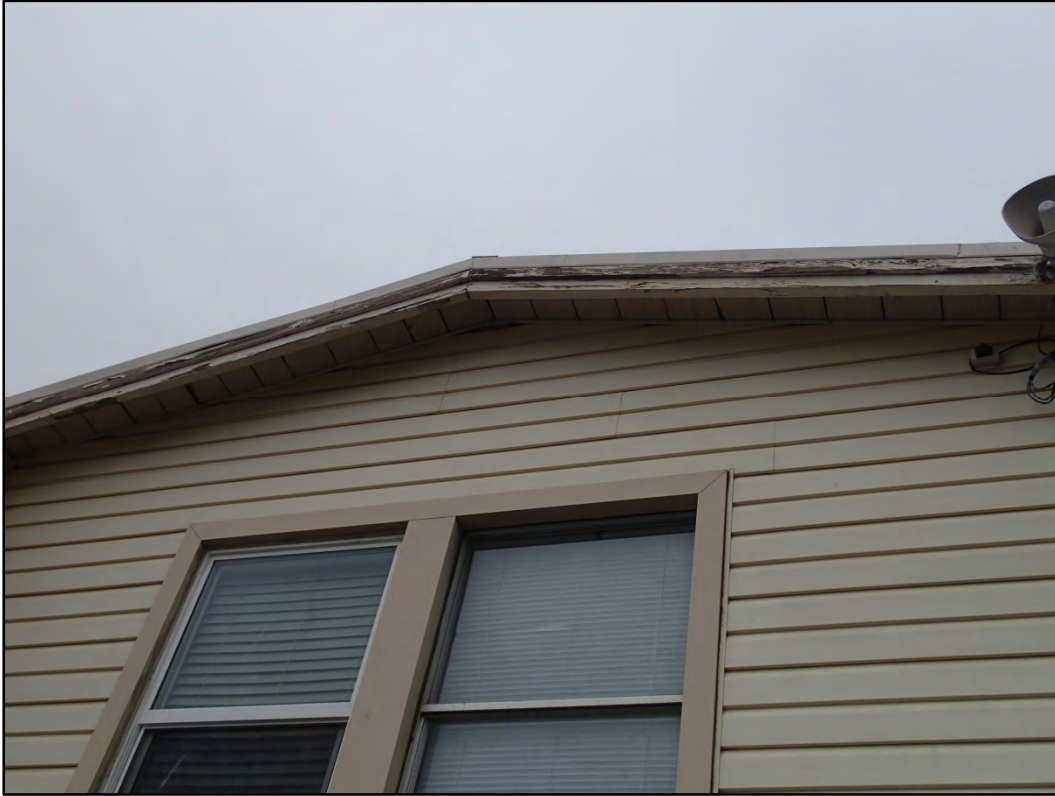
Figure 127-5 – View of the existing paint deterioration on the fascia and eaves at Building 127.
