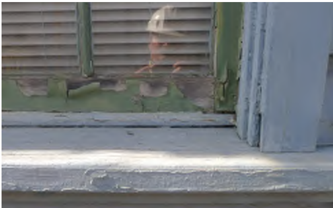
Figure 5 - Building 121: Windows detail. Poor paint and missing glazing putty.
