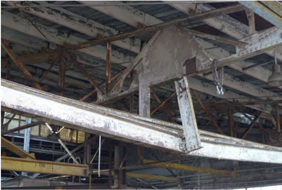
Figure 7 - Building 109, western section of building. Note collapsed steel beam.
