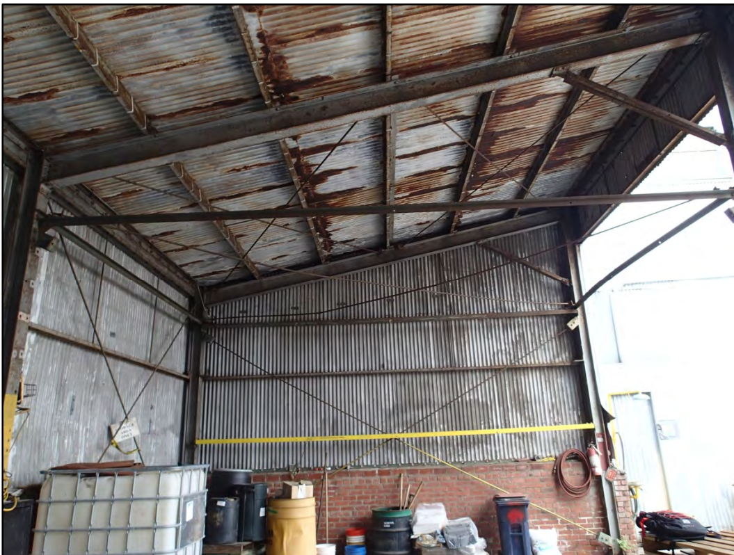
Figure 120-7 – View of the typical loose steel braces in Building 120.
