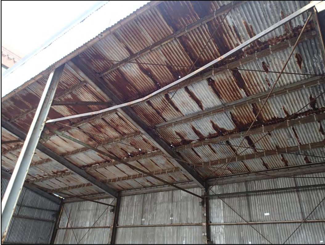
Figure 120-4 – View of the typical interior roof corrosion in Building 120.
