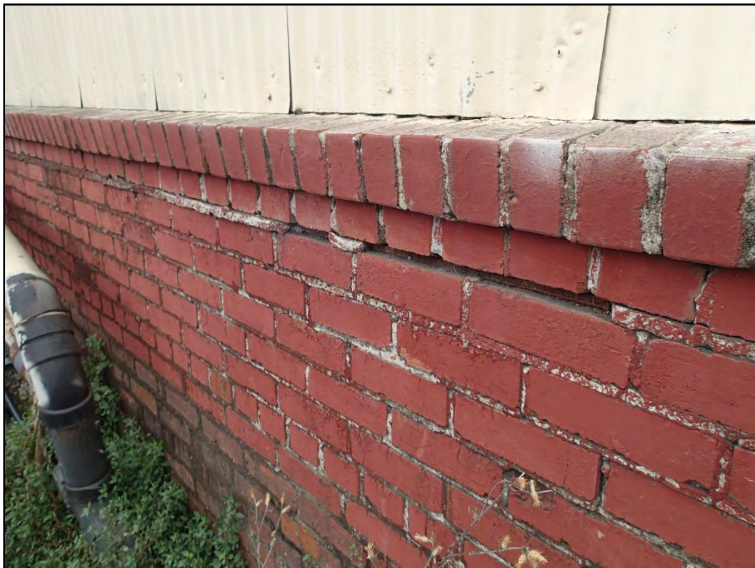
Figure 120-3 –View of deterioration in the exterior mortar joint at Building 120.
