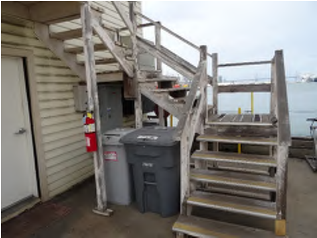
Figure 2 – Exterior stair damage
