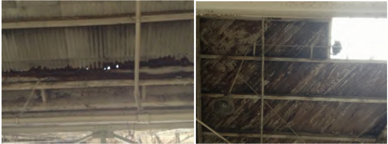
Fig. 1 - Building 108 metal roof from interior on left and wood roof from interior on right
