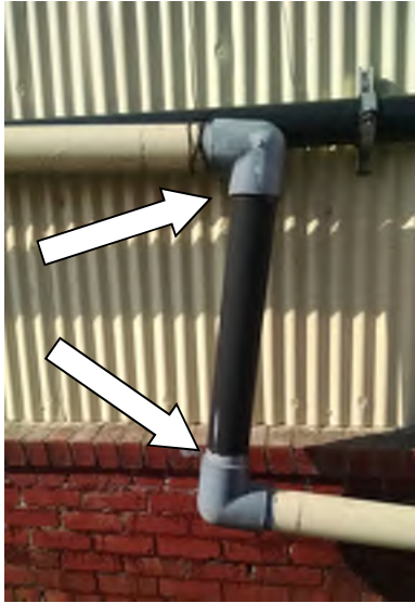
Figure 108-3 – Non-waste fitting on plumbing waste pipe.
