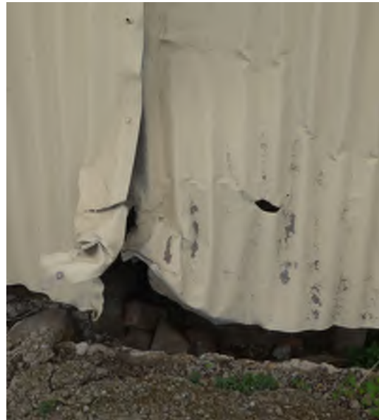
Figure 12 - Impact damage to CMP at grade, west elevation.
