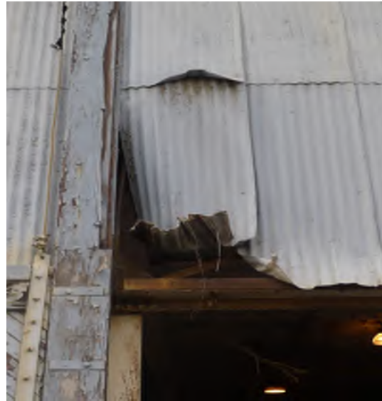
Figure 10 - Impact damage to CMP, west elevation
