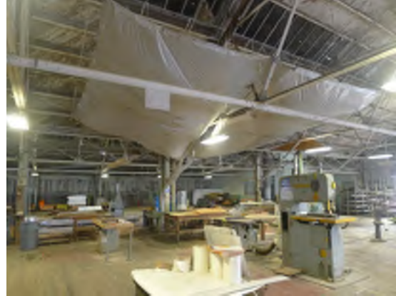
Figure 37 - BAE staff built roof leak containment.
