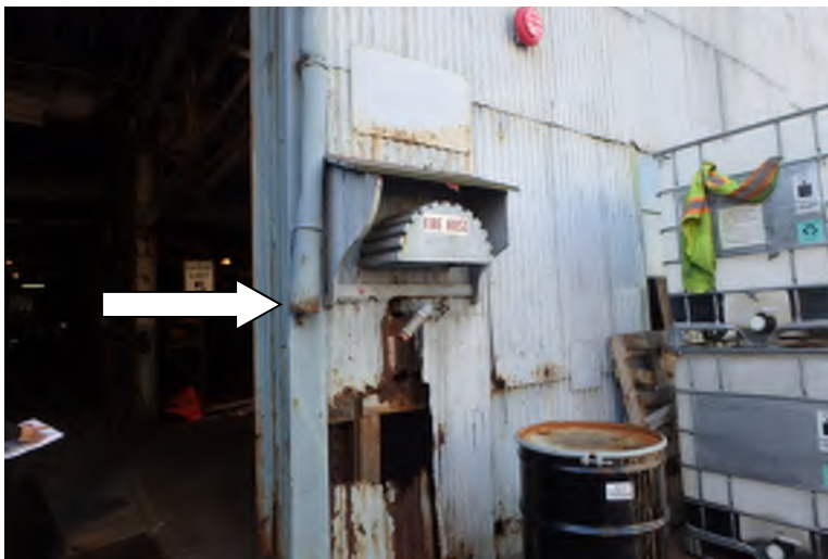
Figure 108-2 – Broken Rainwater Leader.
