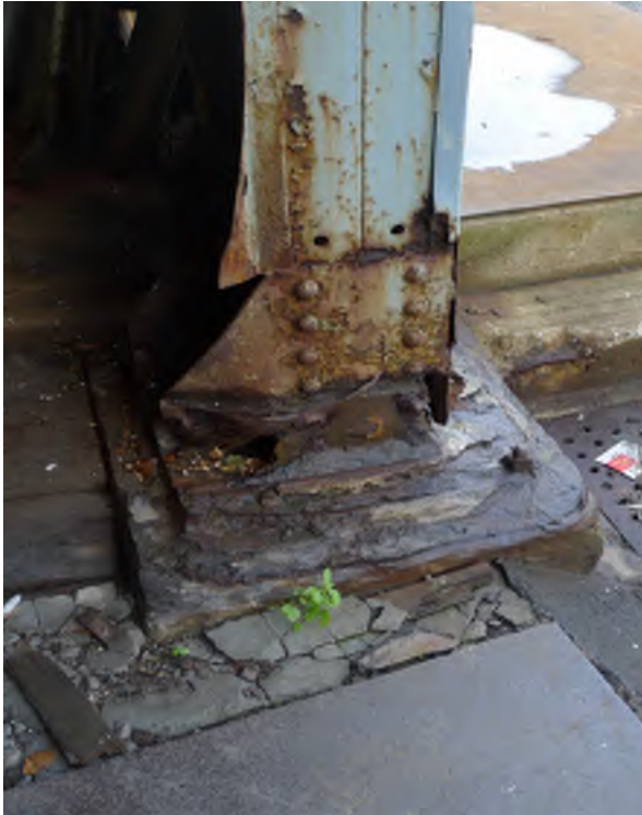
Figure 42 – Deteriorated structural column base, north elevation.
