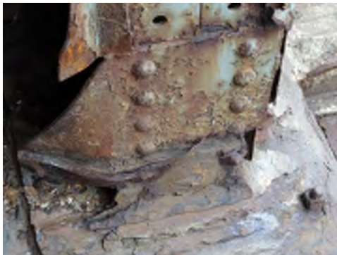
Figure 1 – Typical base plate and column damage
