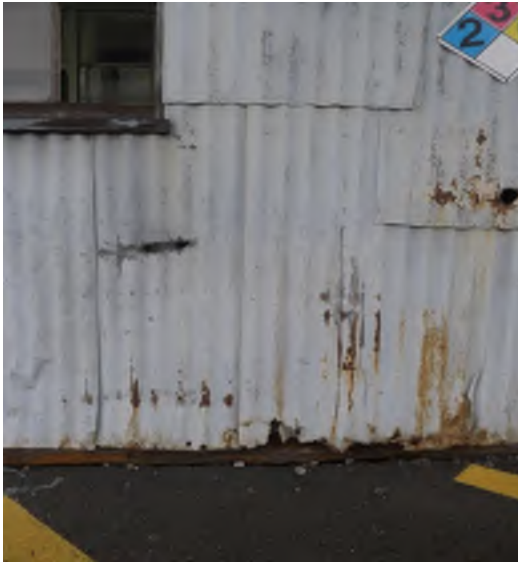
Figure 9 - Deteriorated CMP at grade
