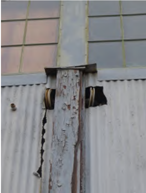
Figure 20 – North elevation, electrical equipment
