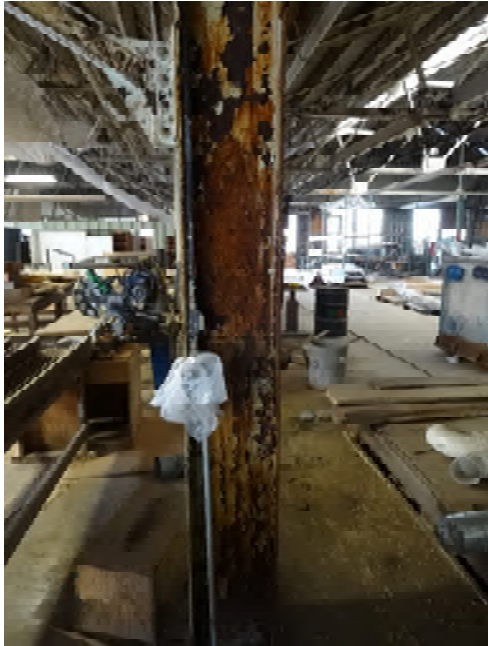
Figure 2 – Typical column corrosion
