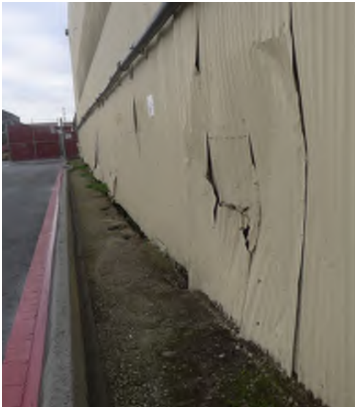
Figure 11 - Impact damage to CMP, east elevation.
