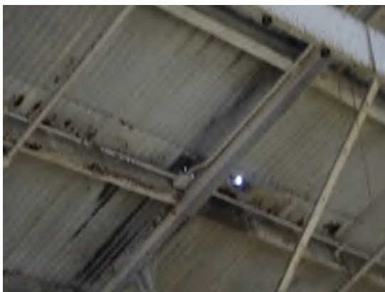
Figure 4 – Typical CMP roof damage
