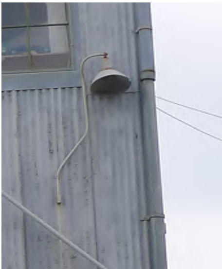
Figure 22 – North elevation, electrical equipment
