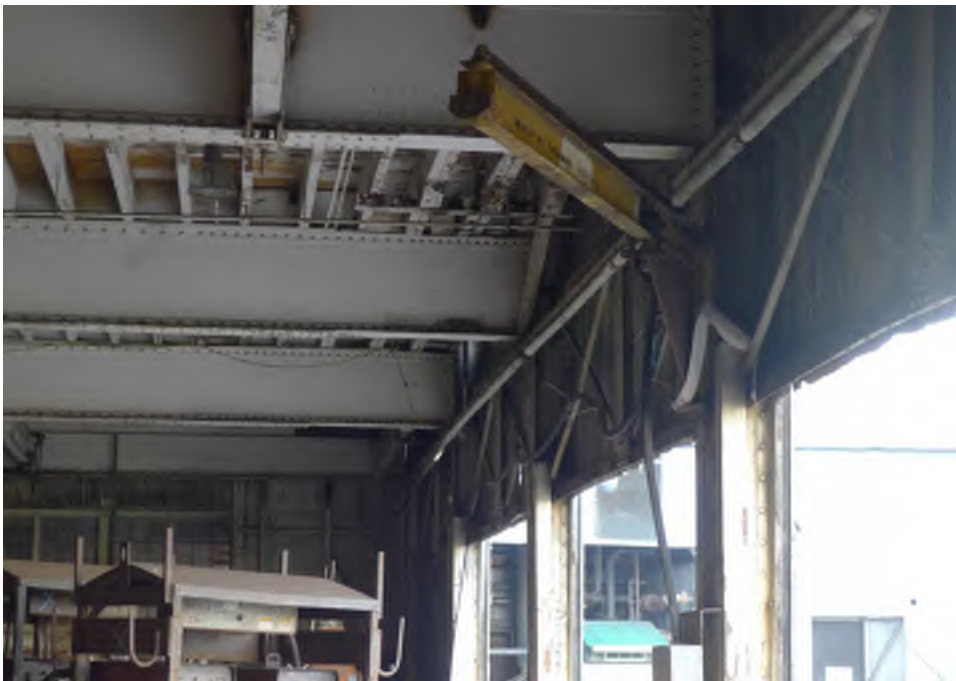
Figure 41 - Built-up steel beams in the west side at loading doors, looking south.
