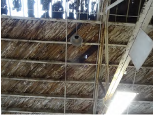
Figure 5 – Typical wood roof damage
