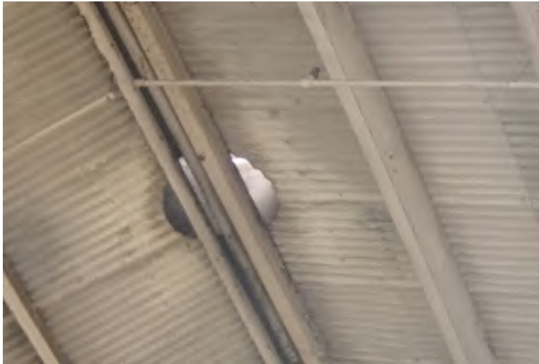
Figure 108-1 – Gravity Vents in ceiling.
