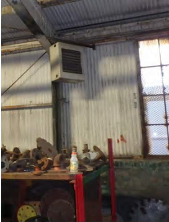
Figure 107-3 – Unit Heater without Gas Connection
