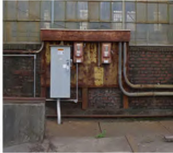
Figure 18 – North elevation, electrical equipment
