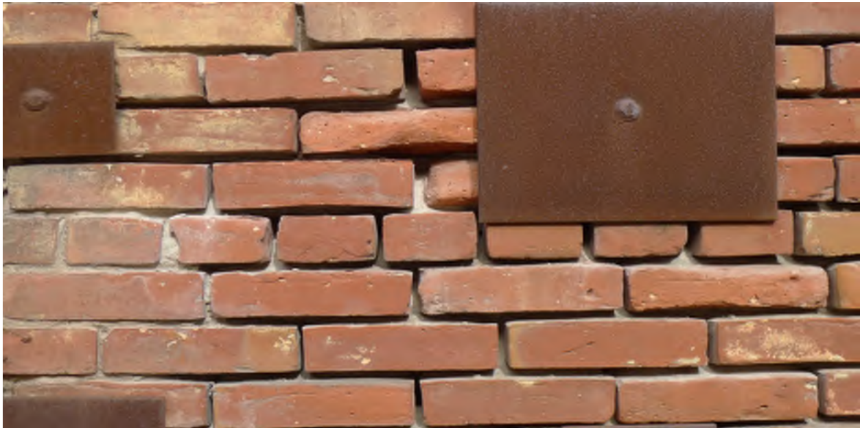
Figure 12 - South wall, deteriorated mortar from water intrusion. Reinforcing plates installed at an unknown date.
