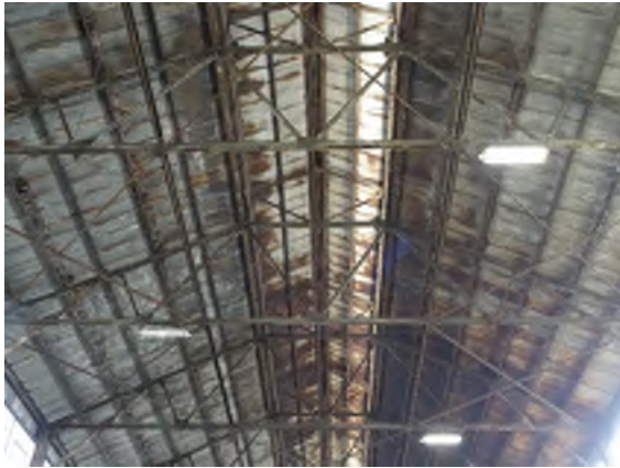
Figure 1 – Typical roof framing and CMP corrosion
