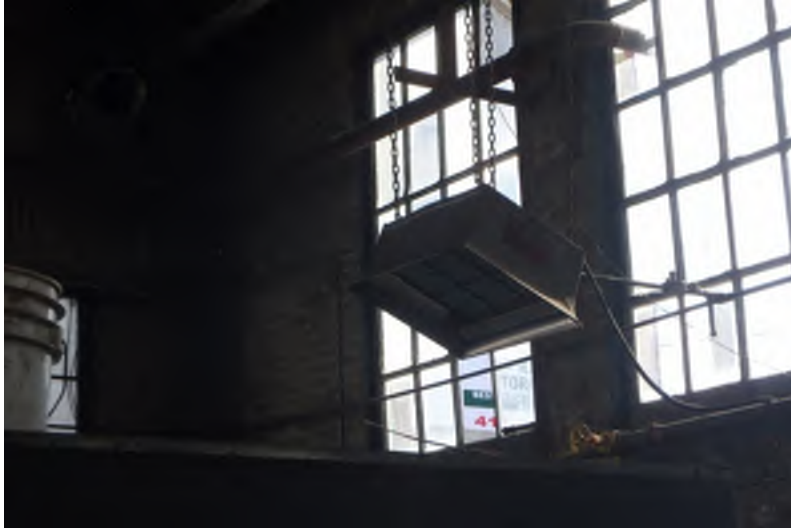
Figure 105-1 – Gas Radiant Heaters
