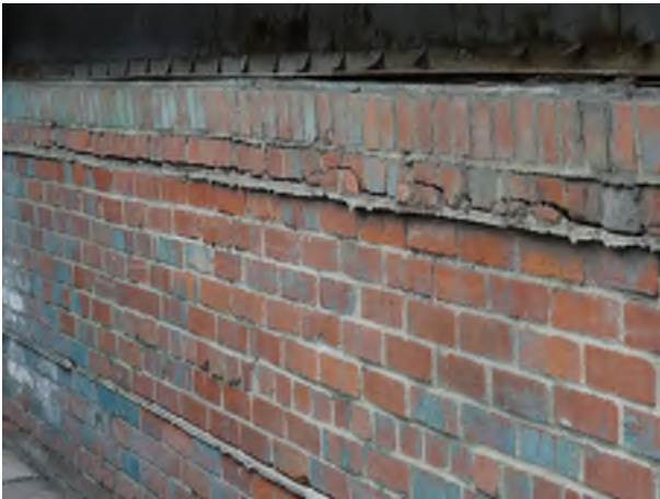
Figure 3 – Partial height masonry wall damage
