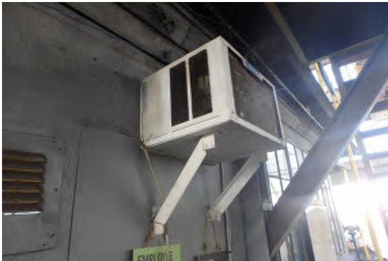
Figure 105-2 – Window-Mounted DX Cooling at Office
