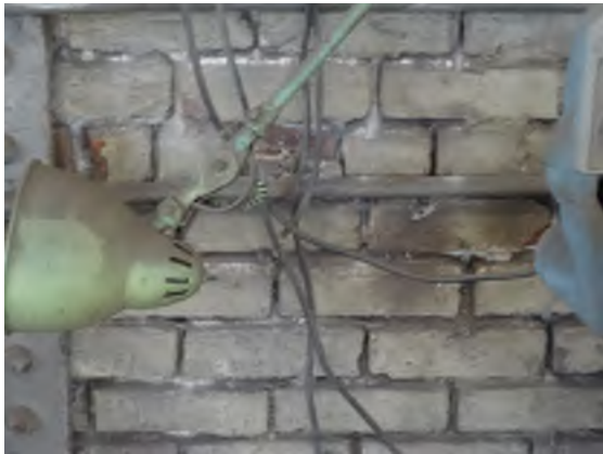
Figure 2 – Typical full height wall masonry damage
