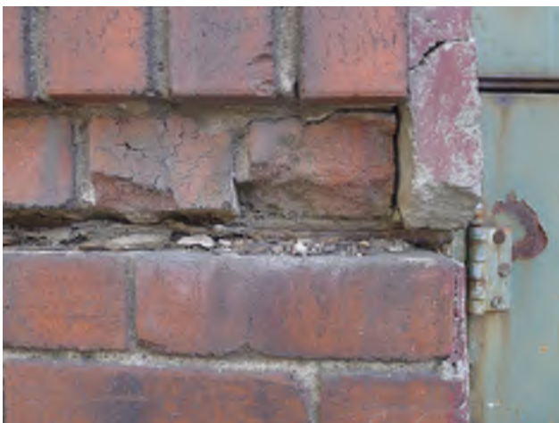
Figure 6 - Building. 103: Brick spall/crack at fire door. Note exposed rebar below header course.
