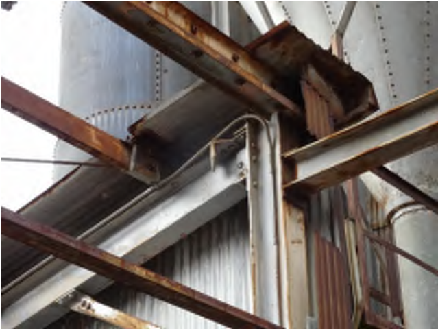
Figure 6 – Typical corrosion to steel framing members in open area
