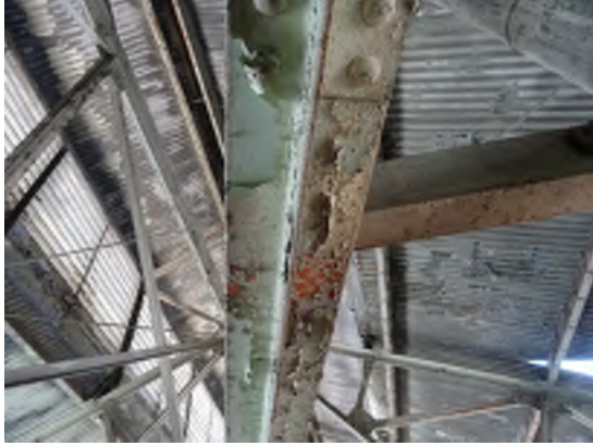
Figure 2 – Typical corrosion on steel framing and CMP
