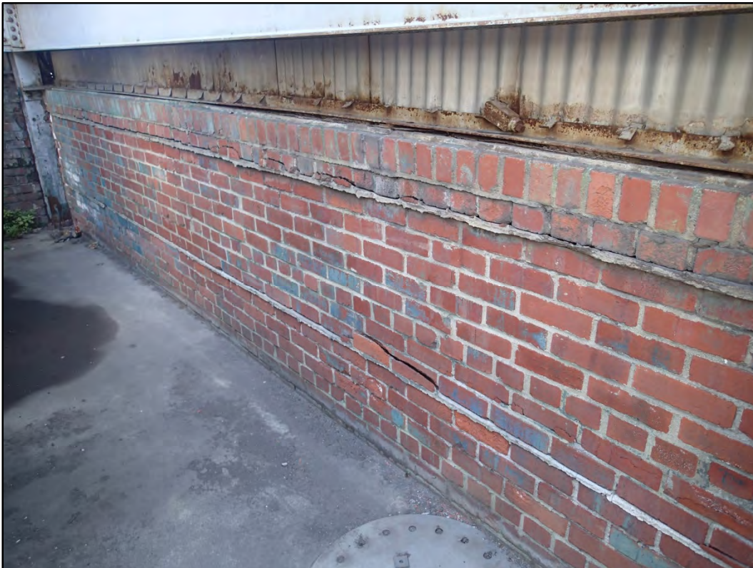
Figure 107-3 - View of Building 107 typical exterior brick mortar joint deterioration.
