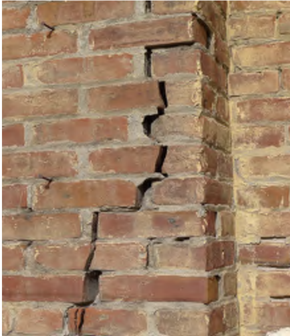
Figure 10 - South wall, cracking at pilasters.
