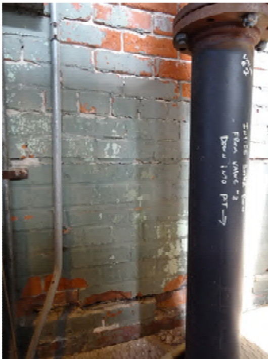
Figure 1 – Partial height masonry wall damage
