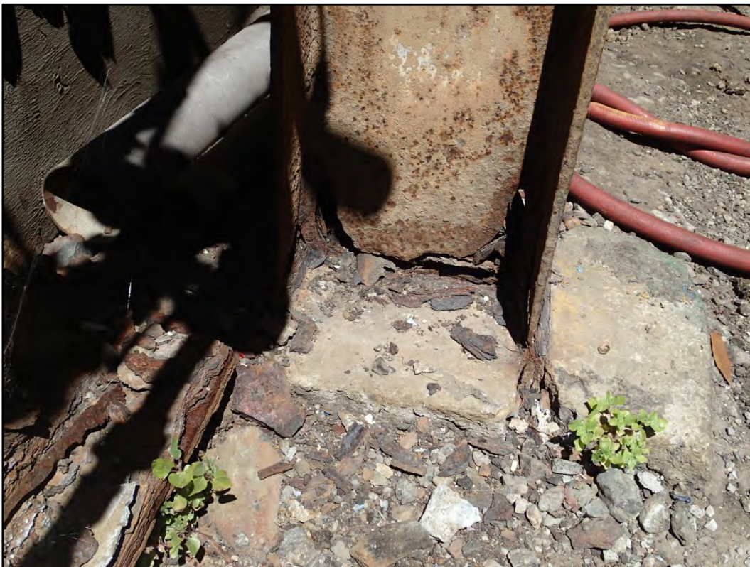
Figure 107-7 – View of the heavily corroded column base at north side of Building 107.
