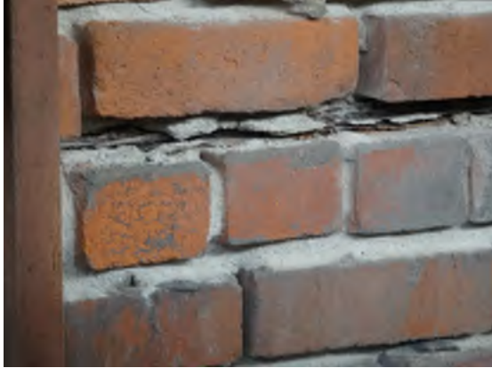
Figure 3 – Typical partial height wall masonry damage
