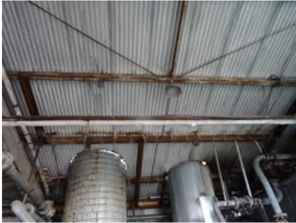
Figure 1 – CMP corrosion at cooling units
