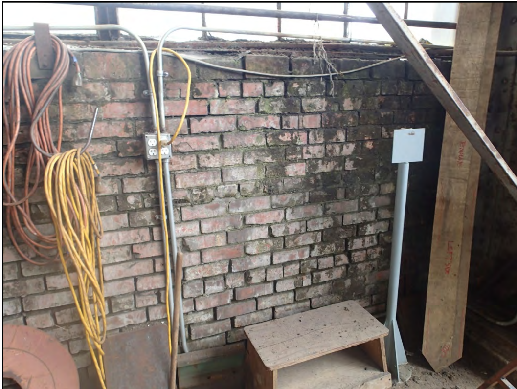
Figure 105-7 – View of the typical Building 105 deteriorated interior brick mortar joints.
