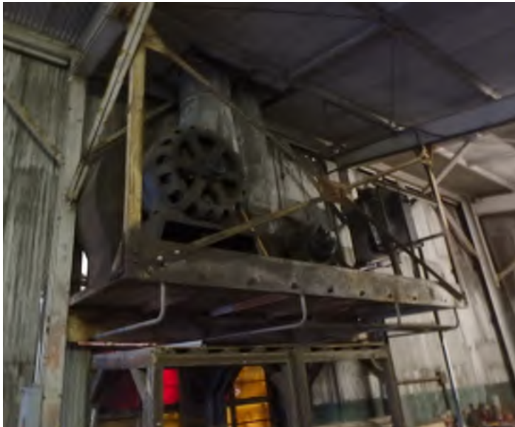
Figure 107-2 – Utility Fans Serving Woodshop
