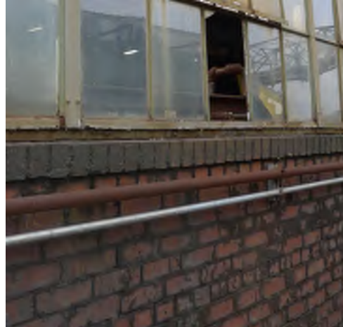
Figure 14 – North wall, joint sealant failure
