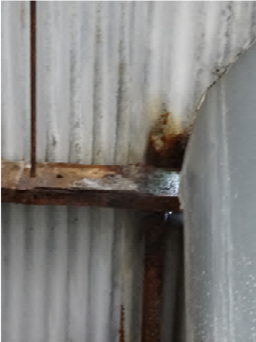
Figure 2 – CMP and purlin corrosion at cooling units
