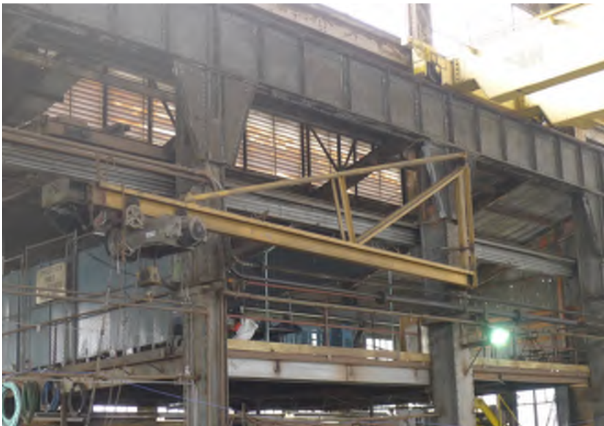
Figure 35 – Main shed, swinging arm crane.
