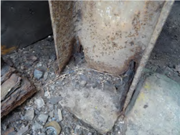
Figure 4 – Column damage at north end
