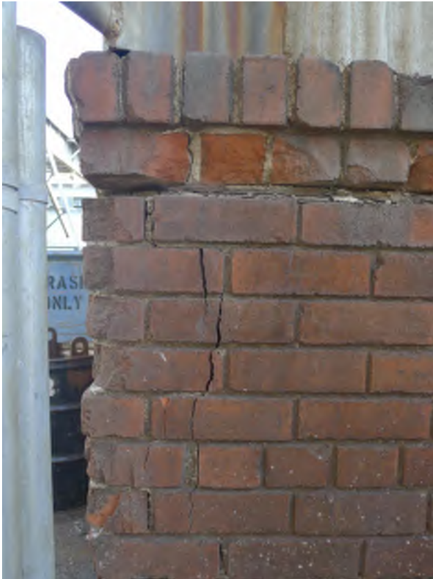
Figure 5 - Building. 103: Brick crack at NW corner.
