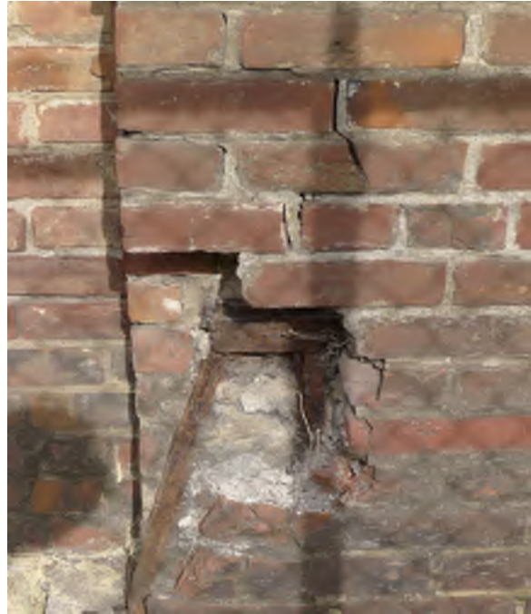
Figure 11 - South wall, displaced masonry at column base.
