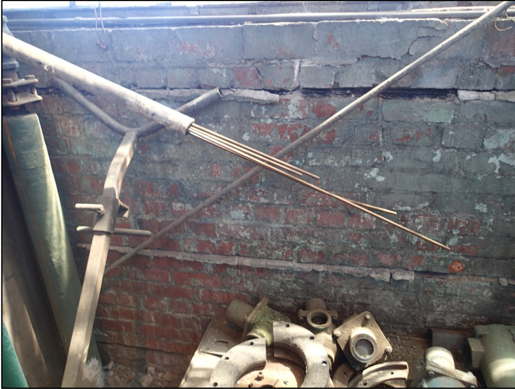
Figure 103-7 – View of the typical Building 103 deteriorated interior brick mortar joints.
