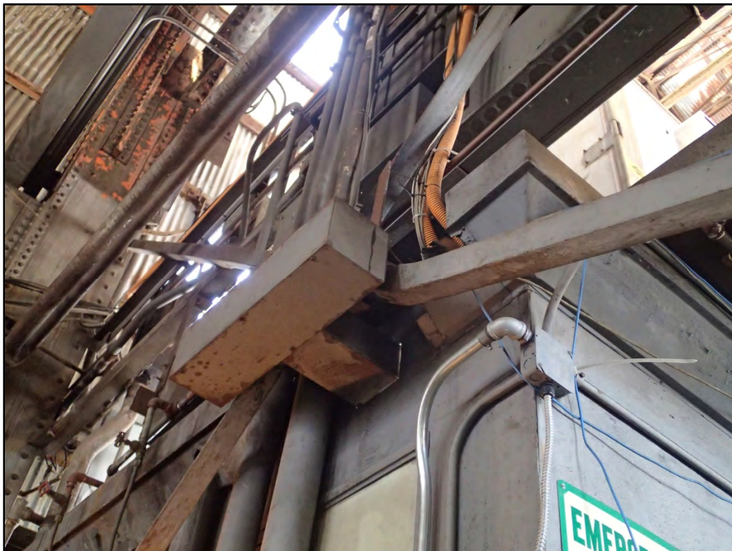
Figure 105-11 – View of the remaining bent braced frame at the west end of Building 105.
