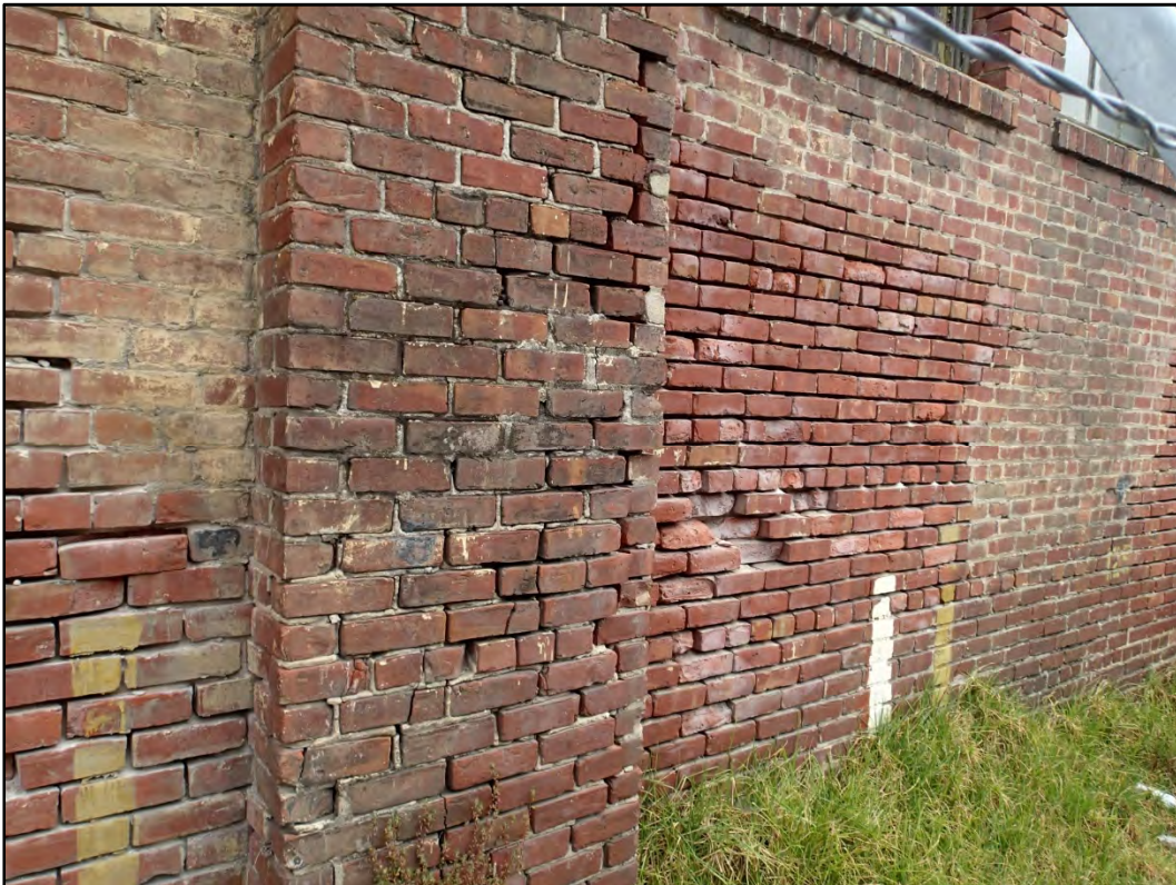
Figure 105-5 - View of Building 105 typical exterior brick mortar joint deterioration.
