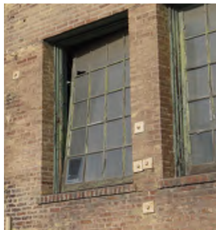
Figure 16 –South wall, hopper operation
