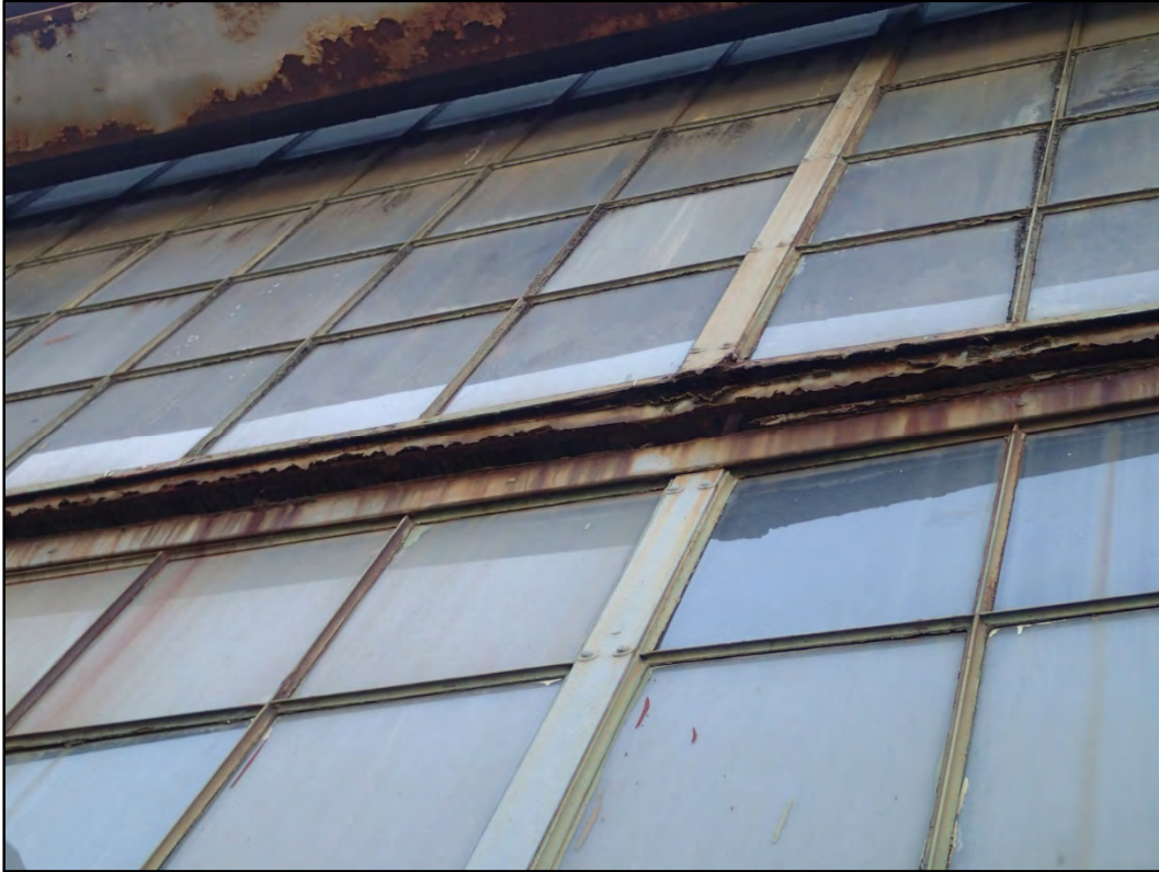
Figure 105-4 –View of the top row of windows that is bulging out towards the exterior.
