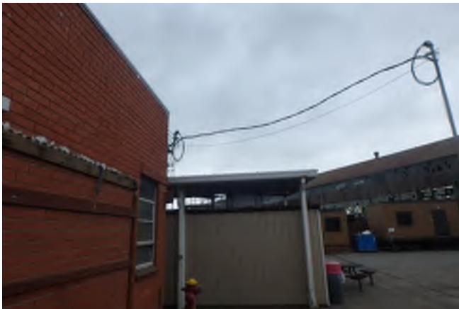
Figure 68-4 – Overhead Power to Temporary Structure
