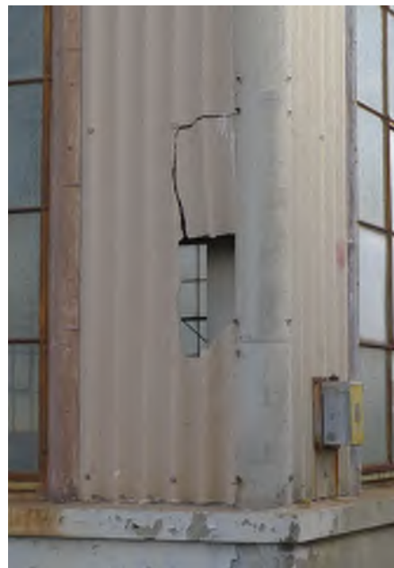
Figure 4 – Southwest corner, CTP damage
