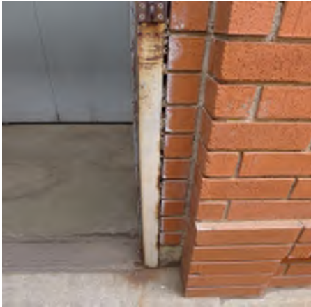
Figure 11 - Sealant failure in door frames
