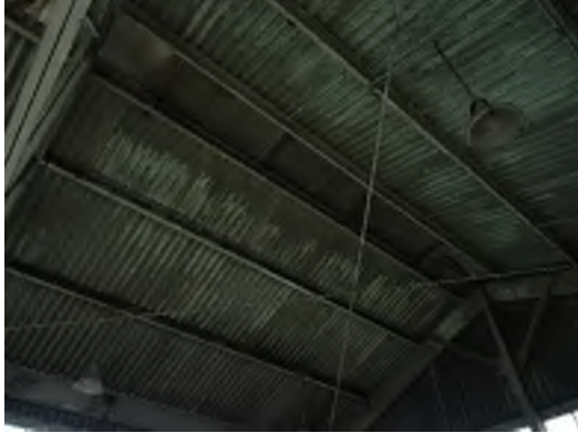
Figure 3 – Building 58 CMP degradation
