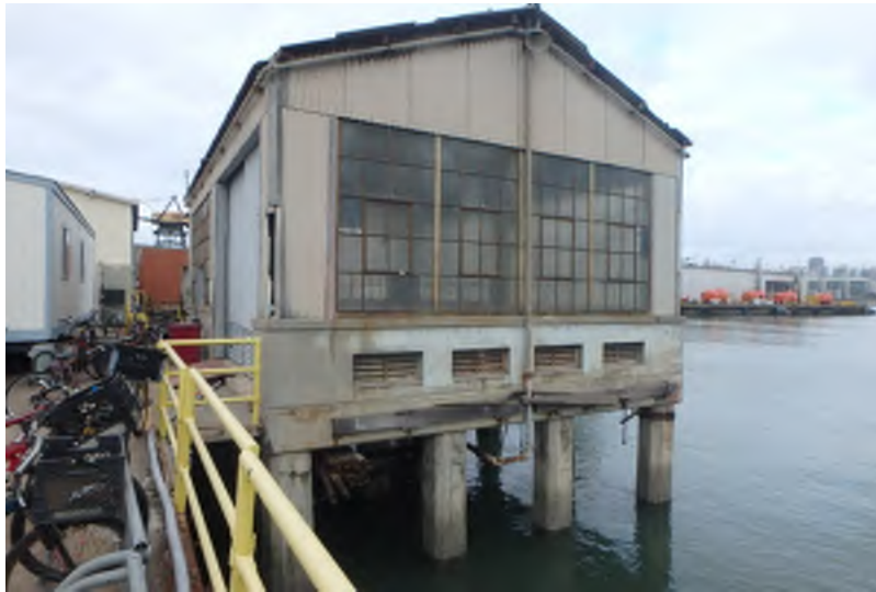
Figure 58-1 – Building Exterior Wall Louvers
