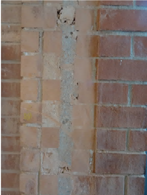
Figure 2 – Cut masonry partition wall with exposed rebar
