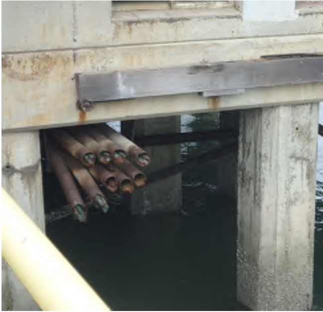
Figure 58-3 – Abandoned Conduit beneath Building
