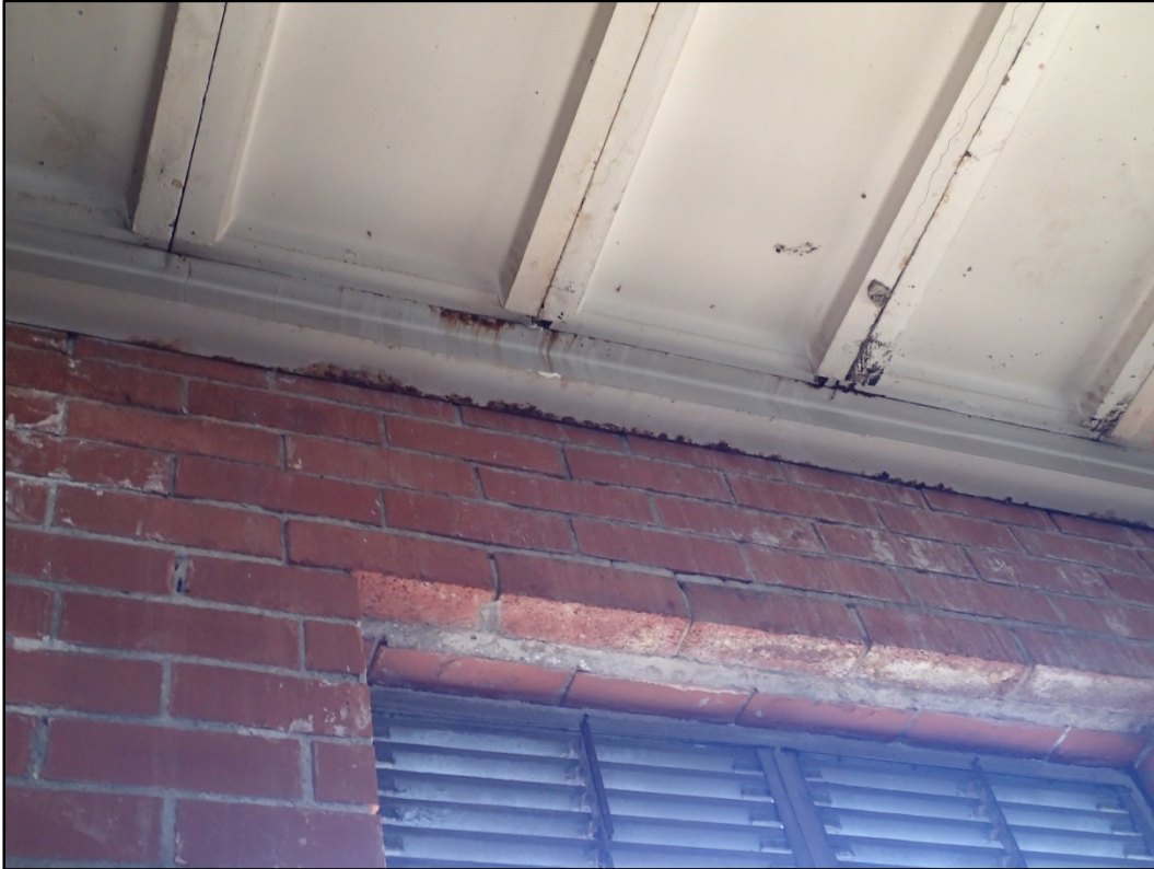
Figure 68-7 – View of localized minor surface corrosion on the ledger along Building 68 south wall.
