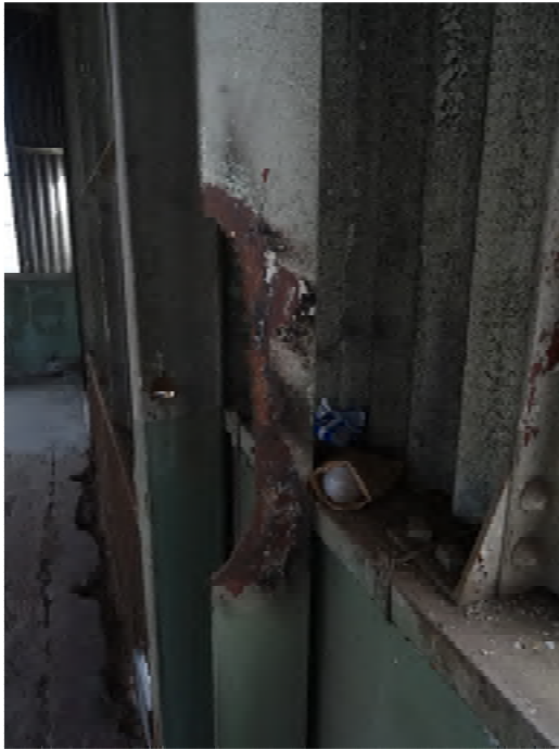
Figure 1 – Building 58 column damage
