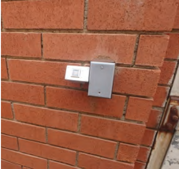
Figure 68-3 – Exterior Lighting Photosensor
