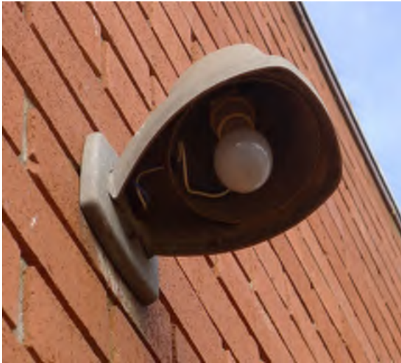
Figure 14 - Exterior light fixture
