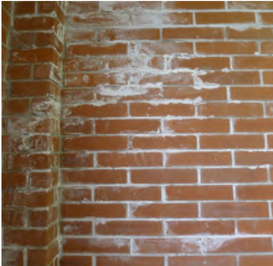
Figure. 16 - Interior efflorescence on brick
