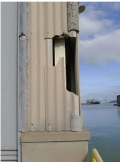
Figure 3 – Southeast corner, CTP damage
