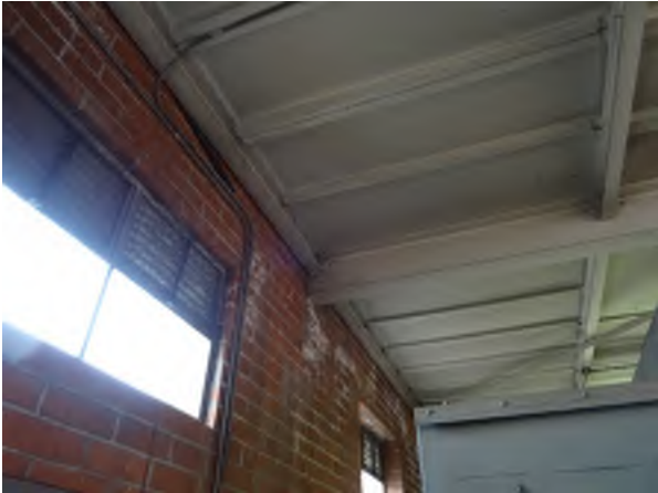
Figure 1 – Concrete precast panels with minor cracking
