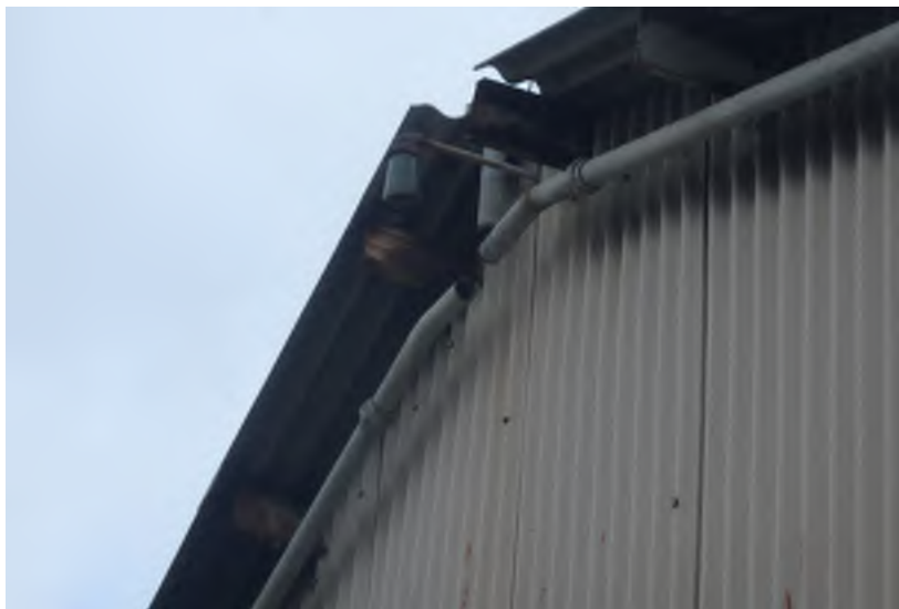
Figure 58-2 – Broken Fire Sprinkler Pipe
