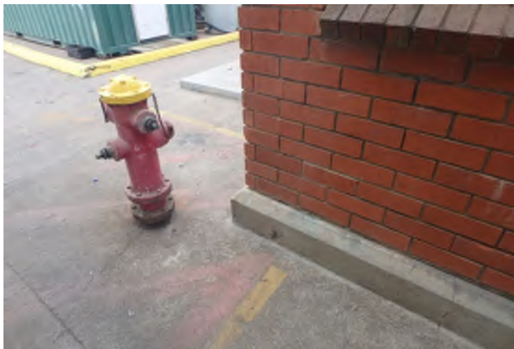
Figure 68-2 – Fire Hydrant at SW Corner
