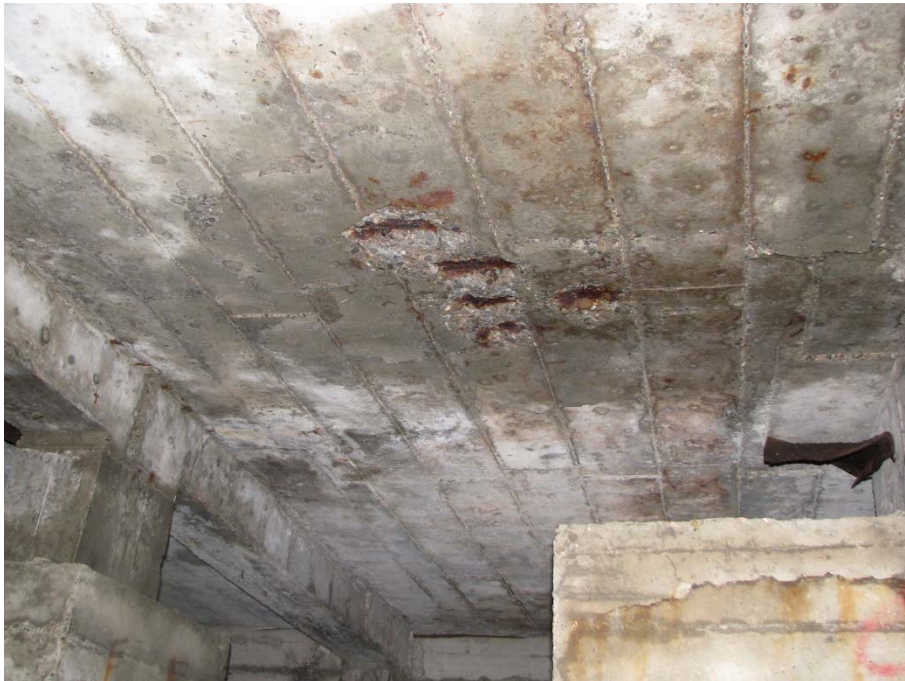
Figure 4 Photo showing typical soffit spall damage with corroded rebar between bents 45-46 row A
