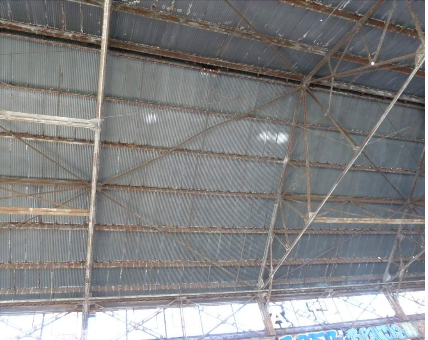
IMAGE 11: Buckled Roof Tie
