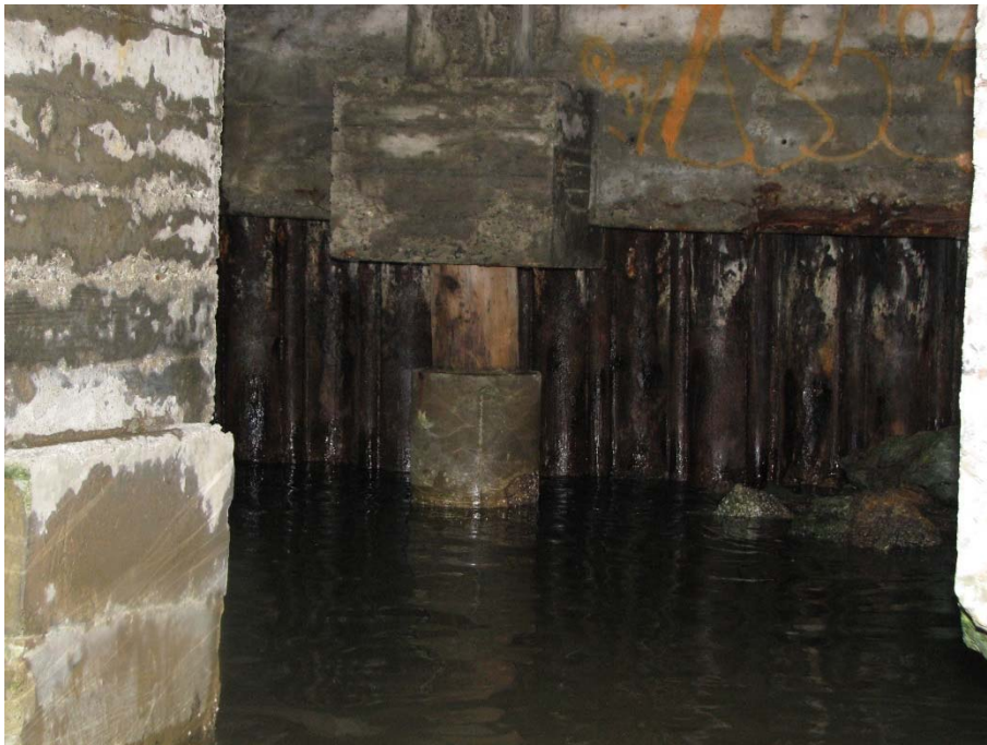
Figure 5 Steel sheet pile at row BB with timber pile at bent 45 row AA shown in front.
