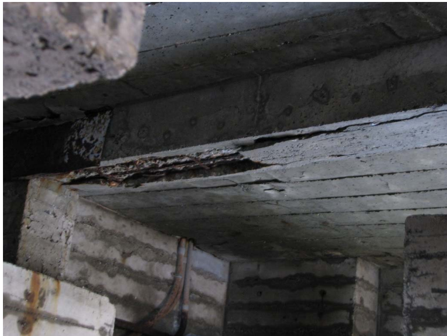
Figure 3 Photo showing spall damage with corroded rebar to cap beam at row 51 A-B
