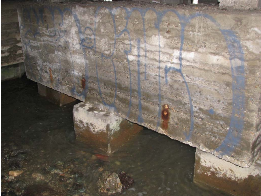
Figure 6 Bents 35-35.5 36 row A. Assumed piles encased in concrete and joined with a cap beam.
