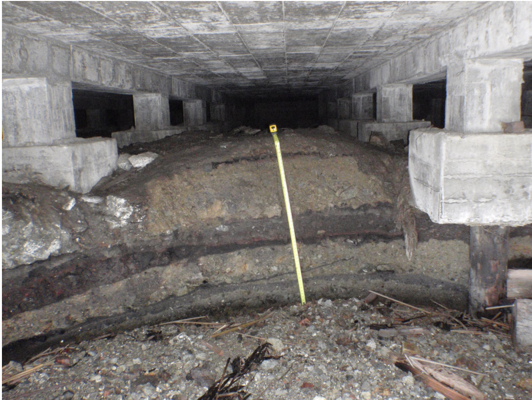
Photo 2 – Exposed Fill Soils under Building 6 at Rows 15 and 16
