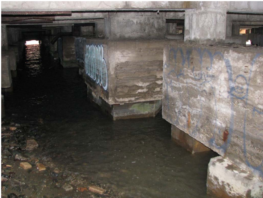
Figure 7 Large concrete encasements at row A located at all bents with four-pile clusters at row I. It is assumed that there are four piles in these encasements to match the outside row, but these were not visible.
