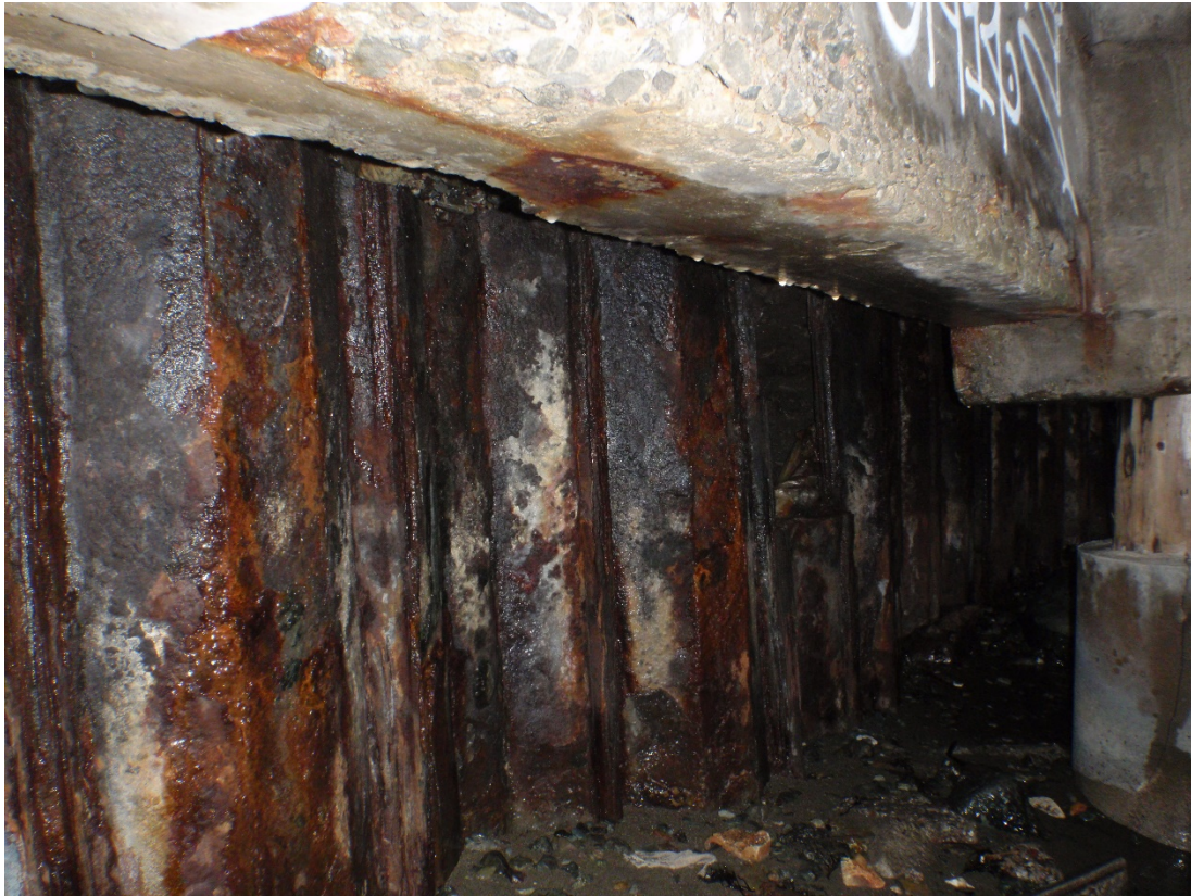
Photo 3 – Corroded Sheet Pile Wall under Building 6 at Row BB, Row 38
