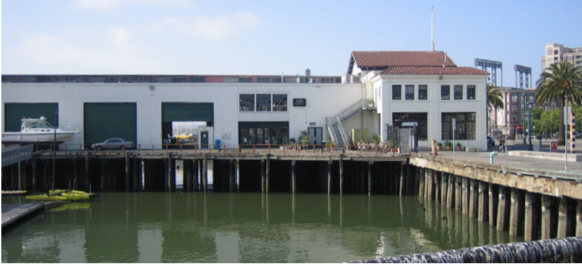
Efforts are underway to rehabilitate and reopen the Pier 38 bulkhead building which had been closed (along with the pier shed) due to safety and code compliance violations.
